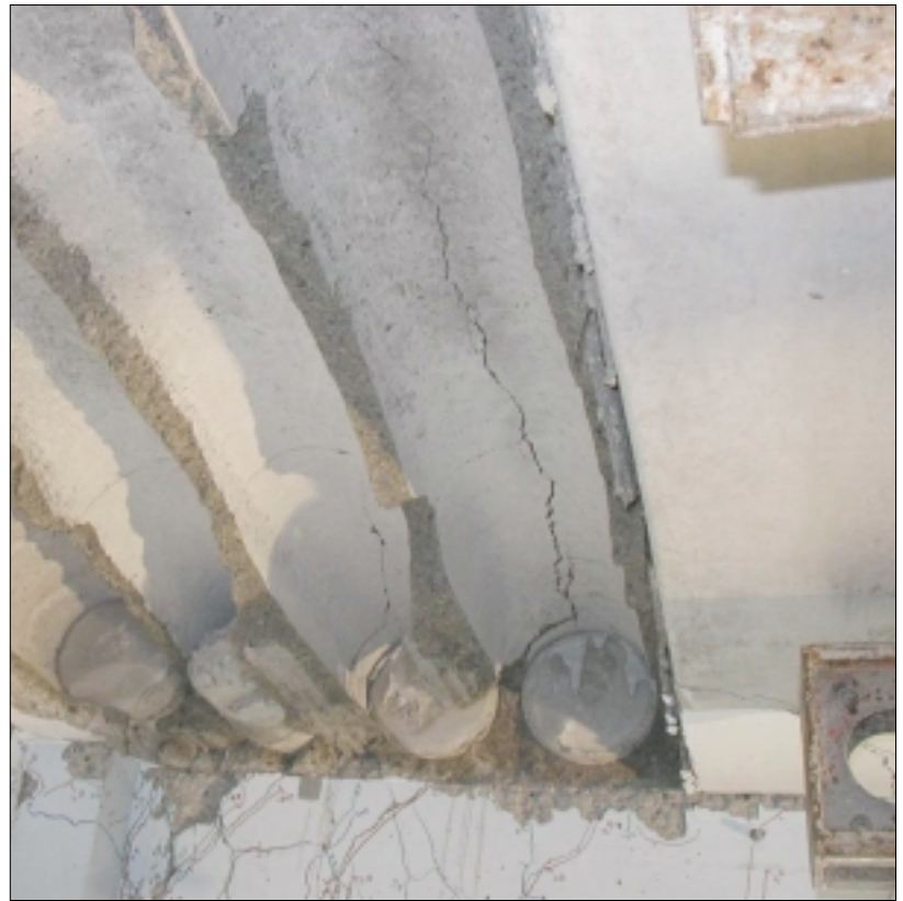
Fig 2. View of the Southwest corner after the lower portion of the southernmost hollowcore unit had fallen off. The adjacent hollowcore unit is still intact.
