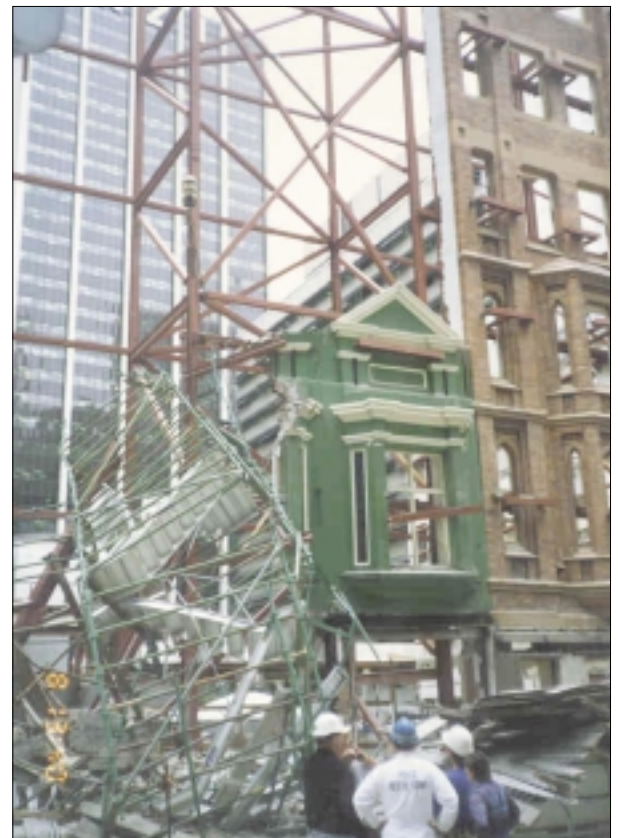
Below: a rare collapse of a heritage façade in Sydney, Australia in 1990. There were, fortunately, few injuries and no fatalities
