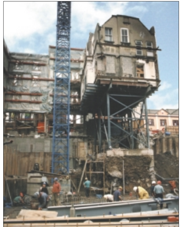
Above: A dramatic example: retention of second and third floors of 5, Duke Street, Marks & Spencer, Grafton Street, Dublin
