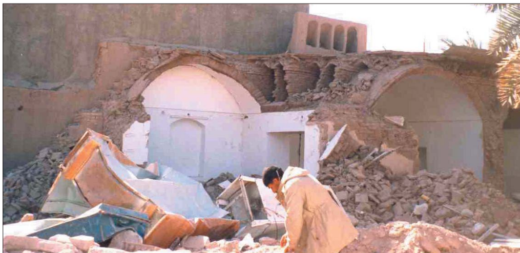
Fig 3. Non-engineered mud brick arch structure after the Bam, Iran earthquake
