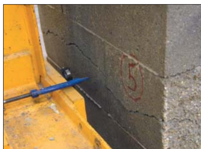
Fig 4. Failure of a B-wallete indicating thin joint is stronger than solid dense concrete blocks
