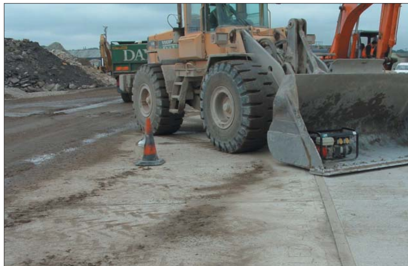
Fig 5. Full scale construction using recycled aggregates for heavy duty concrete pavement application
