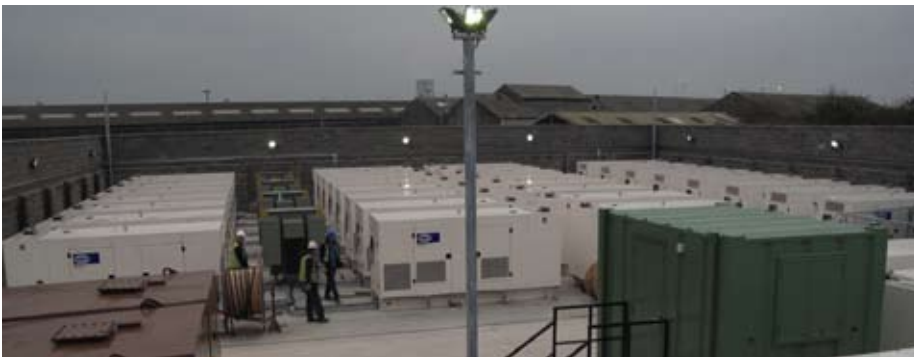
Figure 12 Power generators supplying the National Grid at Green Frog Power
