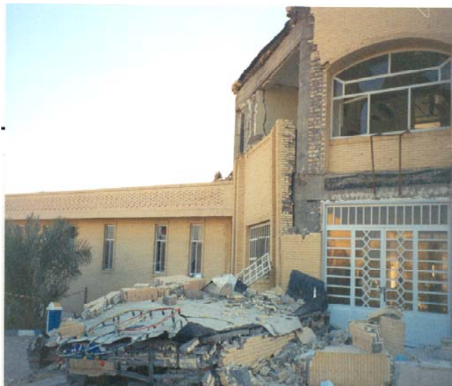
Photograph 24: The reinforced concrete structure of the main building of Aflatoni hospital survived, however, the extended canopy structure of the jack arch on brick walls collapsed due to wall failure
