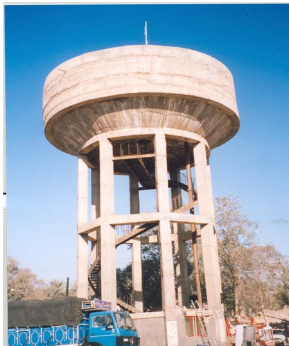
Photograph 20: The main reinforced concrete water tower in the centre of Old Bam, in the fire station. Survived with shear cracks in the beam at column beam connection (9EMS)
