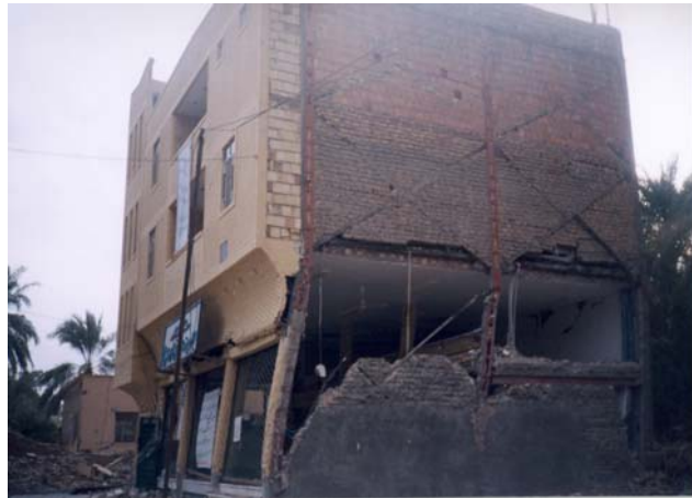
Photograph 33: Ground floor level shop with high floor to ceiling and no internal cross walls. The steel frame cross bracing at ground floor level is missing at the rear, batten column buckle about its hollow axis resulting in soft storey structural damage. (photo by: H. Darejati)
