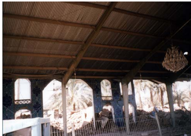
Photograph 6: Rafter stays (bracings) between the rafters at eave level and purlins and cable diagonal bracing between columns at every other bay provided sufficient stiffness to stop longitudinal collapse of this mosque hall.
