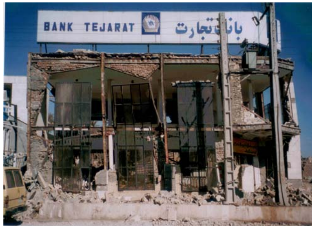
Photograph 18: Southern view of Bank Tejarat with irregular and bracings.
