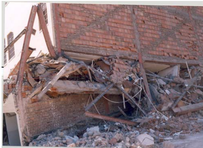
Photograph 12: Northern elevation view of the above building showing deformations were concentrated on column heads at second floor car park area ( 9 EMS). The corner columns are single UB and intermediate columns are back to back welded channels with no buckling stiffness, poorly welded weak diagonal bracing made of 80mm channels or T18 bars in East-West direction had no resistance towards lateral loading.
