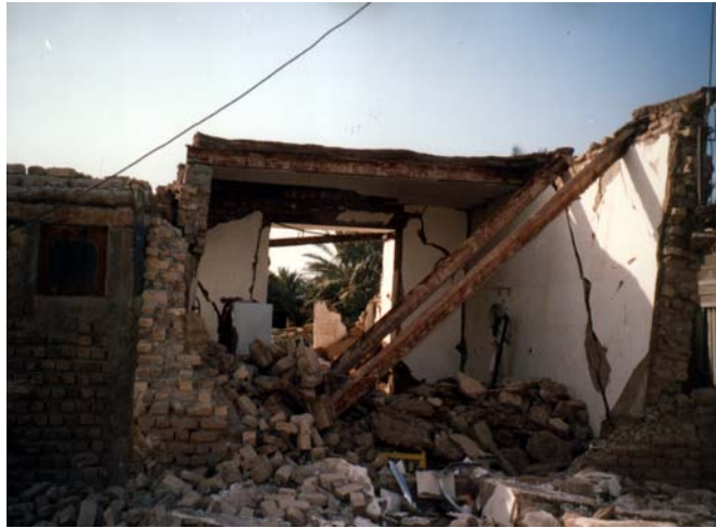
Photograph 7: Lateral movement in the wall resulted in the jack arch beams losing their bearing and collapse
