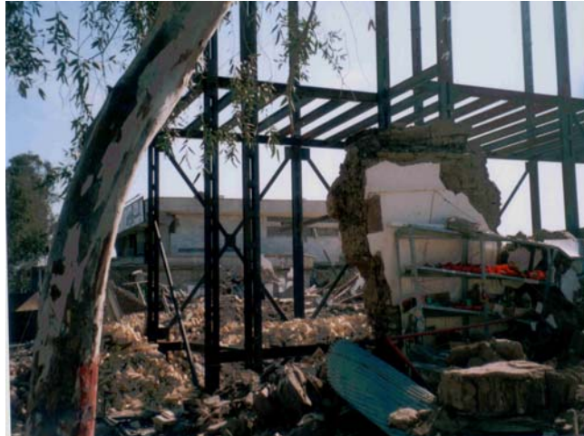
Photograph 10: Steel structure frame of batten columns, Khorgini beams and connections supporting jack arch beams. Gausset plates at bracing connection cannot be welded to the centre of flange of Khorgini beams because the beam is supported on the side of the column resulting in weak bracing
