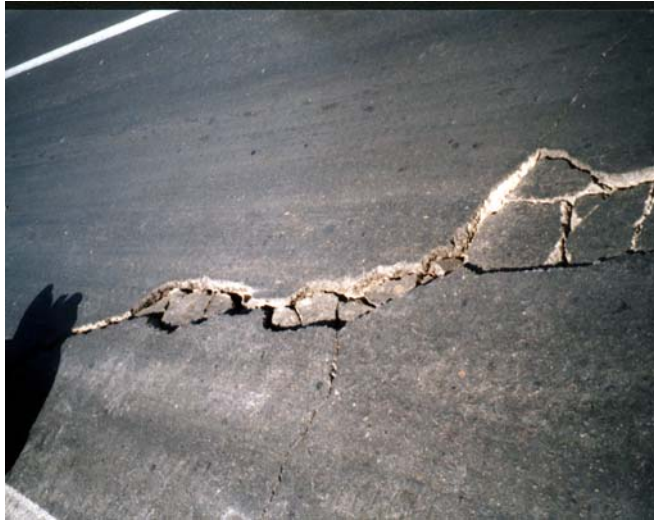
Photograph 1: Surface cracks 50mm wide appeared near the fault on the main roads close to Baravat
