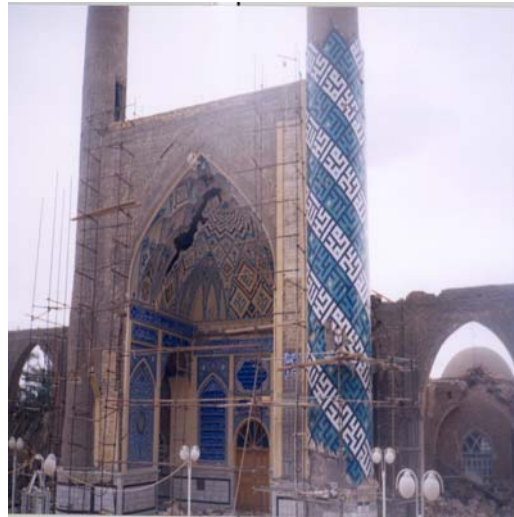
Photograph 5: This mosque with minarets about 20m tall and vault of 7m span wide 13m tall survived with damage to the false ceiling plaster and structural damage to the minaret with no tiles (Photo by: H. Darejati)
