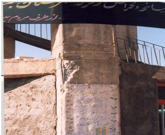
Photograph 22: Buckling of column reinforcement resulting from missing confinement traverse bars, Main reinforced concrete water tower in the centre of Old Bam. The earthquake intensity was 9 EMS
