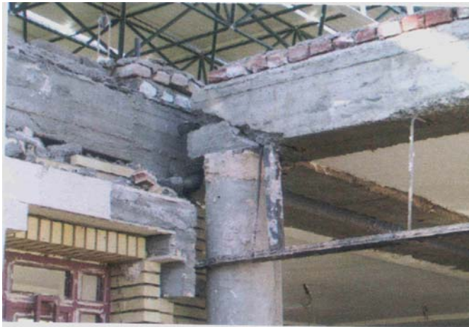
Photograph 23: Bam Railway terminal, failure of support due to insufficient bearing (extract from figure 13 taken by M.Moghtaderi-Zadeh, et al. Ref: 14 )
