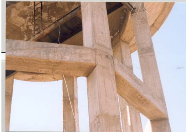
Photograph 21: Structural shear cracks in the beam at beam column connection, reinforced concrete water tower shown in Photograph 20
