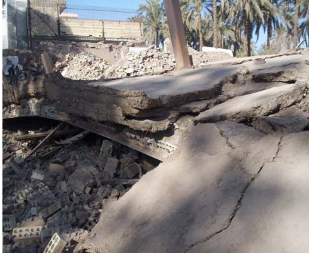
Photograph 9: Successive layers of mud straw on jack arch roof in combination with seismic load resulted in plastic hinges on top and bottom of the columns and collapse of the shop with 4m displacement towards west into the pavement area
