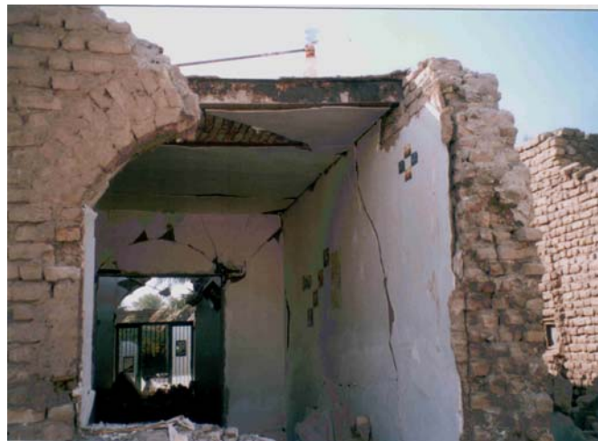
Photograph 8: Gypsum and clay and skim of plaster fell of the soffit of brick arch because of movement of flexible brick arch
