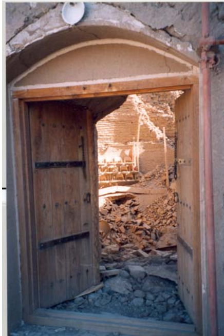
Photograph 29: The reconstructed part of the inner wall of the Ice House collapsed inward as the result of the additional weight of the recently reconstructed stepped dome
