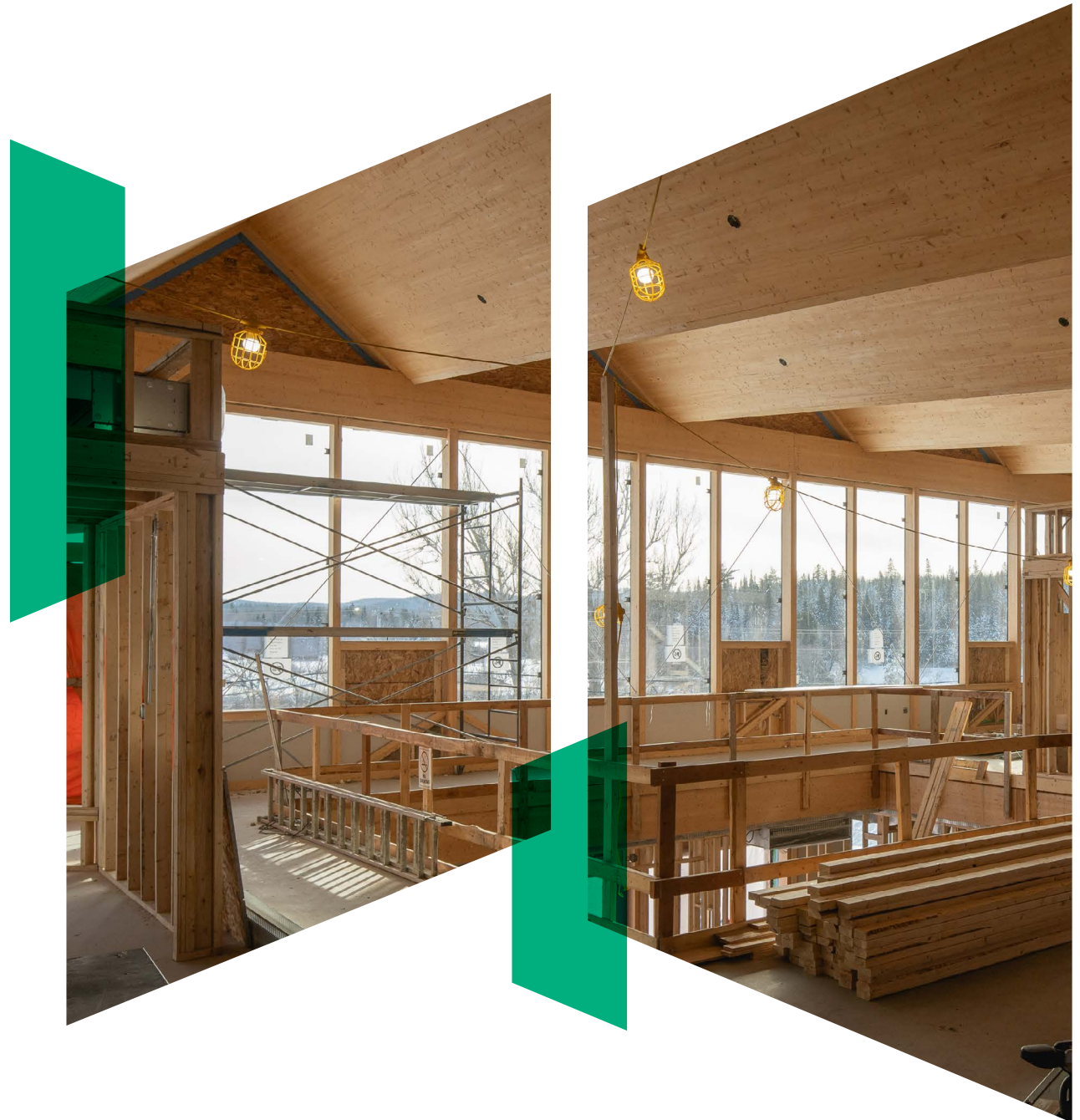
Image – La Pêche Town Hall during construction Structural Award winner for elegant detailing, and an intelligent and striking use of mass timber © Latéral, 2025
