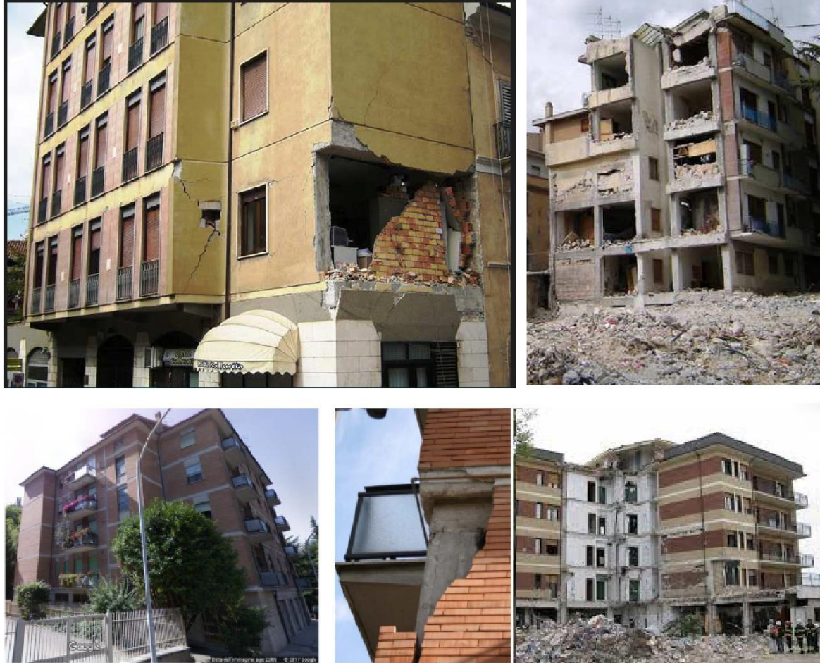
Figure 36: Typical RC buildings damaged during the L'Aquila earthquake, Italy. Masonry infills are visible within the RC frames.
