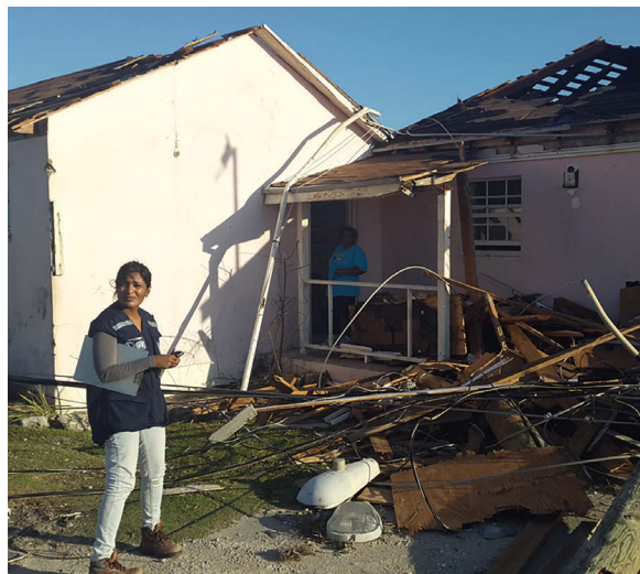
↑FIGURE 1: Disaster response opened new chapter in Jagnarine's career, assessing damaged structures such as after Hurricane Joaquin in Bahamas, 2015
