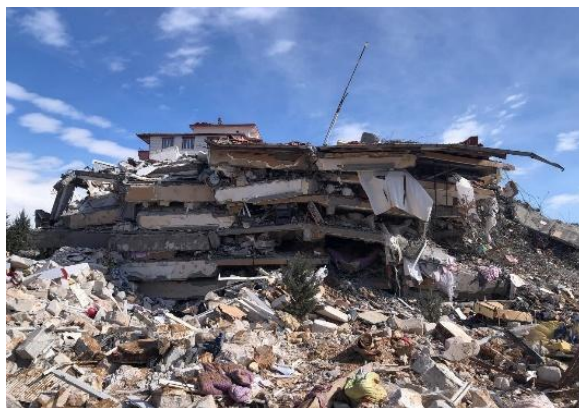
Figure 99: Total collapse and pancake (Besni/Adiyaman).
