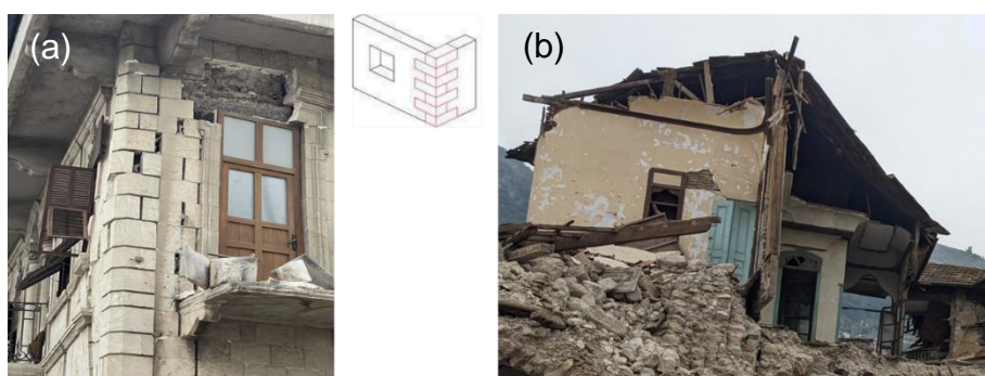
Figure 108: a) Corner failure due to the lack of connections in the quoin induce OOP of the facade, b) OOP failure of the gable.
