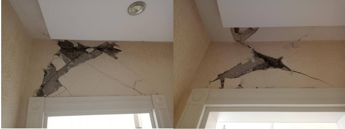
Figure 161: Coupling beam damage.
