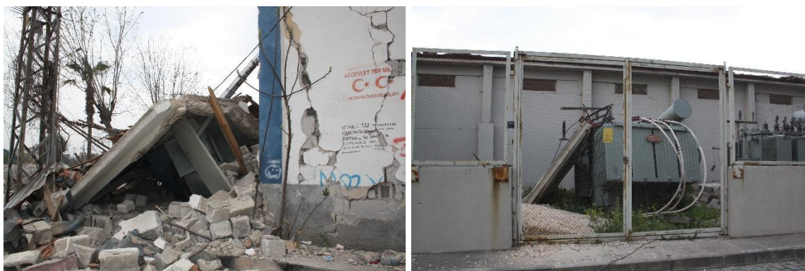
Figure 212: Heavily damaged Low- Medium Voltage transformers observed in Hatay on 17 th March.
