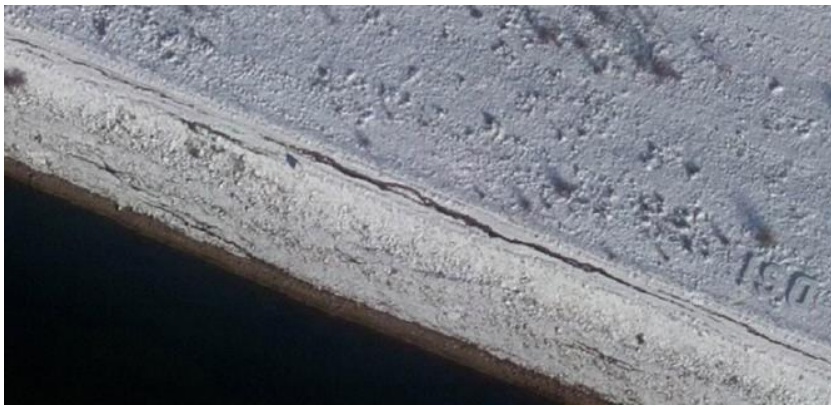
Figure 230: Visible Cracks in Crest – Sultansuyu Dam – Harita Genel Mudurlugu
