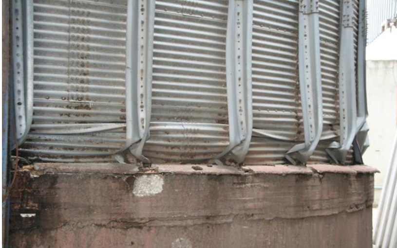
Figure 221: “Elephant foot” failure of silo wall and vertical stiffeners.
