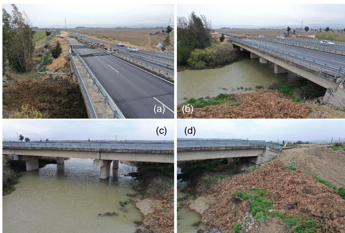
Figure 61: Lateral spreading-related damage of bridge in Demirköprü (36.245878, 36.357019). (a) damage of pavement to the east of bridge (b) View of the bridge from the west side (c) Rotation of piers and visible spreading of soil (d) Rotation of abutment due to spreading.
