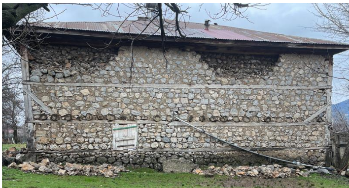
Figure 117: Localised arch failure.
