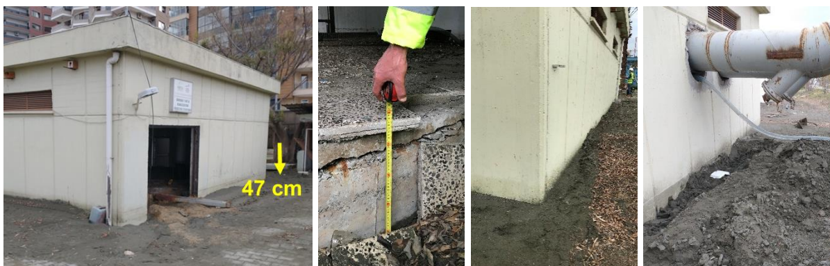
Figure 50: Liquefaction at a water management building close to the seafront (36.590891, 36.175676).
