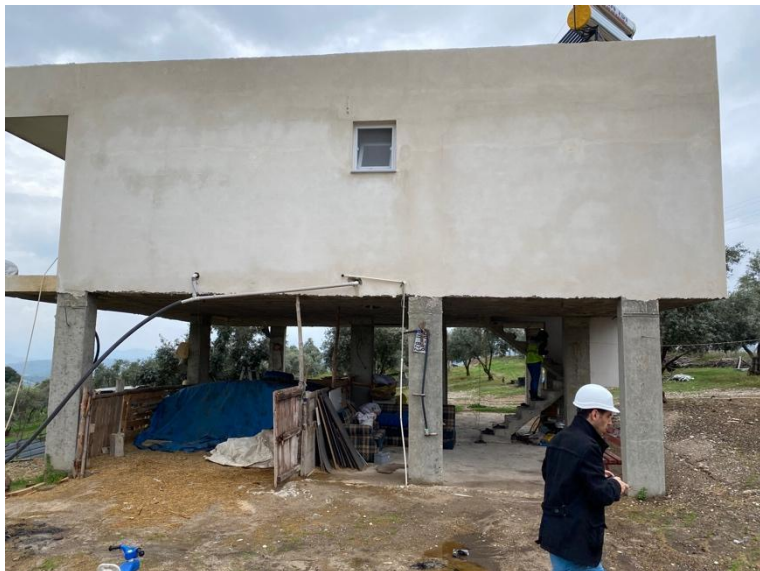
Figure 238: Reinforced concrete house in Kadirli Municipality (Source: EEFIT Team)
