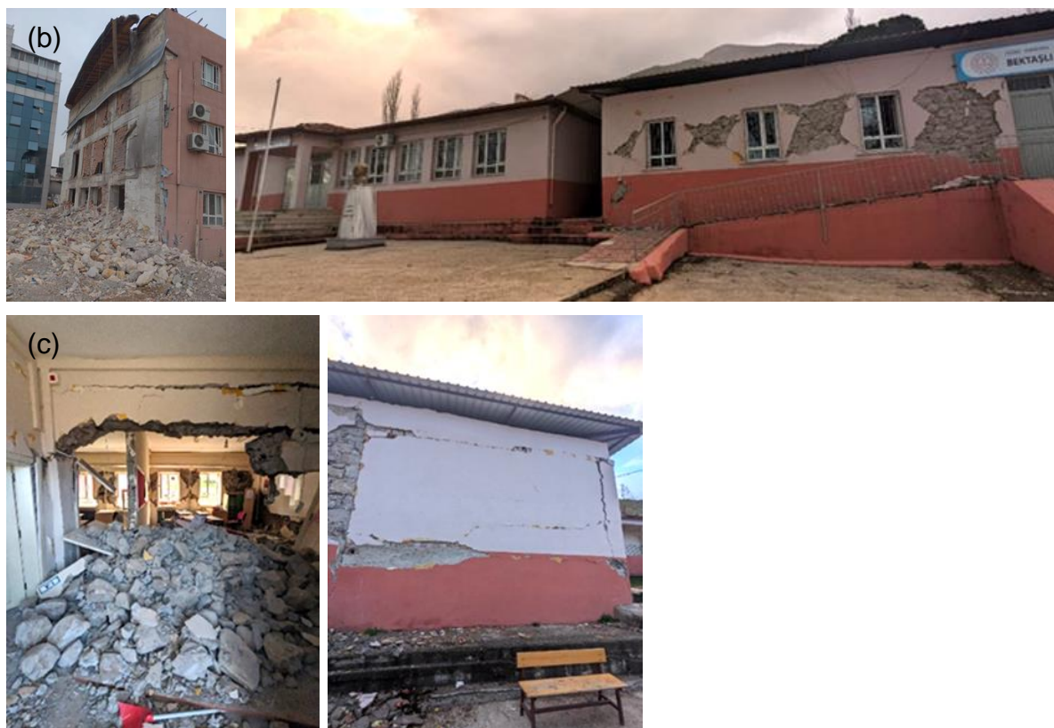
Figure 191: Schools observed to be severely damaged, collapsed or designated for demolition. a) Mithatpasa Ilkokulu, Iskenderun, Hatay– Top floor of one building in stone masonry collapsed, while the remaining buildings were not visibly damaged, b) Inonu Ortaokulu, Antakya, Hatay–RC building. Two other buildings in this compound were demolished and removed and c) Bektasli Ilkokulu, Kirikhan, Hatay– Stone masonry building heavily damaged, while adjacent RC building remained undamaged.
