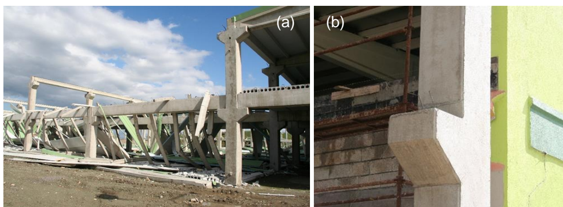
Figure 224: Lightweight precast building (a) Failure of roof beams and cladding (b) Dowels connecting the beams to the column.
