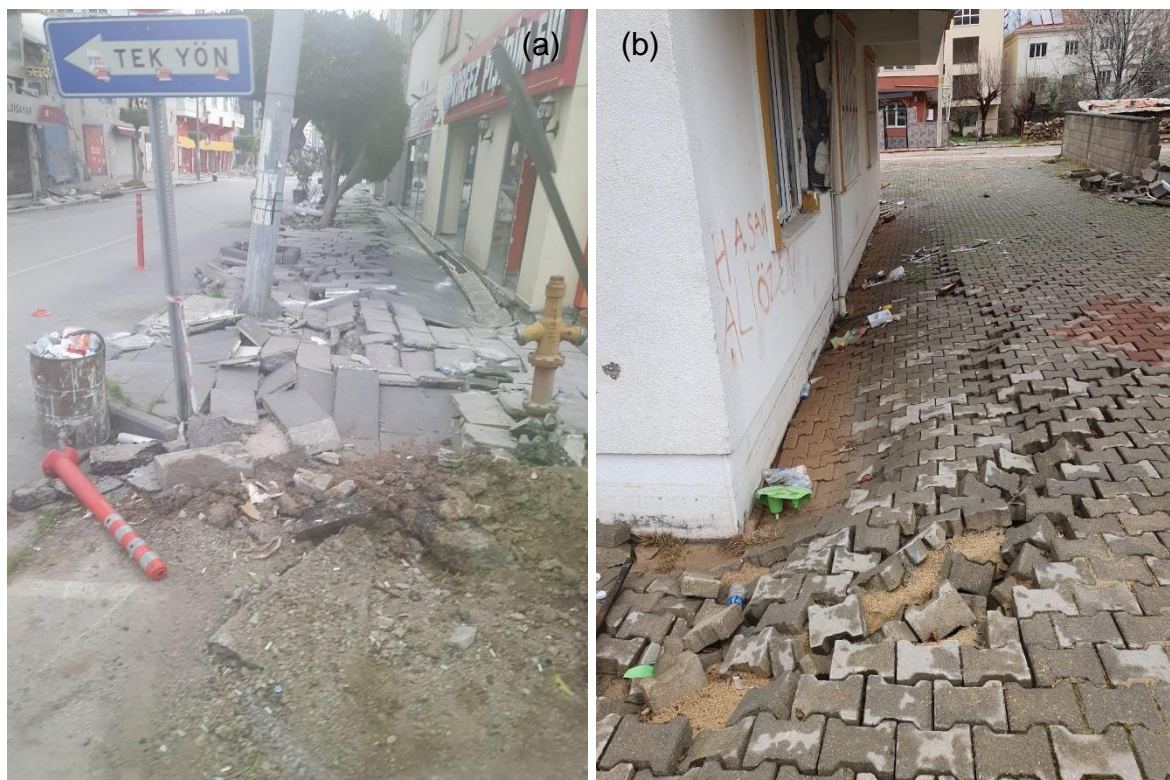
Figure 203: Damaged pedestrian roads – photos taken during the field mission (location: a) Lon 36.5895 Lat 36.1754; b) Lat 37.7887 Lon 37.6482)
