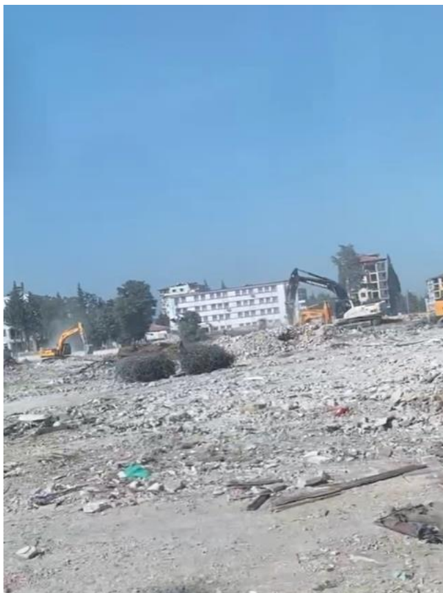
Figure 256: Debris removal in Antakya, showing rebar separated for recycling, 22 June 2023
