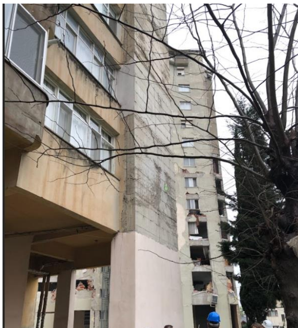
Figure 150: Post earthquake condition of an external shear wall.
