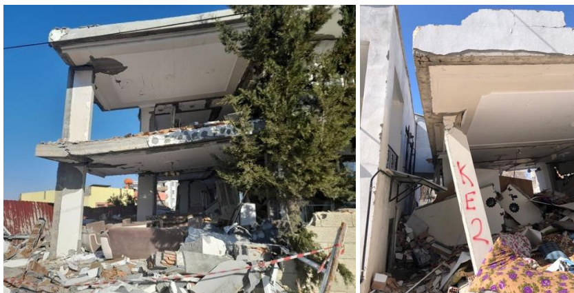
Figure 94: Hollow-tile floor slabs and their strong beam-weaker column effect (City Center/Adiyaman).
