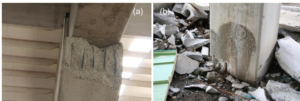
Figure 225: Spalled concrete (a) at the corbel (b) at the column base due to plastic hinge.
