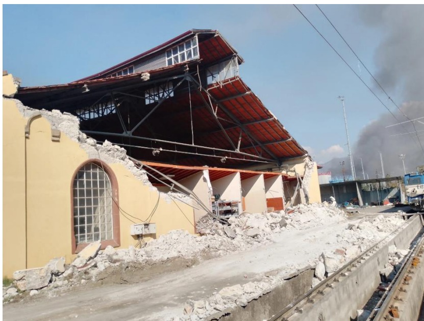
Figure 153: Collapsed building at the Fevzipaşa Train Station [ https://sendikalmucadele.org/btsden-deprem-raporu-demiryollarinda-hasar-fazla/ ].
