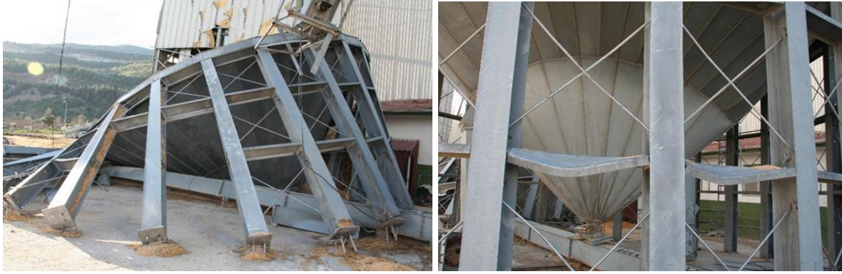
Figure 223: Failure of holding down arrangement and bracing.
