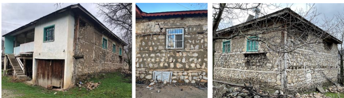
Figure 112: Masonry reinforced with timber elements.
