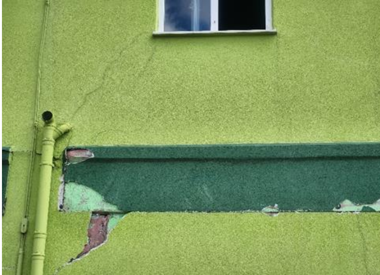
Figure 226: Cracking of infill walls completed unit.
