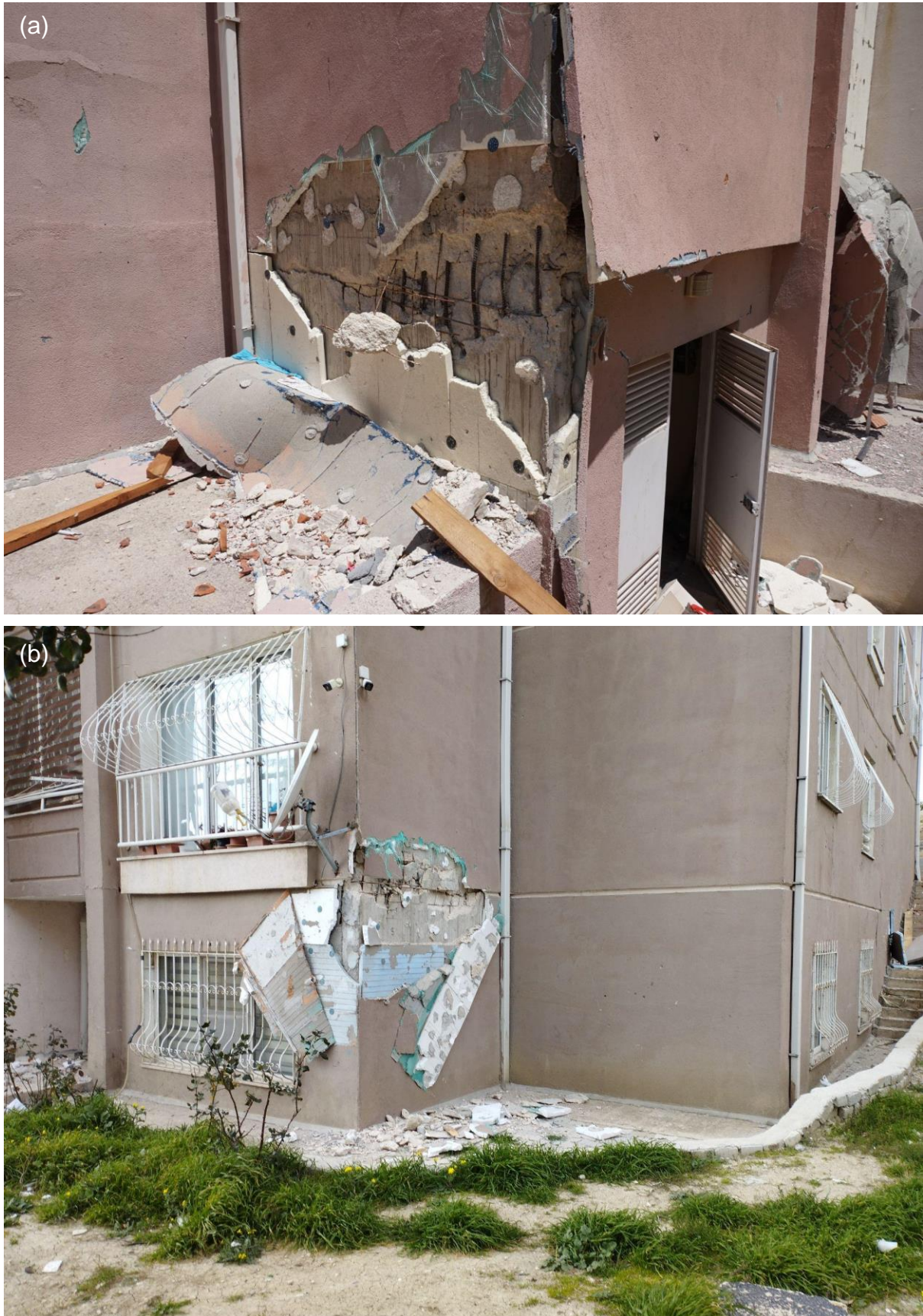
Figure 160: Shear wall damage.
