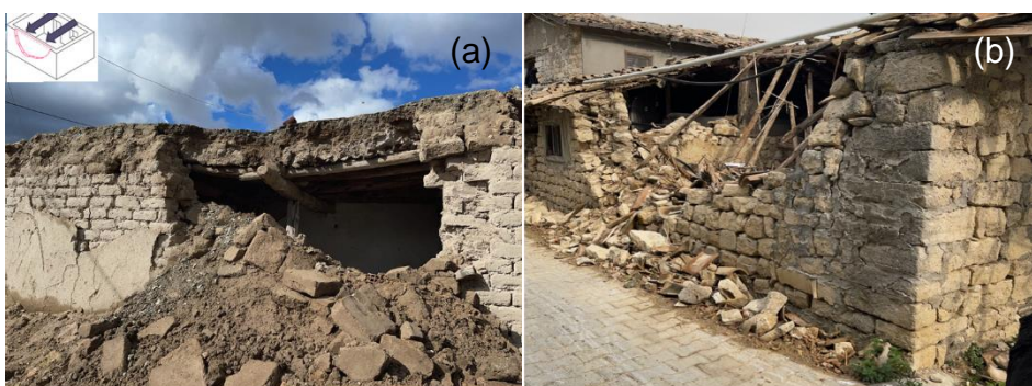
Figure 110: Adobe building failures: (a) Arch failure of the walls due to poor mortar properties; (b) Presence of irregular, small-sized, and round stones or rubble within the wall leaf and a lack of connection between the wall and the roof.
