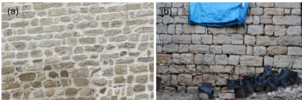
Figure 100: a) Rounded stones with lime mortar, and b) square stones with mortar loss on the surface.
