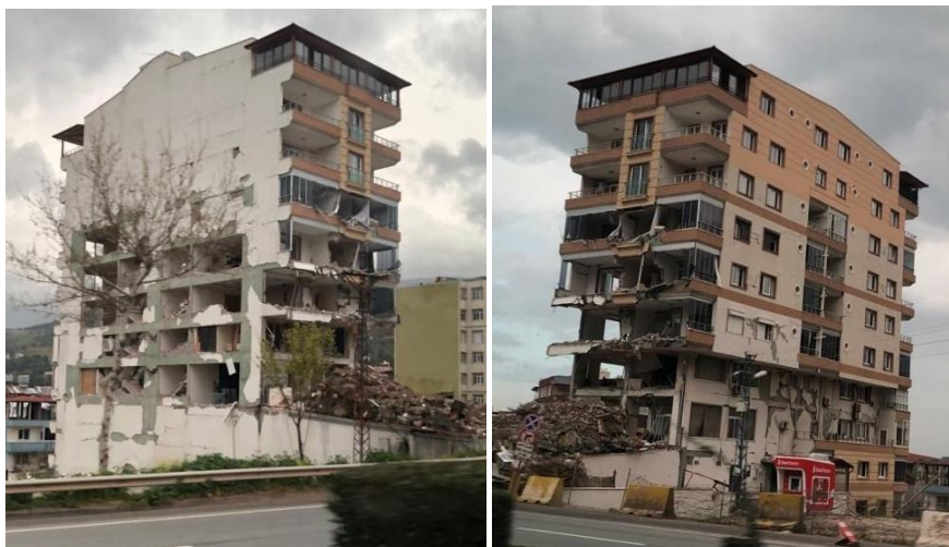
Figure 92: Shear wall damages (Belen/Hatay).
