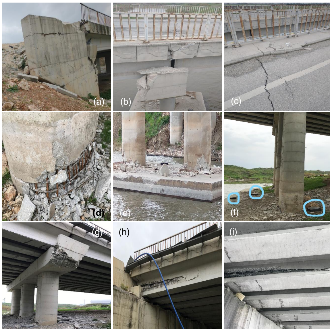
Figure 60: Hatay stadium bridge structural features. (a) movement and tilting of the east abutment, (b-c) deck compression crack, (d) plastic hinging at pillars on west bank (e) plastic hinging at pillars, (f) falling bearings on west bank, (g) shear key failure, (h-i) damaged girder
