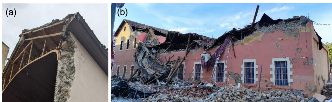
Figure 140: Photographs of damage in structures with roof timber trusses: (a) the Assyrian Catholic Church in İskenderun and (b) the Mithatpasa Primary School in İskenderun.
