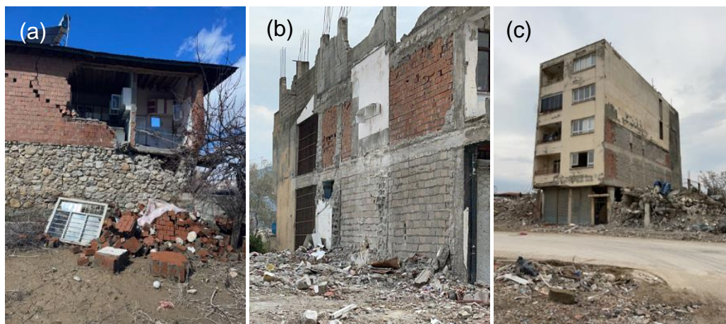
Figure 147: a) OOP failures; b) failed infilled panel and c) Non-Engineered Interventions on a Building with a Vulnerable Soft Storey Due to Large Ground-Floor Openings for Commercial Activities.
