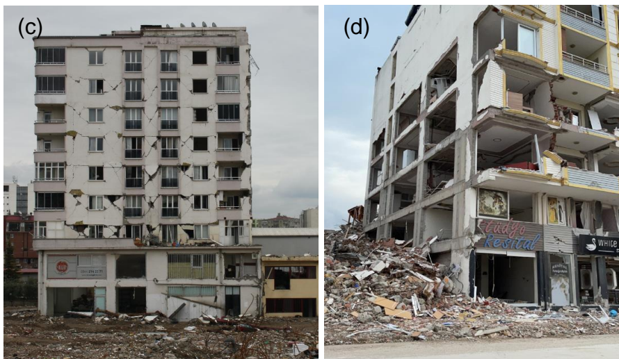
Figure 90: Cracking and fallings of infill walls in (a&c) Kahramanmaraş, (b&d) Samandağ/Hatay).
