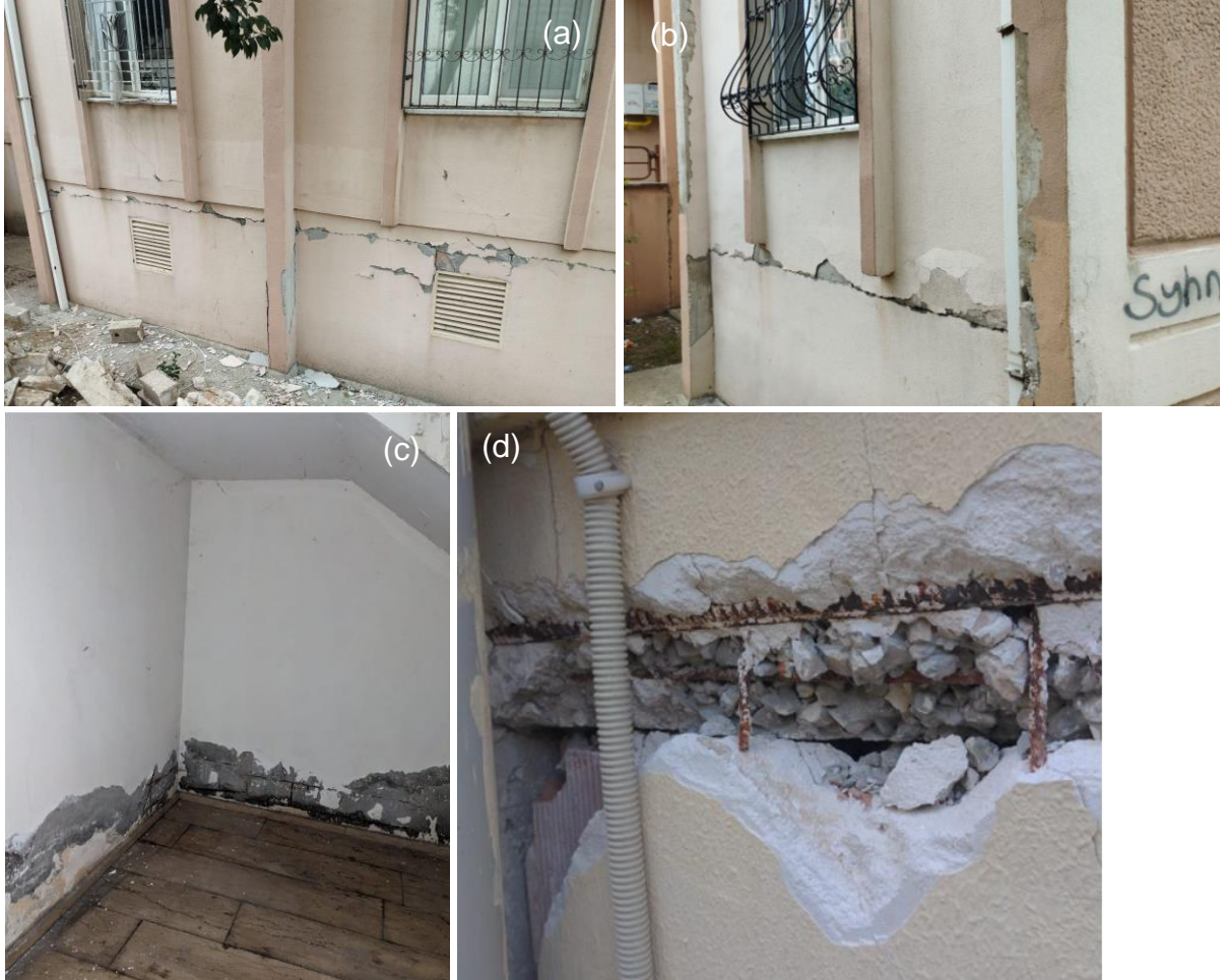
Figure 157: Damage observed in TOKI housing; (a) Separation of infill walls at the ground story and (b) Initiation of cover spalling and separation of infill walls at the ground story; (c) Corrosion of reinforcement on basement floor; (d) Concrete cover spalling and infill wall damage.
