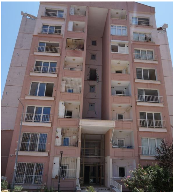
Figure 158: Widespread diagonal cracks in the infills around the window openings.
