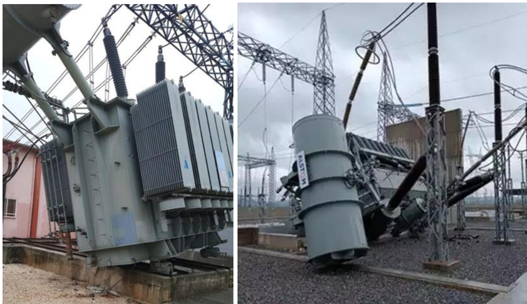
Figure 211: Damaged High Voltage transformers, poor fixing to the rail or foundation: a) Transformer damage, Gaziantep ( source : https://www.instagram.com/yuksekerilim_ariza/ ) and b) Transformer damage, Hatay ( source : https://www.linkedin.com/posts/rehasen_deprem-trafo-reee-activity-7028409428567560192-kcvY/?utm_source=share&utm_medium=member_desktop )
