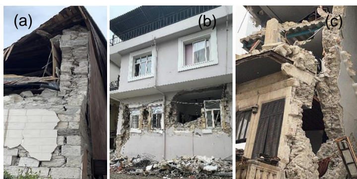
Figure 107: a) Roof failure and severe damage due to leaf separation, b) OOP of localised piers/spandrels; and c) OOP of façade due to lack of connections.
