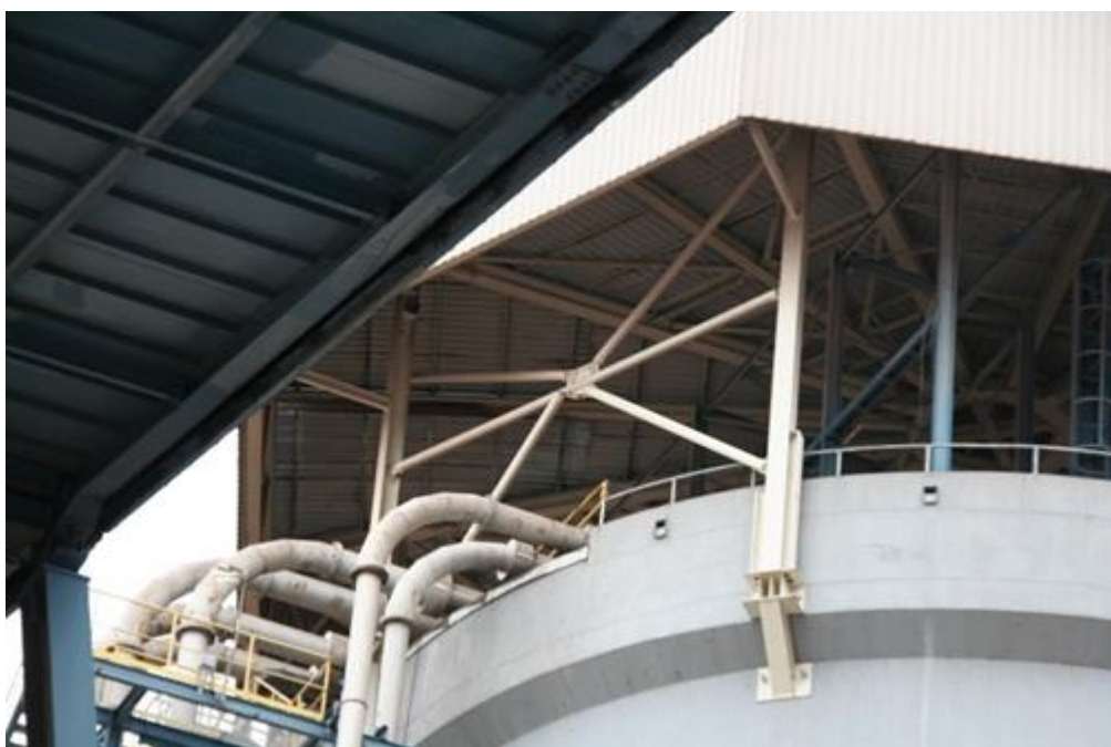
Figure 219: Bracing failure of diesel silo canopy.
