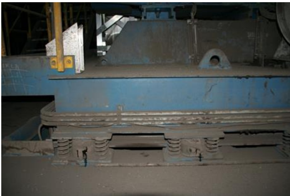
Figure 217: Secondary coal feeding system fallen off the support.
