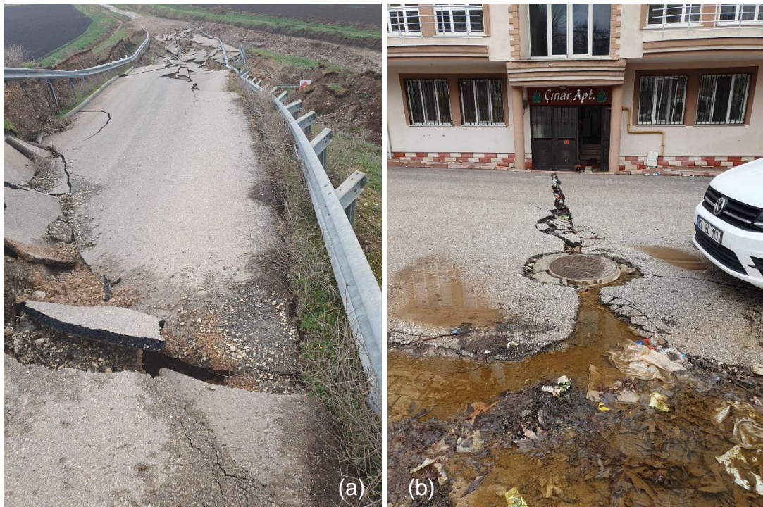
Figure 201: Cracked roadways due to fault lines – photos taken during the field mission (location: a) Lat 37.2836 Lon 37.1141; b) Lat 37.7886 Lon 37.6470
