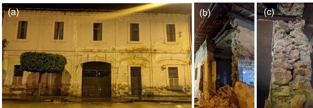
Figure 133: İskenderun High School, photographs of (a) the west façade, (b) the collapsed south-eastern corner, (c) a multi-leaf wall cross-section from the collapsed southeast corner of the building.
