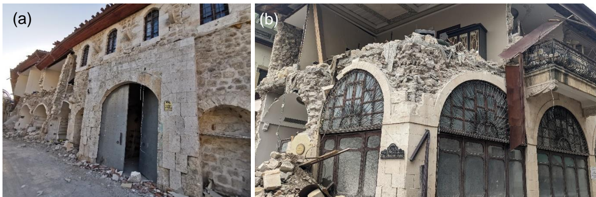
Figure 138: Photographs of damage in two buildings with barrel vaulted floors: (a) south façade of the 16th century Kursunlu Han building in Antakya and (b) the north and west facades of the Shahut hotel building in Antakya.
