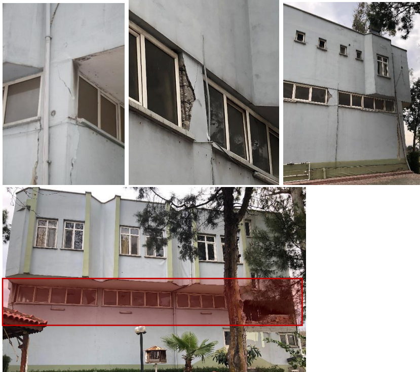
Figure 91: Diagonal cracks in the columns and short column effects (Payas/Hatay).
