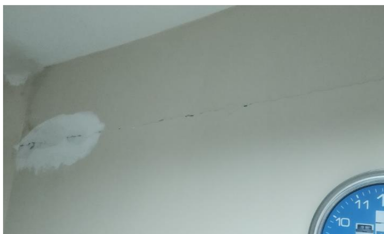
Figure 155: Non-structural crack through the beam-wall connection observed in one of the buildings at Fevzipaşa Train Station.
