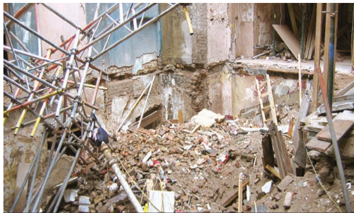
← Figure 6 Result of poorly constructed underpinning
