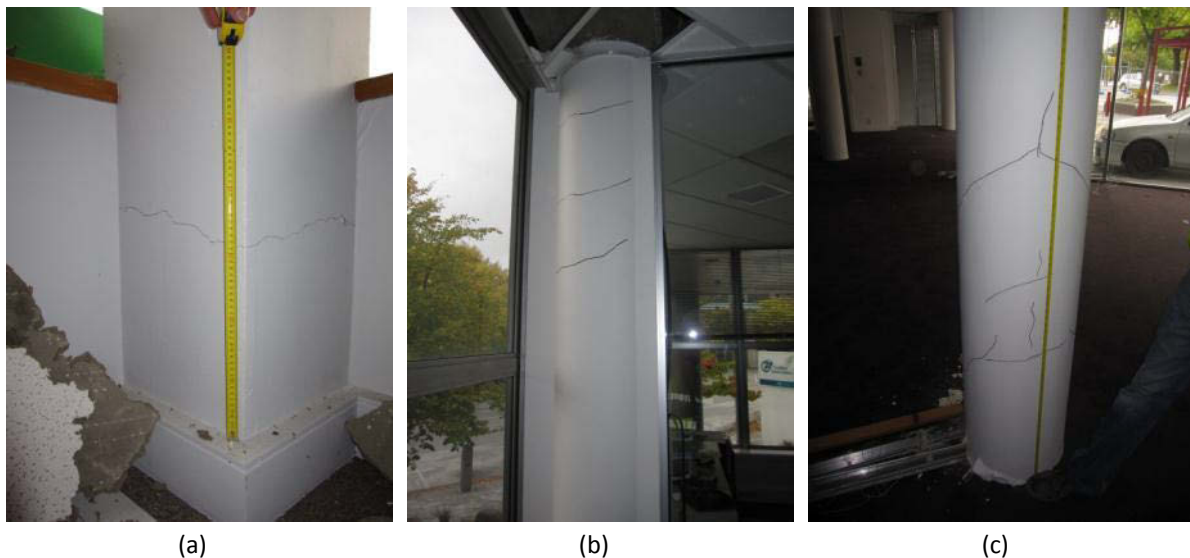
Figure 21 – Column damage observed on Level 2 (internal) inspection of building on Kilmore Street. (a) Flexural crack at ground floor column base; (b) flexural cracking at top of column; (c) potential shear cracking up height of column (note: cracks drawn on column in b and c).
