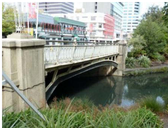
Figure 52 – Steel bridge over Avon River in CBD, showing buckling of outer arch due to movement of abutments resulting from lateral spreading. Although this damage looks significant, the structural system consists of steel girders under the main deck and arches under the footpaths. There was no obvious damage to the main girders.
