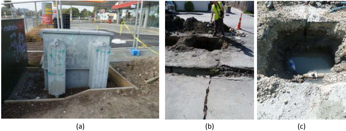
Figure 44 – (a) An electrical services box that had tilted due to liquefaction; it is not known if this resulted in loss of service. (b) A typical services failure that has been exposed ready for repair. This service was located approximately 200m from the river and was damaged from lateral spreading – note the crack in the road substrate in (c), this crack occurred across the entire road surface and is displayed in (b).
