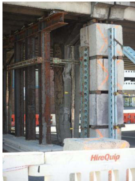
Figure 54 – Moorhouse Avenue overpass, which consisted of many piers (of which two failed). At this particular location the pier consisted of a double column on either side of an expansion joint. The piers were relatively slender about the axis perpendicular to the bridge deck and the pier on one side of the expansion joint formed two plastic hinges about its weak axis due lateral movement of the bridge deck and vertical load. The supporting structure shown in the image was intended to protect the bridge from further damage due to aftershocks rather than to enable reopening. The bridge was still closed at time of survey and was responsible for significant traffic disruption.
