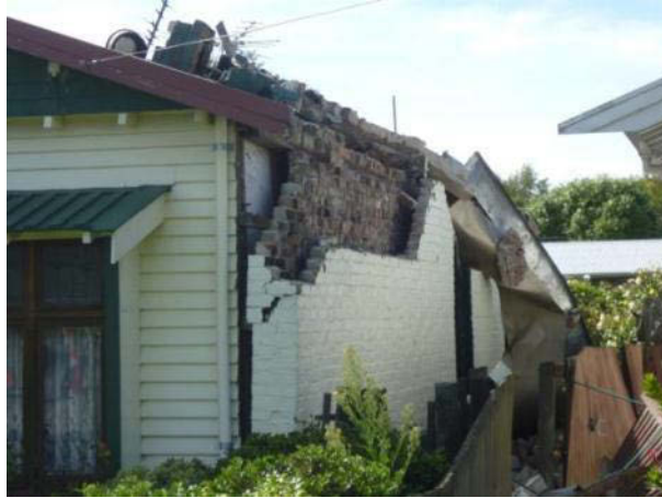
Figure 18 – Masonry wall and chimney collapse on residential timber building. This house has a double-skin masonry wall where the chimney was situated. External assessment shows the timber frame of this building to have performed well, although the masonry wall and chimney have partially collapsed (possibly causing roof damage).
