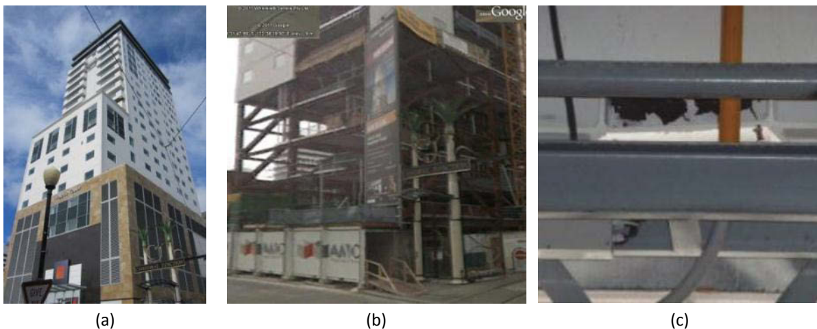
Figure 29 –22-storey steel EBF/Moment Frame building, Pacific Tower, 2010; (a) EEFIT photo from visit; (b) construction photo from Google Streetview, showing perimeter EBFs in lower levels; (c) evidence of EBF link paint flaking due to yielding, and residual deformation, partially obscured by services (Michel Bruneau, from Bruneau et al., 2011).
