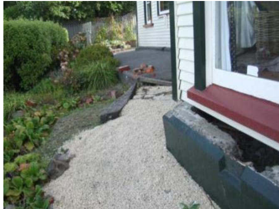
Figure 83 – At this house in Kinsey Terrace the concrete ring foundation had separated from the frame structure due to landslide related ground deformation. Cracks in the garden also occurred and can be seen in the mid-ground
