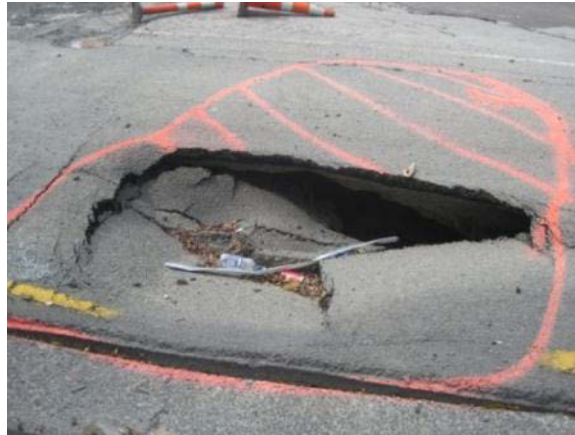
Figure 57 – Ground deformation on Madras St exposing void beneath the pavement.
