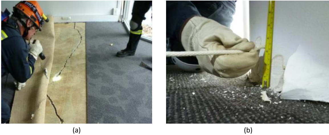
Figure 62 – (a) Cracking in the ground floor slab of a 5 storey building. (b) 75 mm settlement of a column relative to the level of the bulging floor slab.
