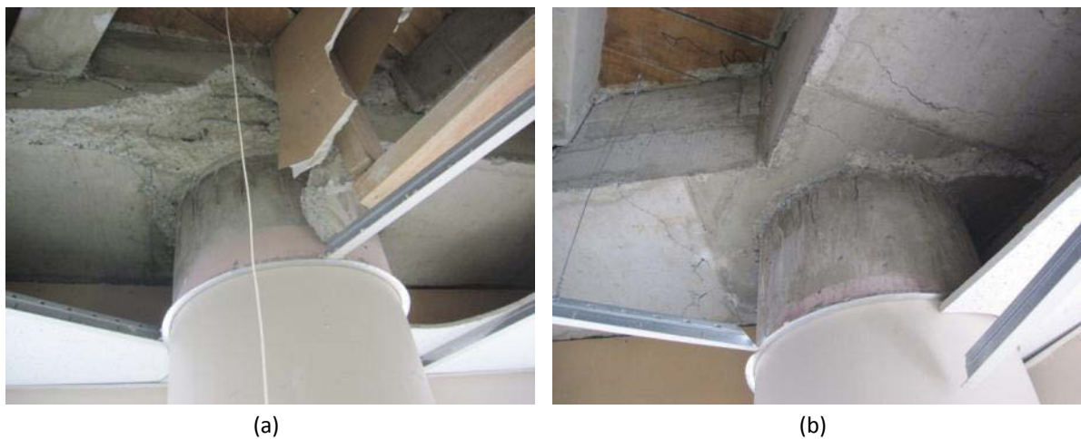
Figure 20 – Beam damage observed on Level 2 (internal) inspection of building on Victoria Street. (a) Internal beam-column joint damage exposing transverse joint reinforcement; (b) flexural cracks on underside of beams at corner beam-column joint.
