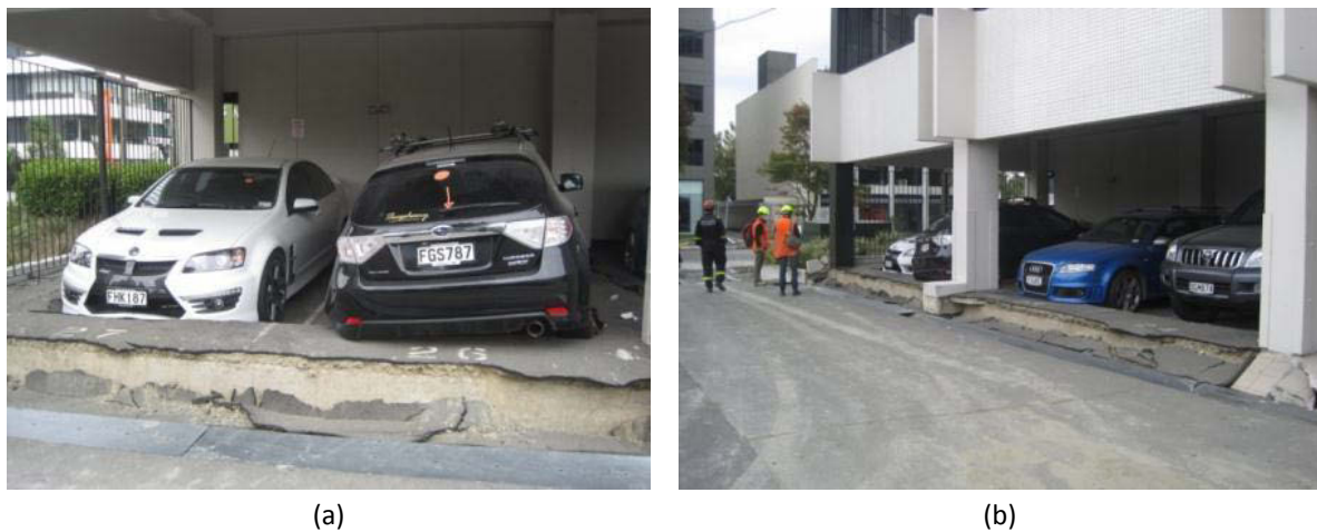
Figure 66 – (a) and (b) Exposed foundation beams in a building with piled foundations.
