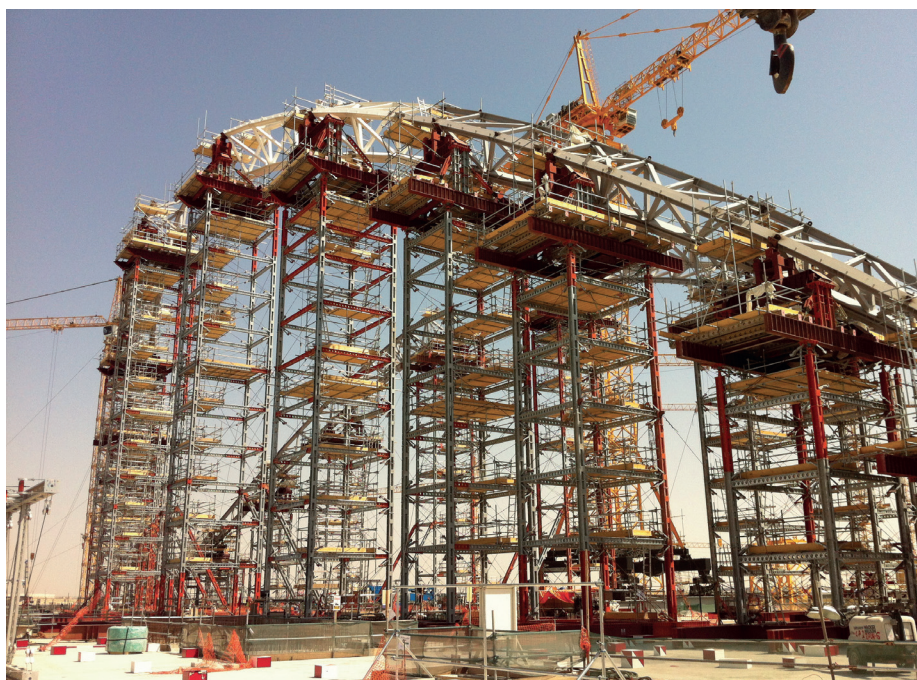
Figure 8 Temporary towers for erection of long-span arch structure. Permanent works design was heavily influenced by temporary condition, with staged global analysis requiring detailed incorporation of temporary works constraints
