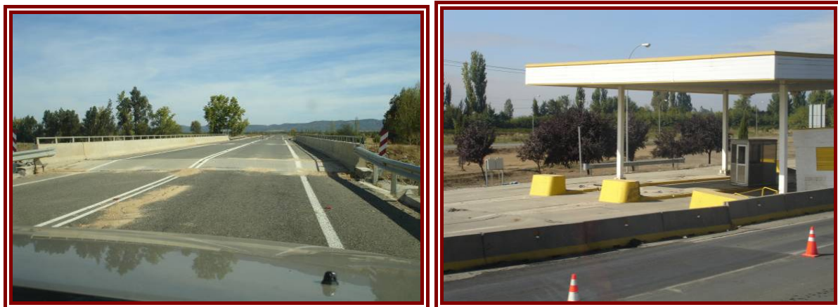
Figure 4-12: Lateral spreading and settlement of bridge abutments occurred at many bridges (left). Road settlement at toll station (right).
