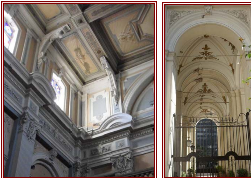
Figure 3-4: Interior corner between façade and south wall of the nave. A crack of separation between the two walls is visible. In the portico a longitudinal cracks runs through all keystones of the vaults supporting the tower. However no lateral permanent sway of the springs is detectable.
