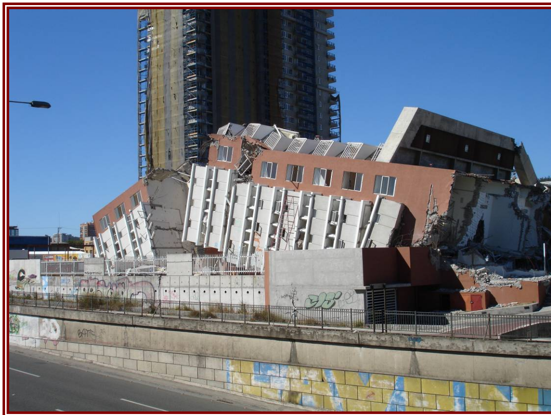
Figure 6-16: Torre Alto Rio (collapsed away from photographer)
