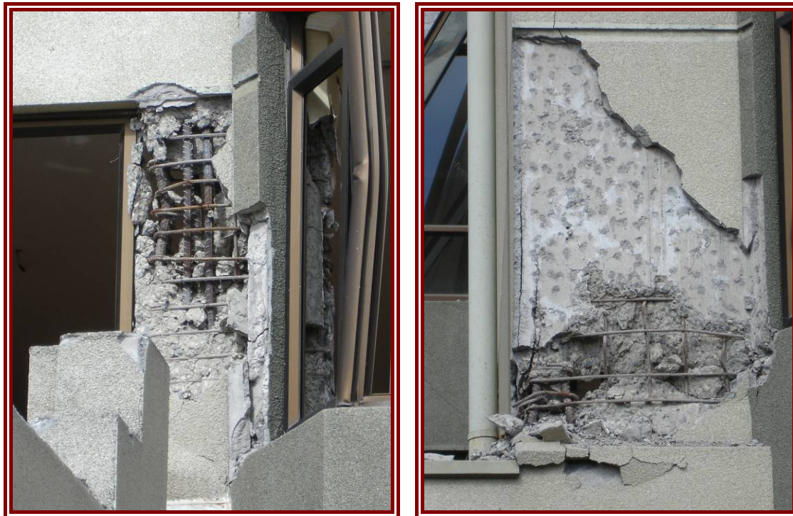
Figure 6-10: Failures to Plaza Mayor I at 1st floor level. Left: Buckling of steel and loss of cover in column elements, Right: lack of links in shear wall elements
