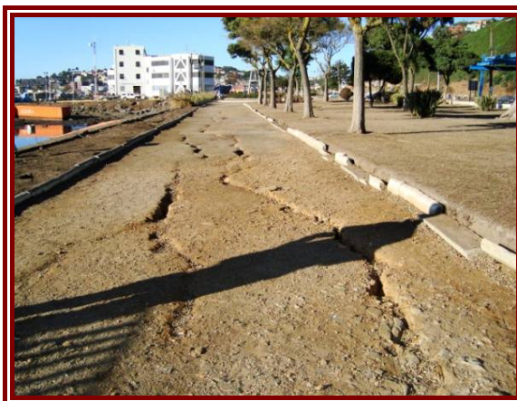
Figure 6-28: Longitudinal cracks Talcahuano Port
