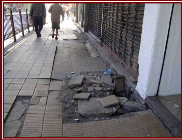
Figure 8-4: Settlement due to water pipeline damage, city of Concepción.
