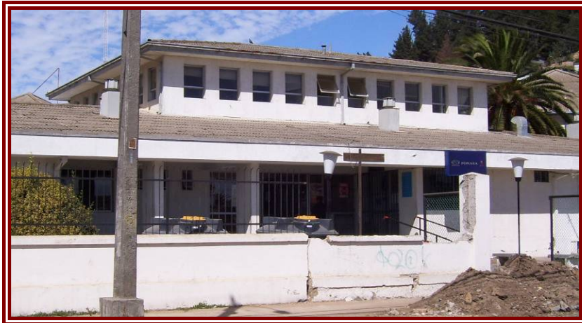
Figure 5-15: Minor damage to hospital building in Constitución
