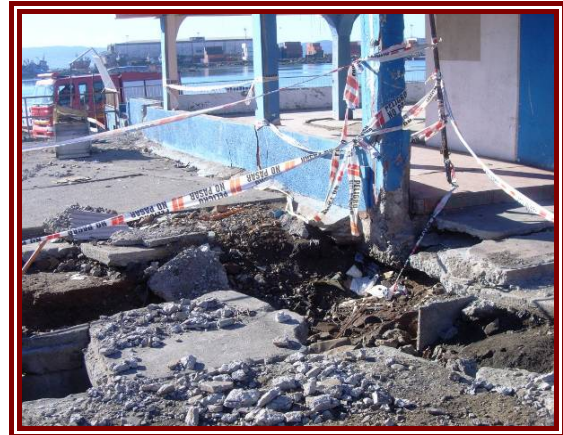
Figure 6-31: Scour damage to building foundation
