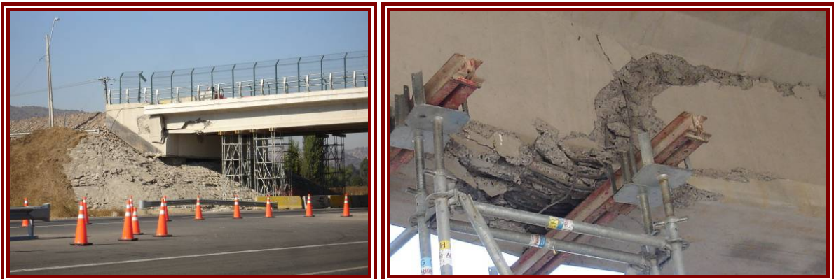
Figure 4-11: Typical damage to overpass bridges near Santiago (left). Prestressing tendons can be seen in the detail on right (right).
