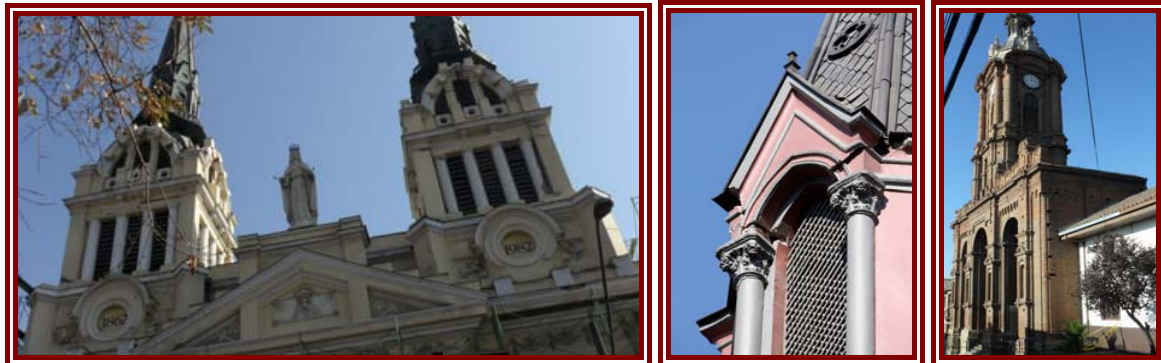
Figure 3-7: a) Twin bell towers in brickwork and timber of the Maria Santissima Sanctuary, damage in the columns and leaning of the timber structure of the left tower. b) Church off Enrique Mac Iver, shear failure at the base of the spire. c) Church of convent of San Francisco in Valparaiso. The convent was initially set in 1845 and the church in 1851 completed with the façade, also by Edoardo Provasoli, in 1890. Was declared national monument in 1983 and partially destroyed by a fire in the same year. It shows vertical cracks over the façade arches and cracks at the base of the tower. Damage to the arches more pronounced than in the case of the Providencia.
