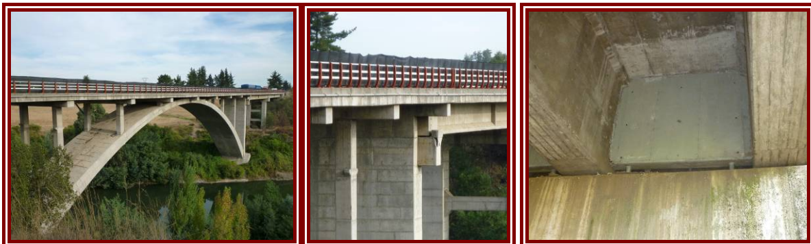
Figure 5-20: Rio Claro Bridge (northbound traffic), shear failure of transverse shear key at midspan, and evidence of retrofit or repair from previous earthquakes
