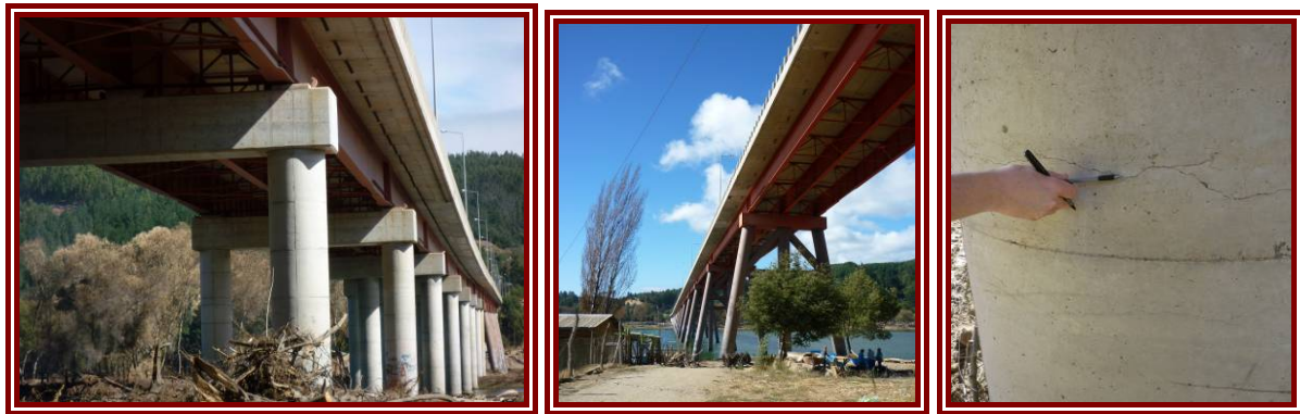
Figure 5-21: Cardenal Raul Silva Henriquez Bridge, Constitución. Concrete piers at north-east end, and raked steel piers at south-west end. Light cracking to concrete piers.
