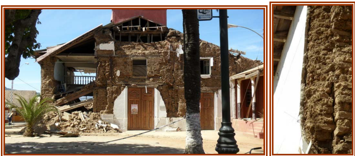
Figure 5-4: The parish Church in Curepto: loss of the façade plaster and partial collapse of the south nave. The anchoring system is visible in façade at the ceiling level.
