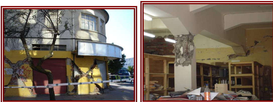
Figure 6-14: Views of the damage to Anibol Pinto 820
