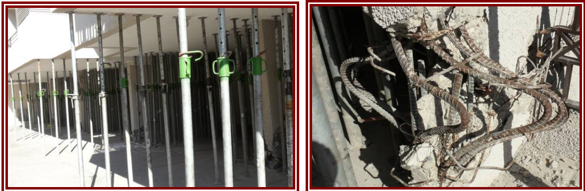
Figure 3-12: Propping due to severe buckling in boundary zones of shear walls
