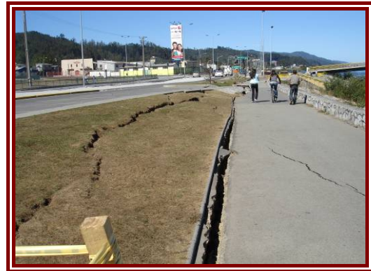
Figure 6-25: Evidence of lateral spreading on the north bank of Biobío river
