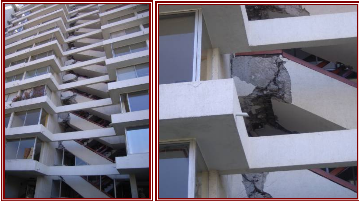
Figure 3-11: Edificio Festival, Viña del Mar, damage to stairwells
