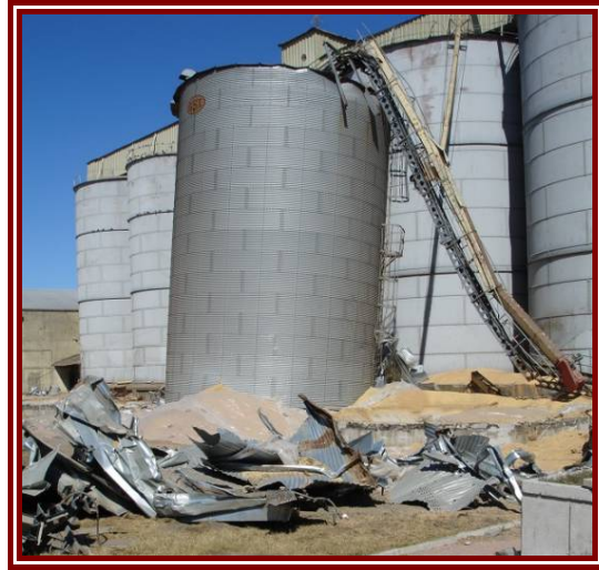
Figure 6-37: Leaning silo and damaged grain conveyor
