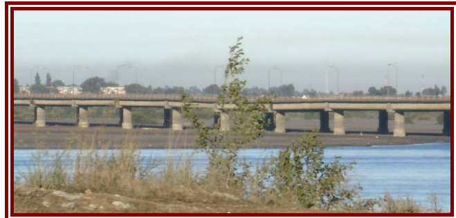
Figure 6-27: Signs of pier settlement on the Juan Pablo II bridge
