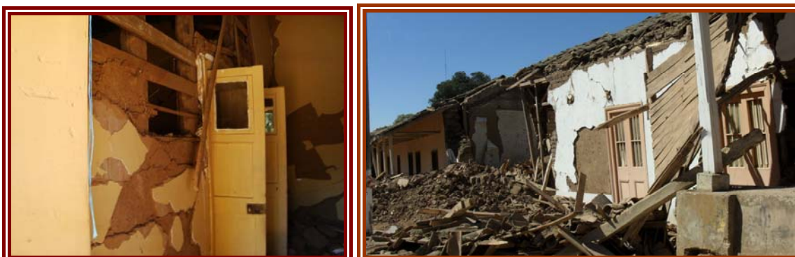
Figure 4-7: Pumanque: Adobe house confined with lightweight timber and damage to row of houses on main street.
