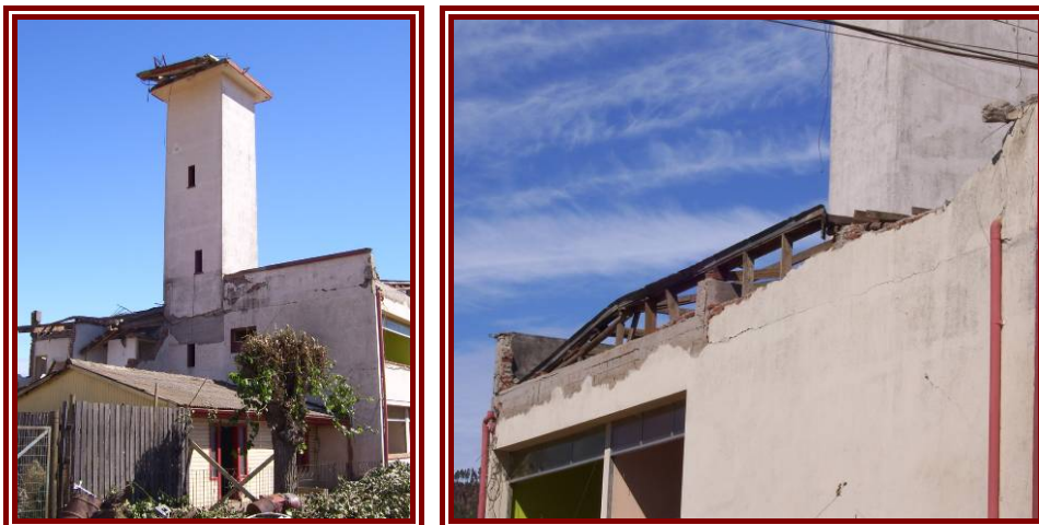
Figure 5-16: Severe damage to fire station in Constitución including collapsed tower and parapet, and damage to external walls
