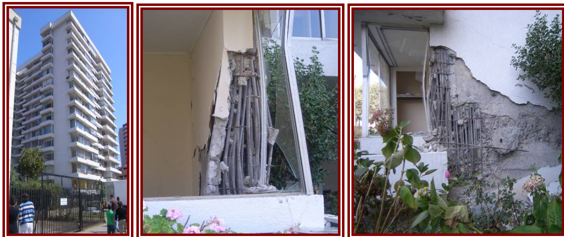
Figure 3-10: Edificio Festival, Viña del Mar, and damage to shear wall boundary zones
