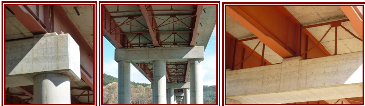
Figure 5-22: Cardenal Raul Silva Henriquez Bridge, Constitución. Displaced shear keys and significant residual lateral displacement, residual displacement along bridge and buckling of girder lateral bracing.
