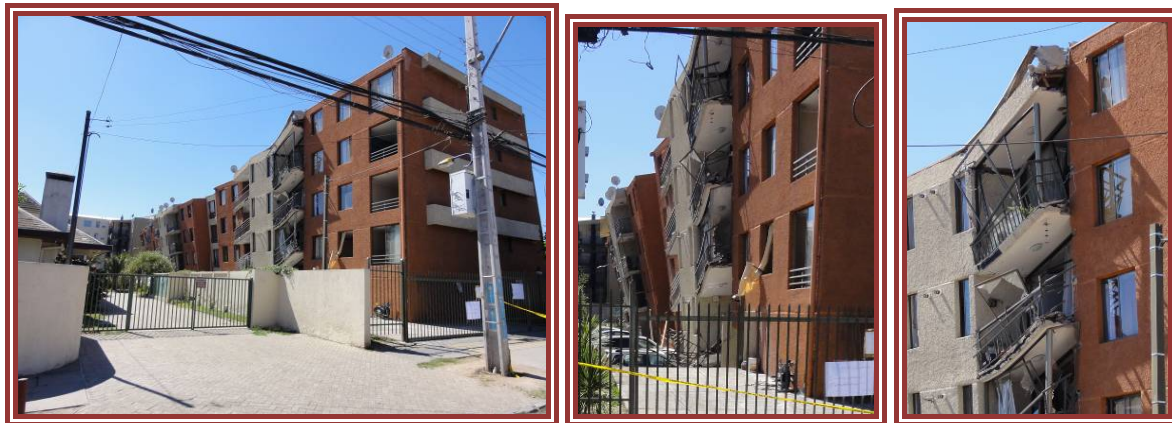
Figure 3-15: Damaged apartment block in Maipu district (Tristan Valdes), Santiago, general views and detail of the damage at the connection of two parts of the building with different ground floor structural system.
