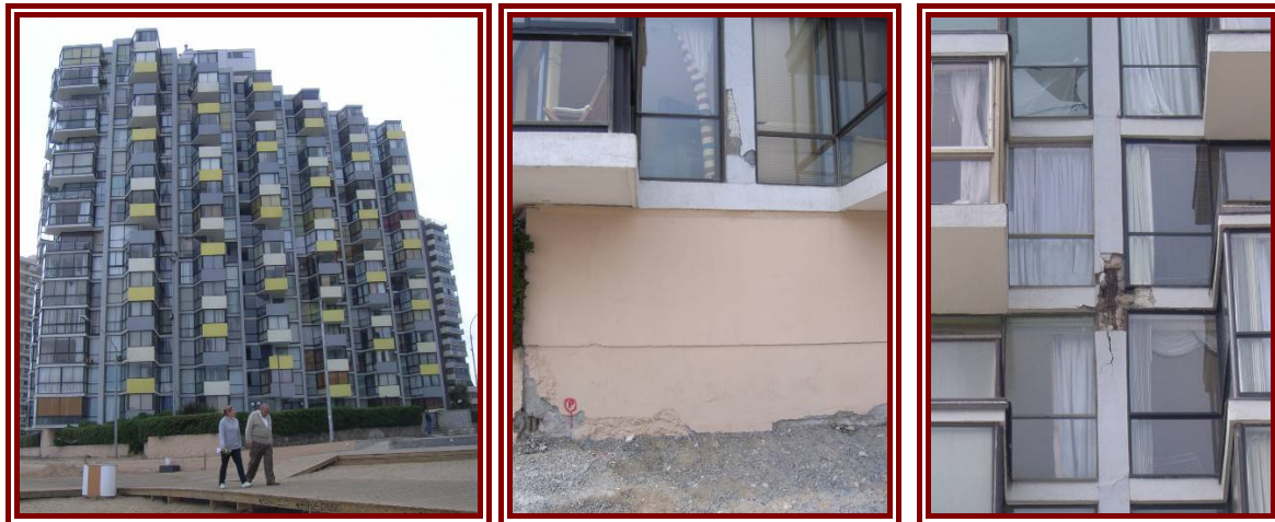
Figure 3-13: Waterfront apartment building, Viña del Mar, external damage
