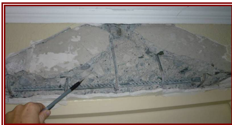
Figure 5-8: Edificio Amalfi – Heavy spalling of door lintels but core concrete intact.
