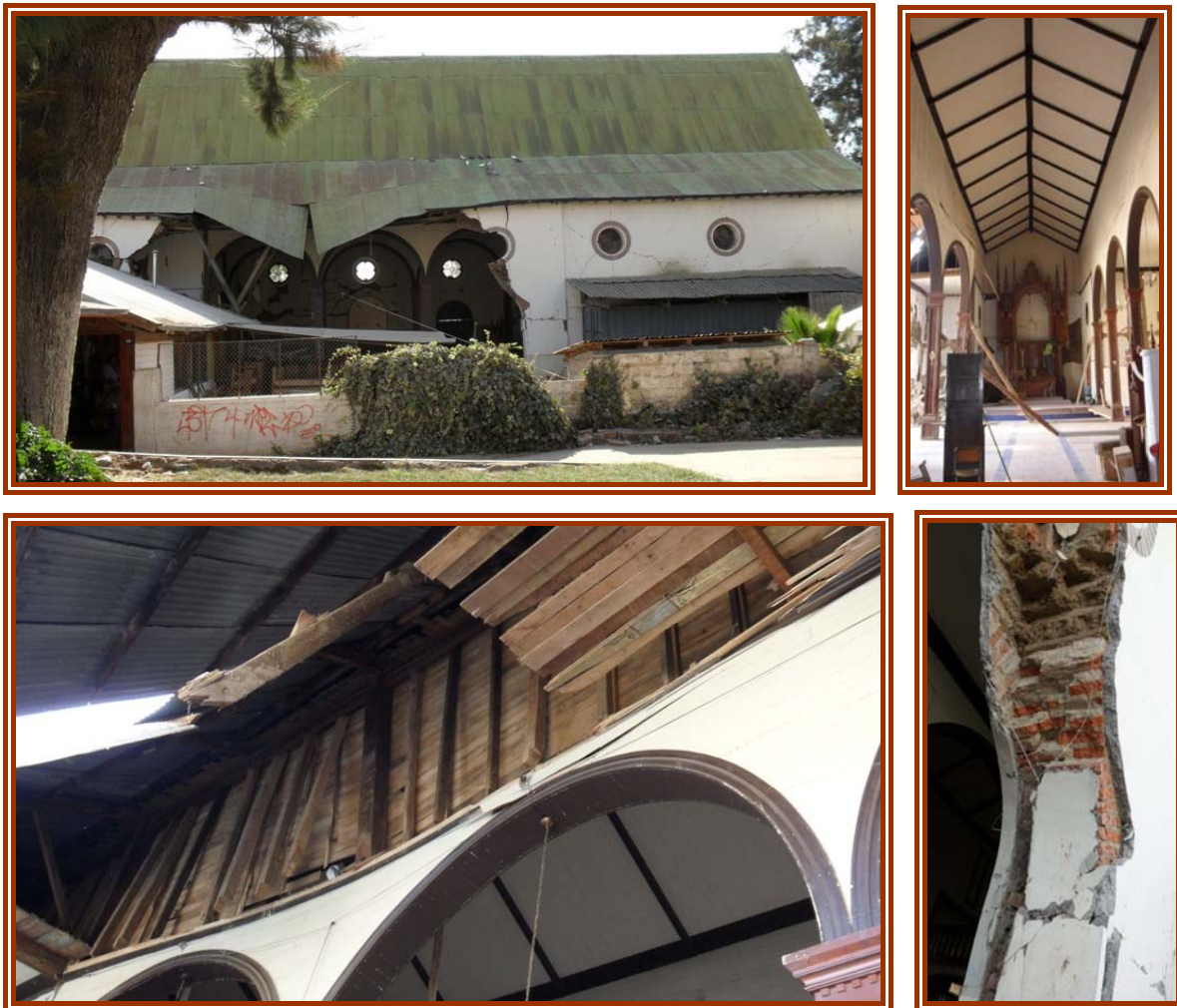
Figure 4-9: The parish Church of Lolol: failure of the side walls around the lateral door, view of the internal structure of the nave in timber, Detail of the timber cladding above the arches, detail of the shotcreting of the external sidewalls introduced as repair after 1985 earthquake.
