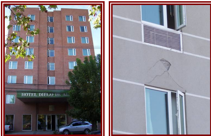
Figure 5-6: Hotel Diego de Almagro and light damage above windows on 2 nd and 3 rd floors
