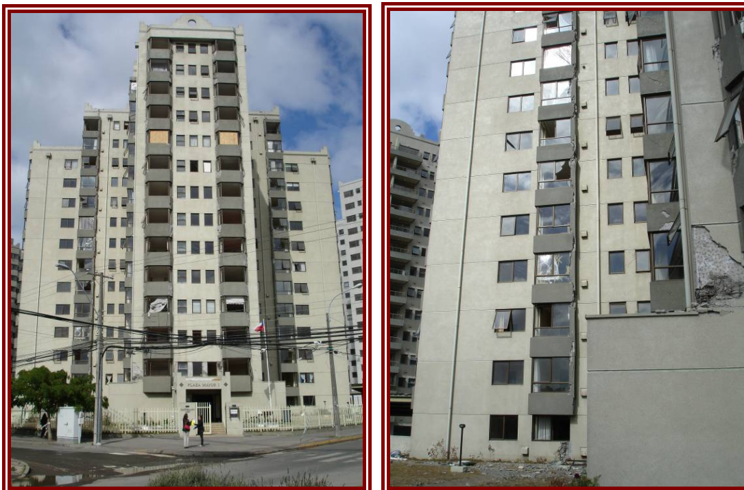
Figure 6-9: Plaza Mayor I (2002) showing extensive damage around projecting windows.
