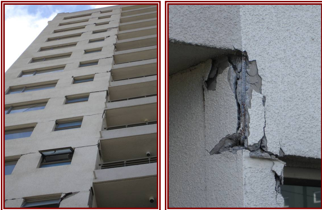
Figure 6-12: Damage up the full height of Plaza Mayor IV (left), Detail of beam column connection in Plaza Mayor IV (right).
