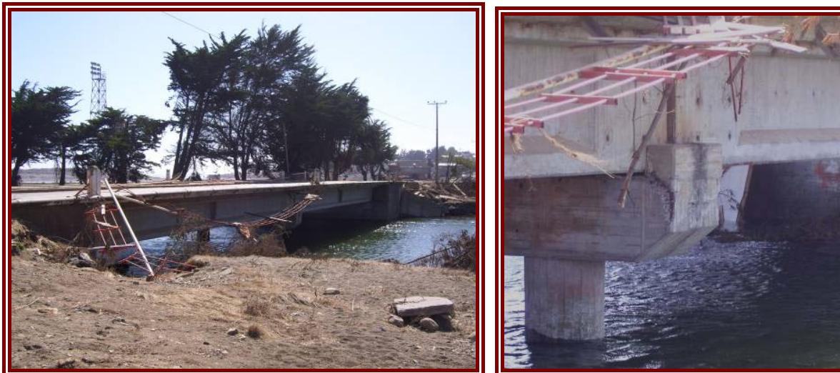
Figure 5-24: Bridge on M-80-N in Pelluhue, and damage to shear key on upstream side.
