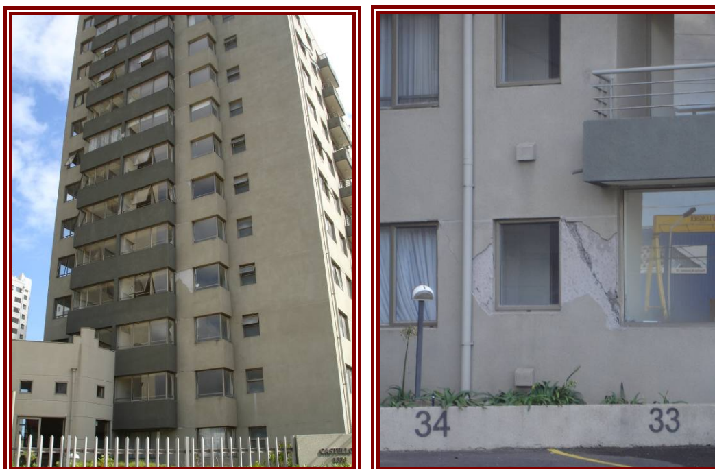
Figure 6-11: Minor external damage to Plaza Mayor II (left), Detail of cracking of shear walls in Plaza Mayor III (right)
