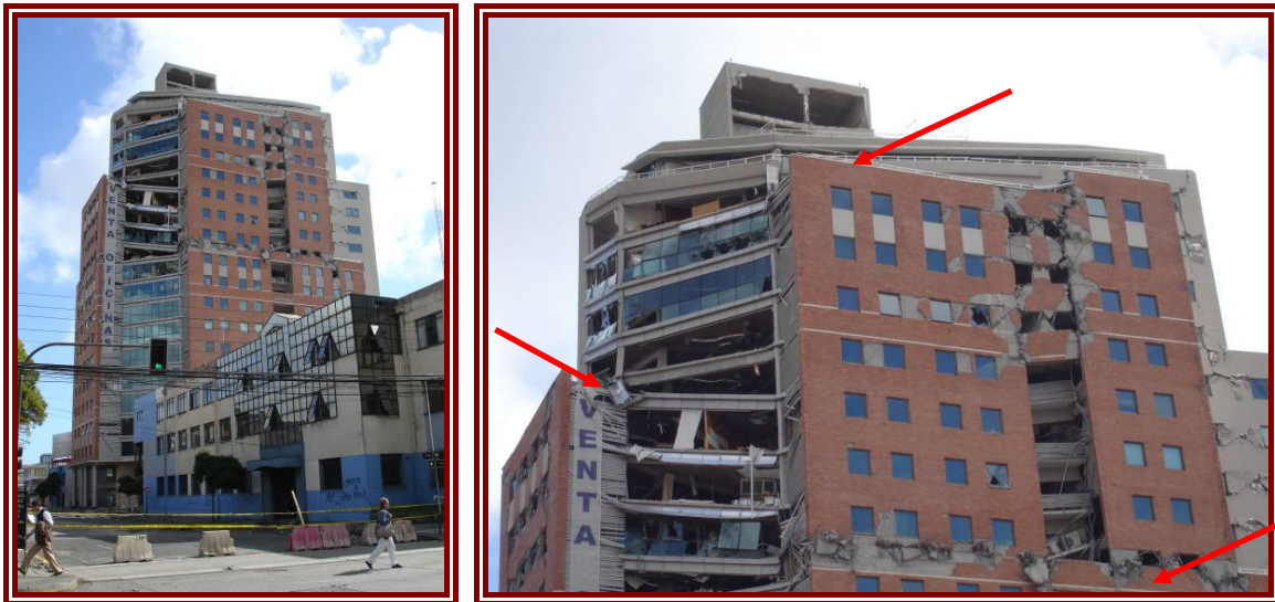
Figure 6-5: Torre O'Higgins 241. On right the 3 soft storey collapses are identified with the arrows.
