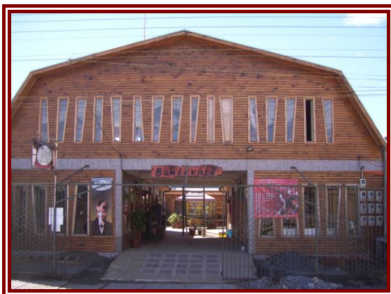
Figure 5-12: RC frame building with timber infills and practically no damage
