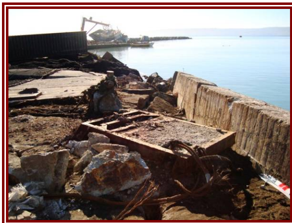
Figure 6-29: Retaining wall failure Talcahuano Port
