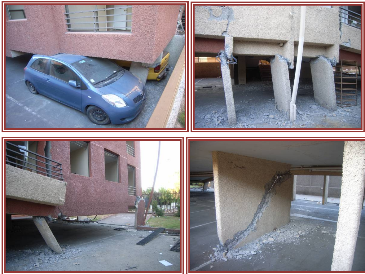
Figure 3-17: Details of the damage to the ground floor of the apartment block in Figure 3-16
