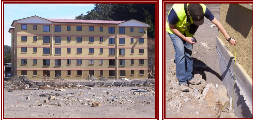
Figure 5-11: Apartment building near waterfront in Constitución and scour at foundations
