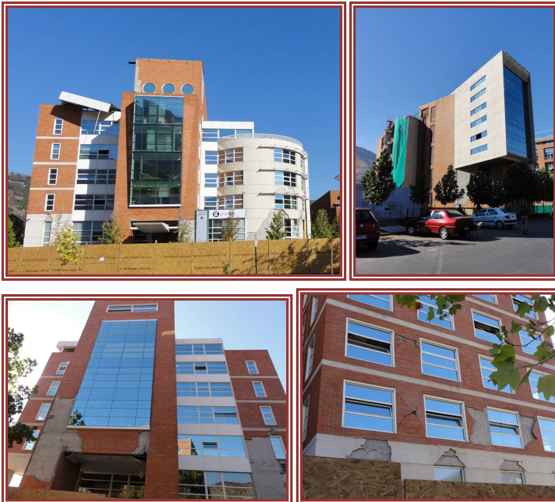
Figure 3-20: Damage to the structural system and facade of some modern buildings in Ciudad Empresarial, Santiago
