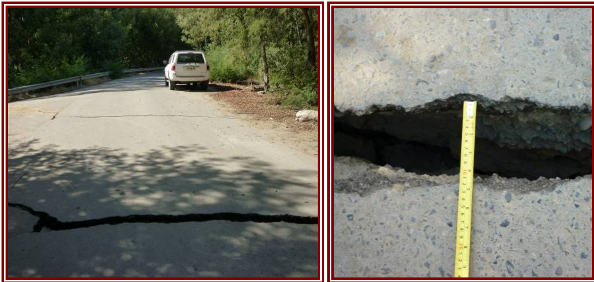
Figure 5-23: Significant lateral spreading of soil and damage to roadway close to Cardenal Raul Silva Henriquez Bridge, Constitución.
