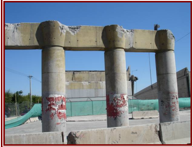
Figure 3-25: Damage to tops of support portals.
