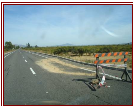
Figure 4-16: Typical damage to minor roads
