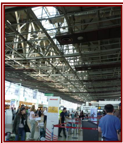
Figure 3-21 Santiago airport – suspended ceiling collapse
