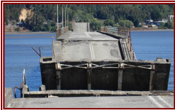
Figure 6-24: Span failure in the Puente Viejo Bridge
