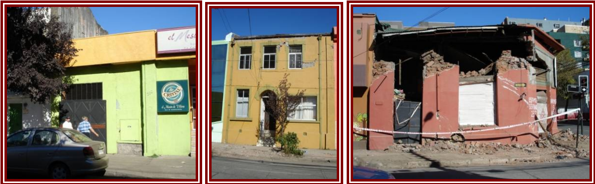
Figure 6-2: Examples of damage assessment from photos: (left to right) Superficial damage, Moderate Damage, Substantial to Very heavy damage
