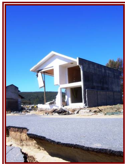
Figure 6-33: Damage to house and road, Dichato
