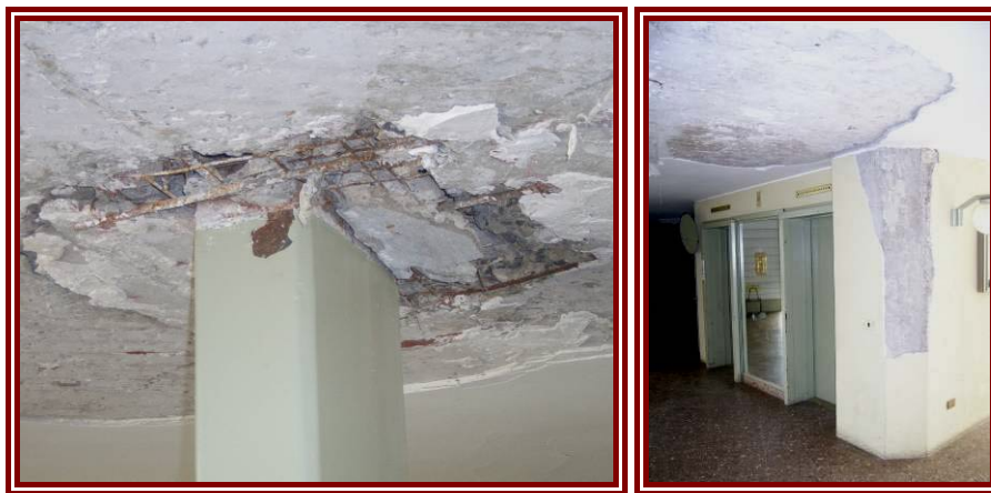
Figure 3-14: Waterfront apartment building, Viña del Mar, internal damage
