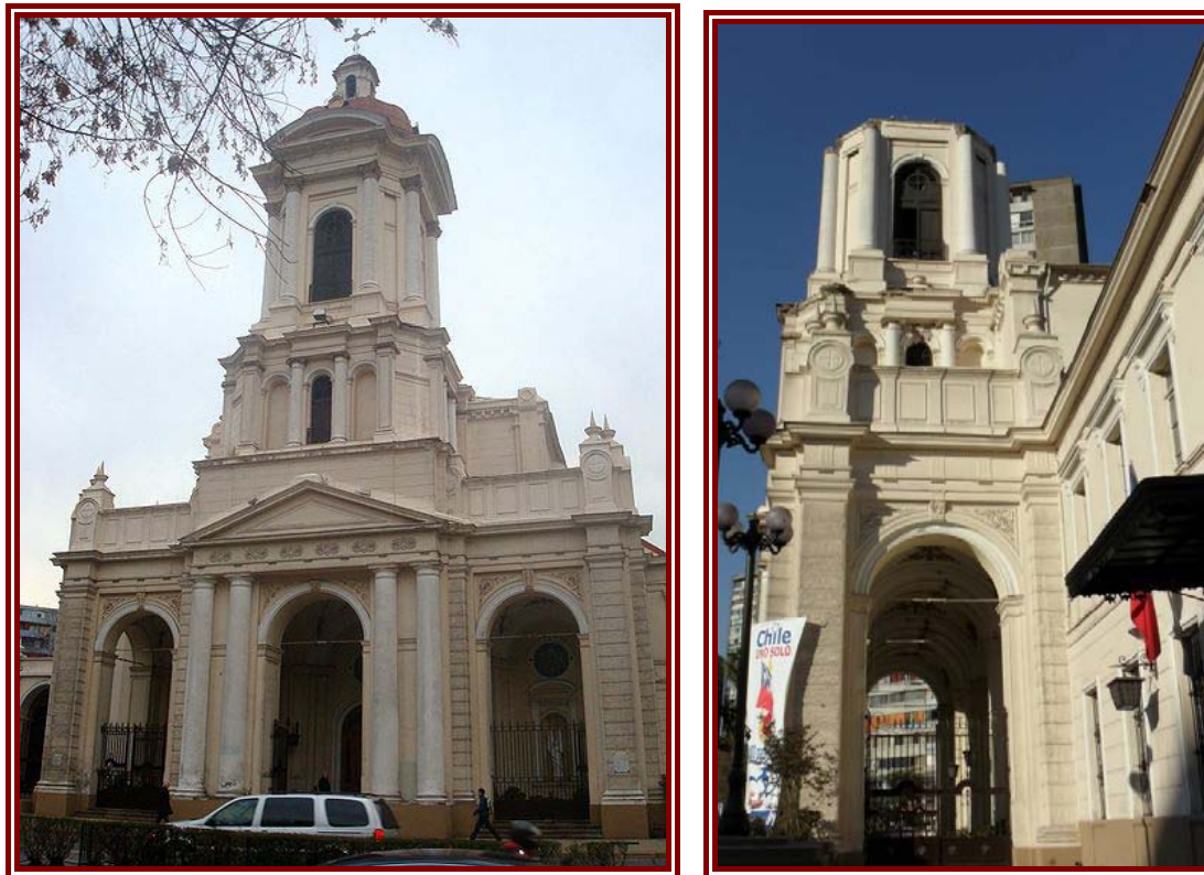
Figure 3-3: Iglesia de la Providencia: Façade elevation before and after the earthquake. The cap of the bell tower has been lost.
