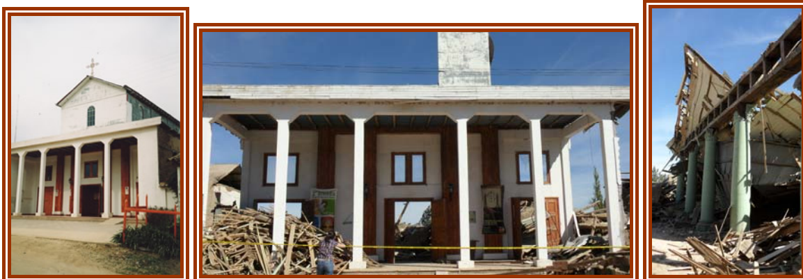
Figure 4-6: Pumanque: Nueva Senora del Rosario Church, before and after the earthquake. The green columns of the main nave are made of a steel profile with an outer concrete casting and the roof rests on a timber verendeel truss.
