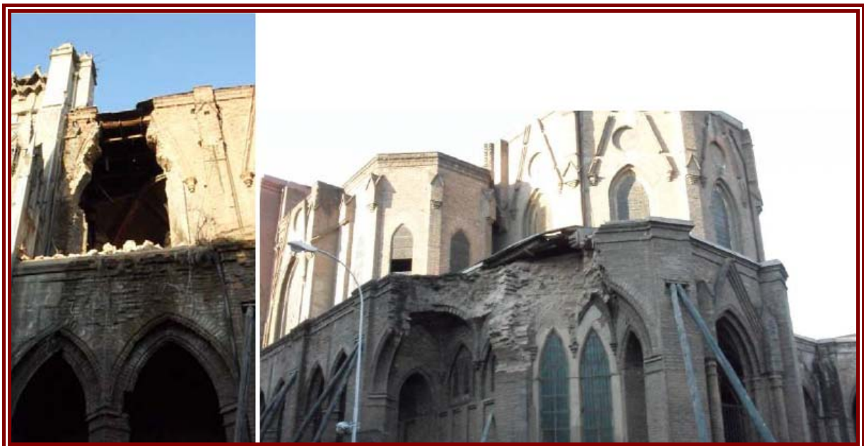
Figure 3-6: Loss of material at the intersection between façade and southern elevation where there is an abrupt change in stiffness. The missing portion of the south east chapel fell as a solid boulder.
