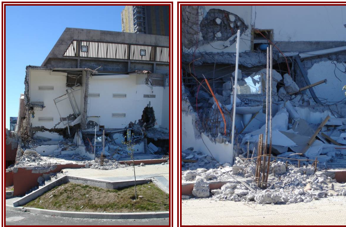
Figure 6-17: Torre Alto Rio. View of 1 st floor ceiling (left), Detail of remains of 1 st floor columns at foundation level (right)
