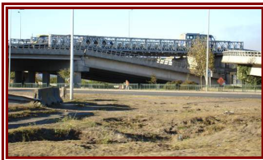
Figure 6-26: Collapsed approach span on the Llacolen bridge
