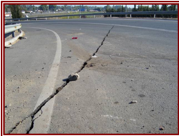
Figure 4-14: Crack in 5 Sur Road between Santiago and San Fernando City.
