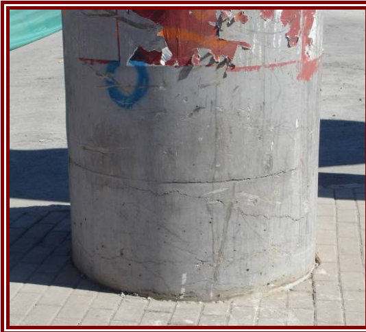
Figure 3-24: Minor cracking at base of concrete columns
