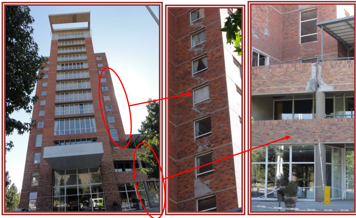
Figure 3-18: Damage to a hotel in Ciudad Empresarial, Santiago
