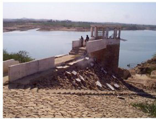
Figure 42 Failure of the appurtenant structures
