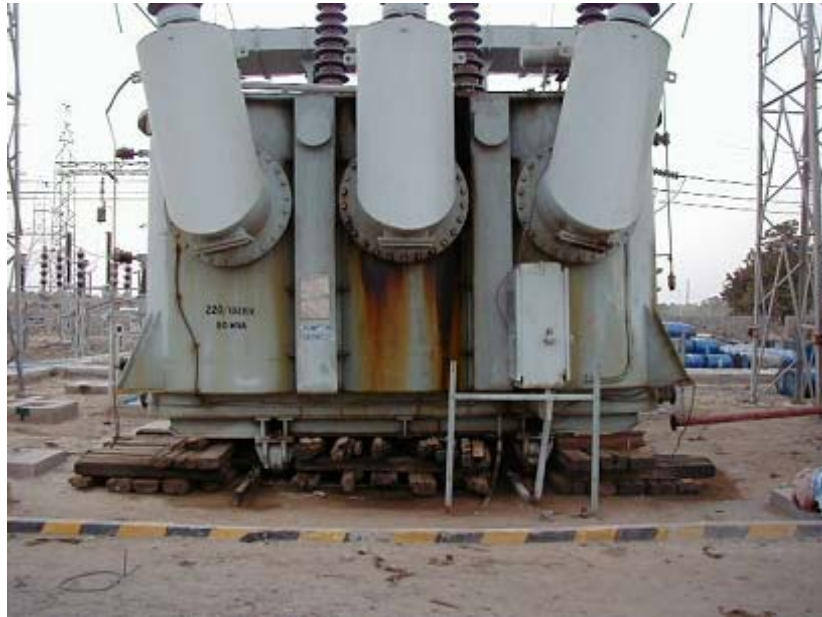
Figure 62 Transformer on Temporary Supports at Anjar Substation
