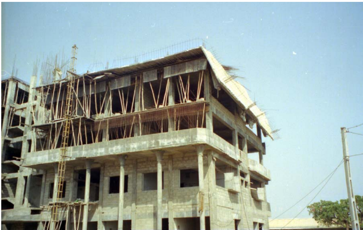
Figure 55 Kandla Port: collapse of cantilever overhang of building under construction
