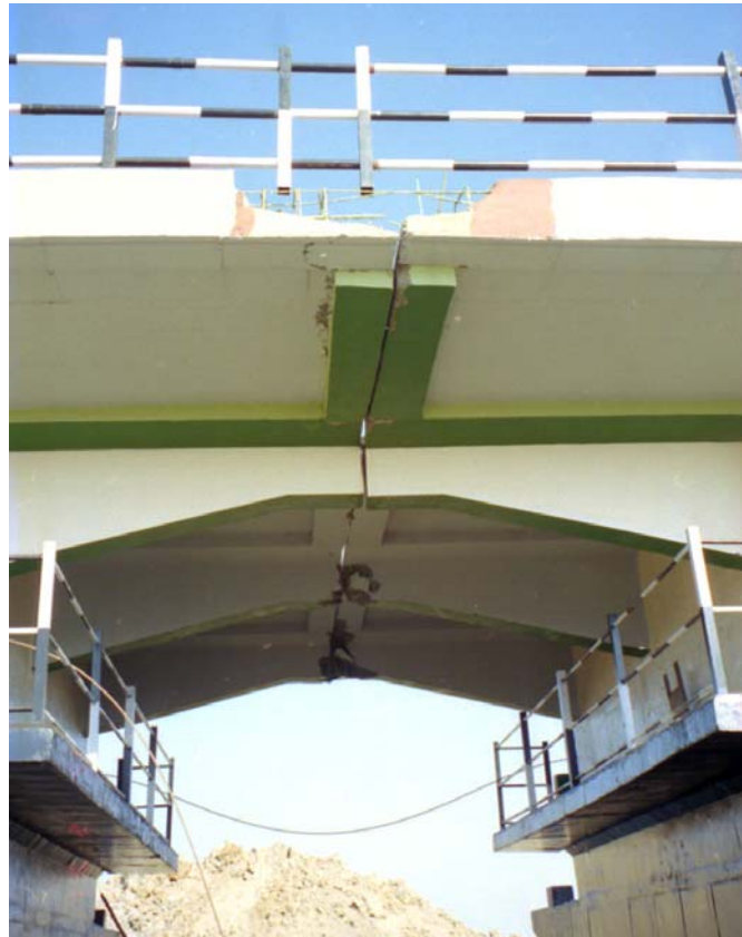
Figure 27 Surajbari New Bridge: pounding between ends of adjacent spans had caused some damage
