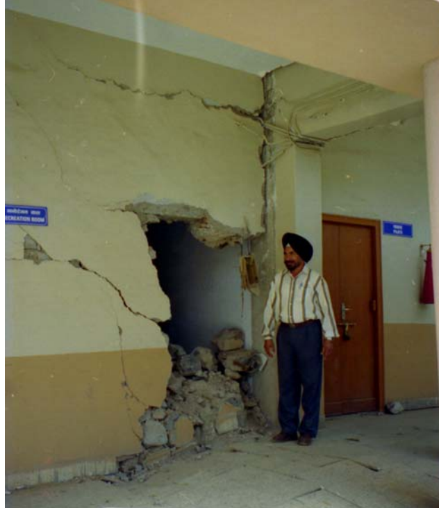
Figure 52 Kandla Port: single storey annex at the rear of 4-storey administration building had shallow foundations and had suffered from settlement and lateral spread of founding soil
