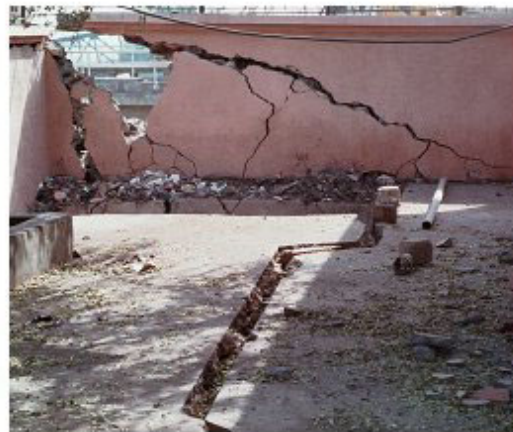
Figure 29 Collapsed wall due to lateral spreading
