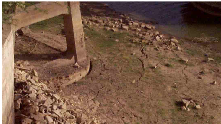
Figure 11 Lateral spreading next to the well caisson
