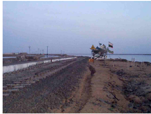
Figure 37 Lateral spreading next to the track
