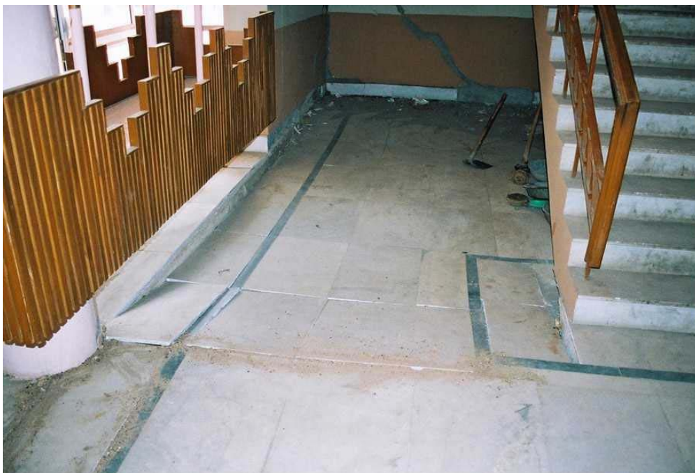
Figure 53 Kandla Port: Similarly, the ground slab of the main building had settled and required replacement
