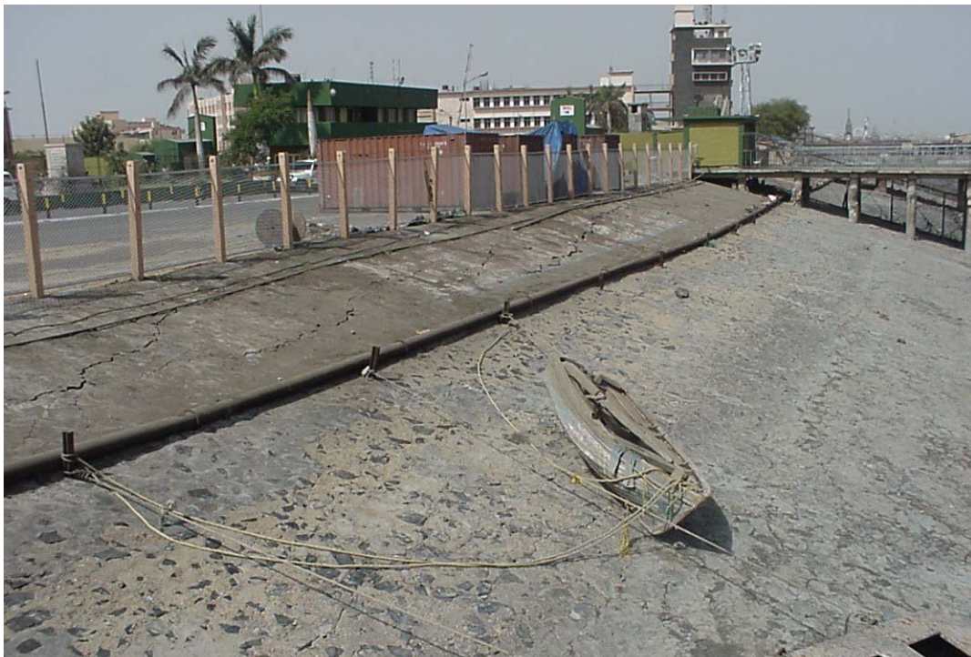
Figure 46 Kandla Port: armoured slope had longitudinal cracks showing there had been some lateral spreading of the fill
