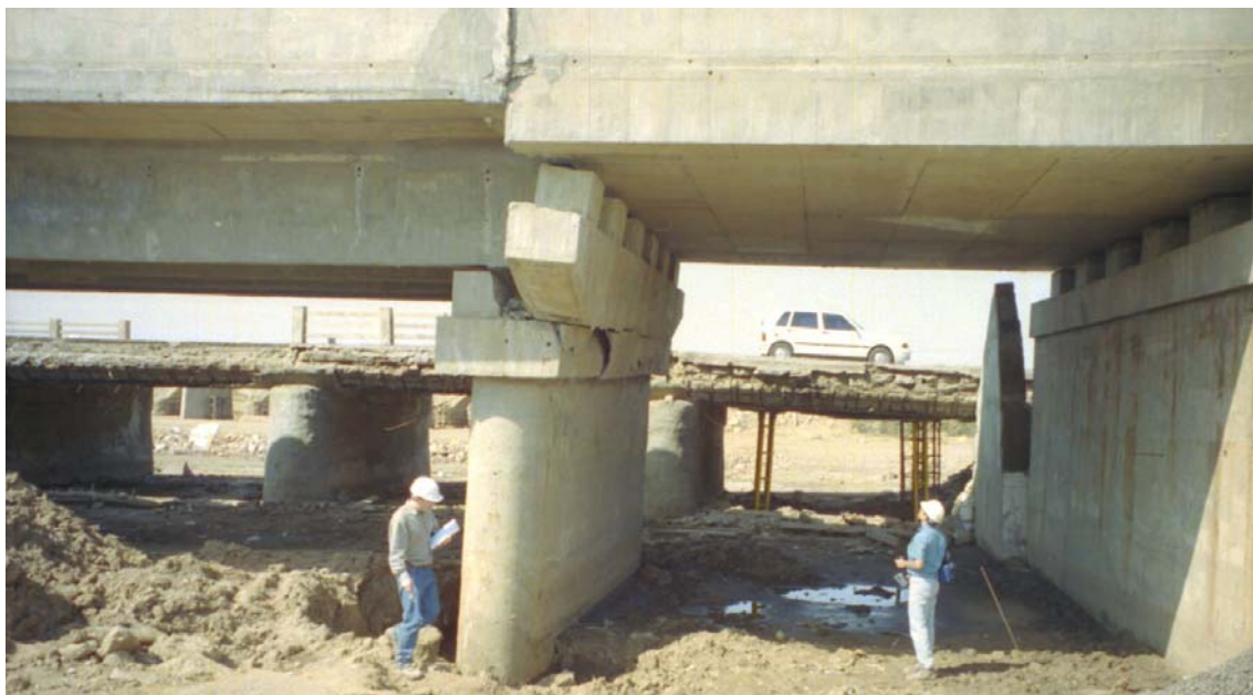
Figure 12 Four-Bridges Site on NH8A just to east of Bhachau – new (almost completed) road bridge: collision of deck with pier upstand, wing wall has moved forward relative to abutment, marks on pier and abutment show about 500mm settlement of soil
