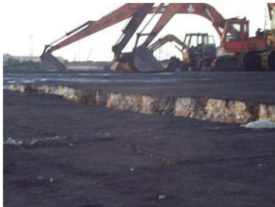
Figure 33 Settlement of backfill behind the jetties in Navalakhi port.
