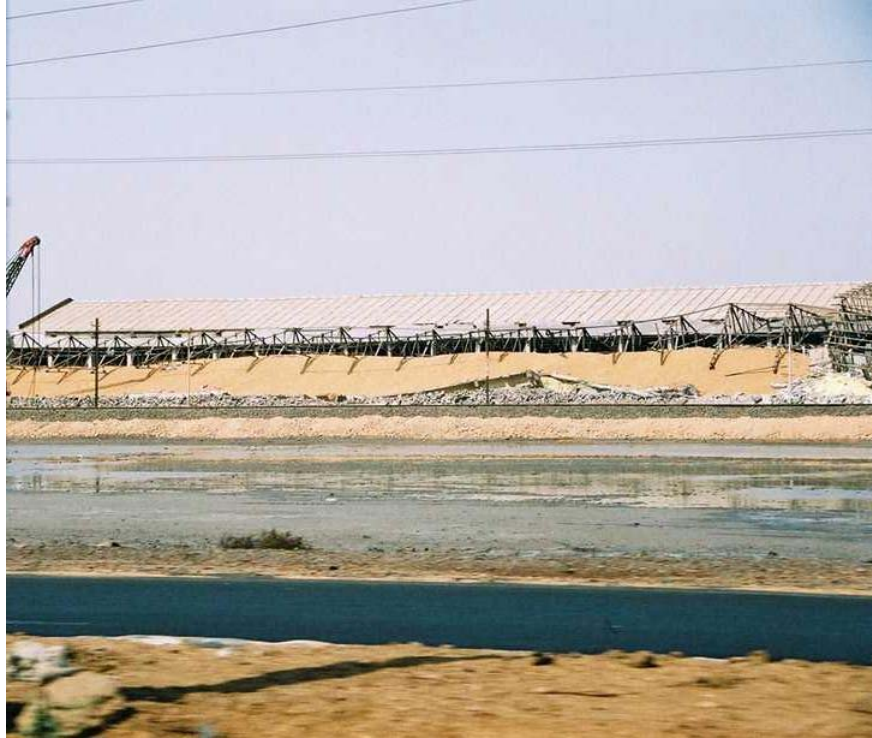
Figure 56 Collapse of Masonry Walled Bulk Material Warehouse, near Kandla
