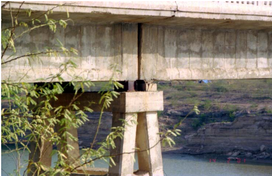
Figure 3 Rudramata (Khari) Bridge – fractured bearing plinth
