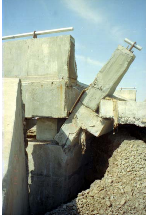
Figure 13 Four-Bridges Site on NH8A, new road bridge: east abutment had moved forward by about 500mm, ballast wall had collided with end of deck, and fill had settled
