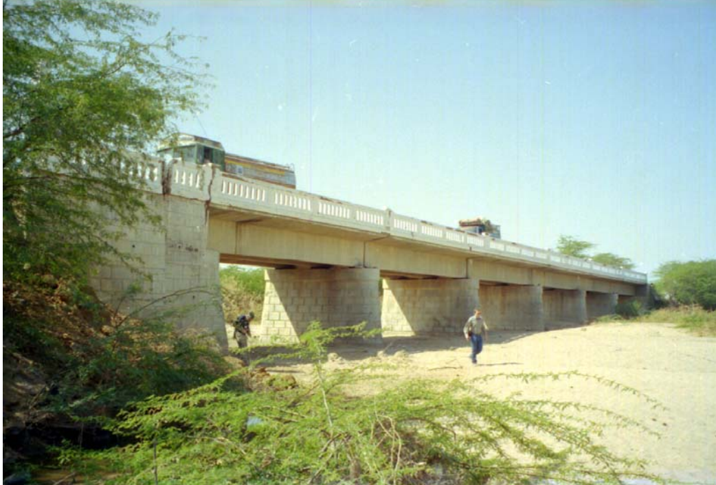
Figure 5 Six Span Bridge near Dudhai – oriented east-west, 25km from epicentre, probably constructed in the 1960s
