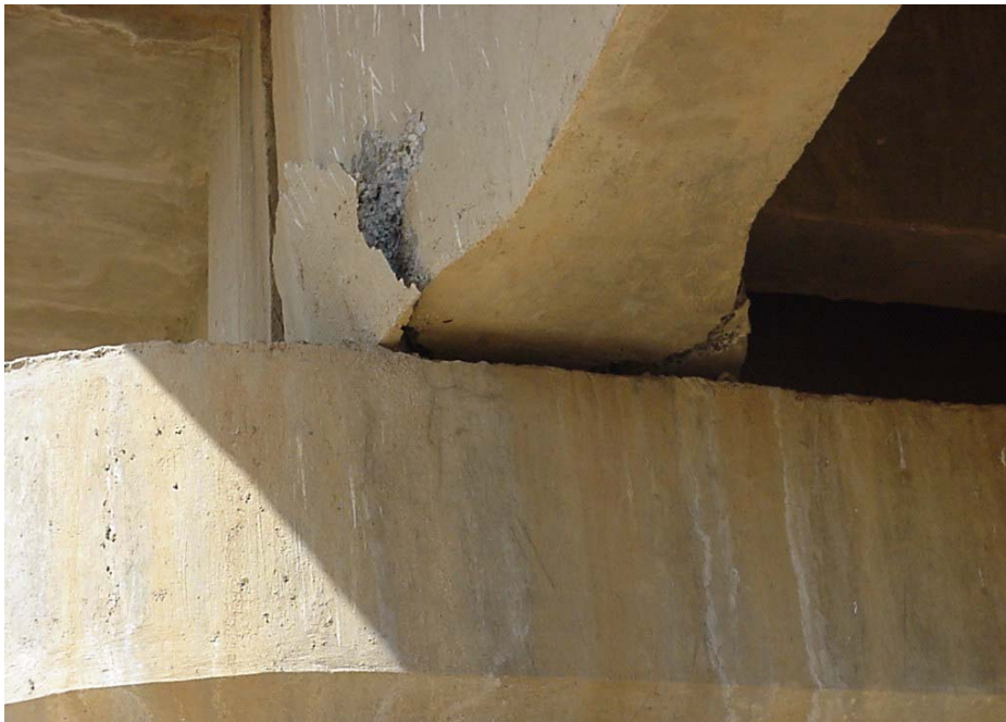
Figure 8 Six Span Bridge near Dudhai – damage to beams at bearings
