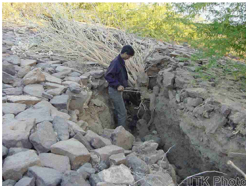
Figure 48 Deep cracks following the failure of the upstream slope [courtesy of IIT Kanpur]
