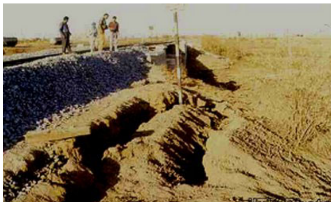
Figure 6 Lateral spreading of a railway embankment [courtesy of EERI]
