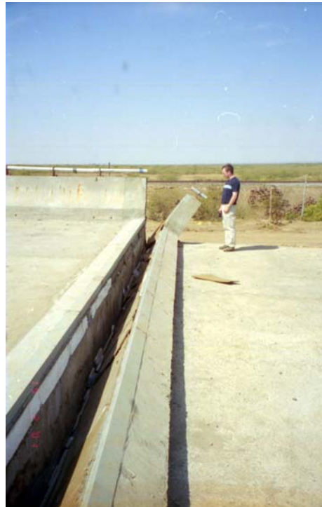
Figure 14 Four-Bridges Site on NH8A, new road bridge: tilted ballast wall
