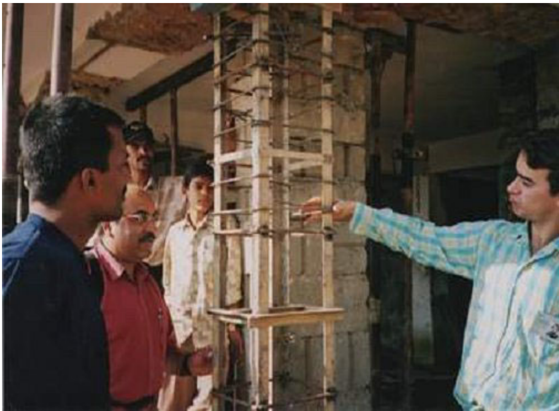
Figure 10 Repair works to damaged masonry building with RC floor. The new structural element has little connection with the existing structure.
