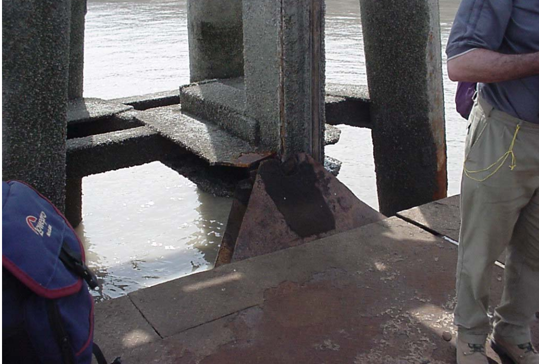
Figure 45 Kandla Port, launch jetty: pontoon guides were also damaged
