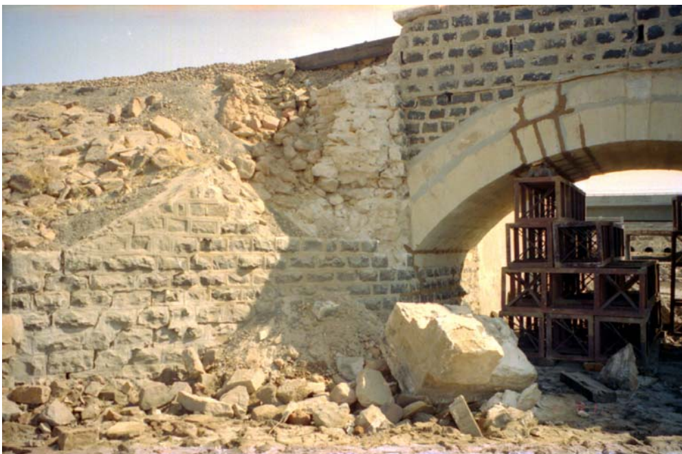
Figure 21 Four-Bridges Site on NH8A, metre gauge rail bridge: at east end of bridge masonry wing wall had been badly damaged and joints between arch blocks had been injected with epoxy
