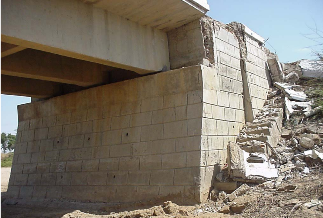
Figure 7 Six Span Bridge near Dudhai – settlement of the ground in front of the abutment, impact damage to ballast wall and loss of reinforced concrete parapet
