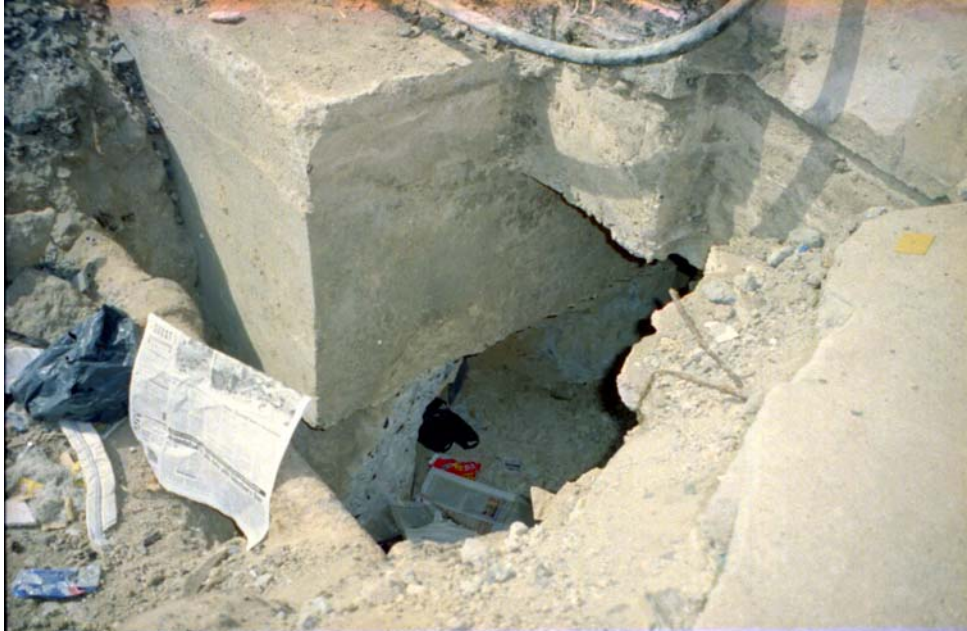
Figure 51 Kandla Port control tower: freshly spalled surface of corner pile indicated bending distress due to inertia loads and lateral spreading of underlying soil.
