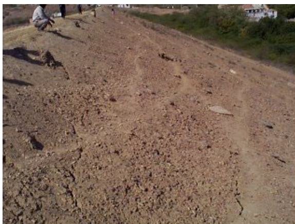
Figure 39 Longitudinal cracks on the downstream face
