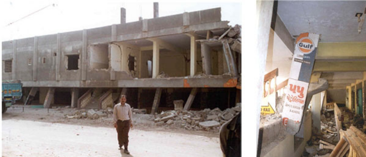
Figure 5 Soft storey failure in Gandhidham
