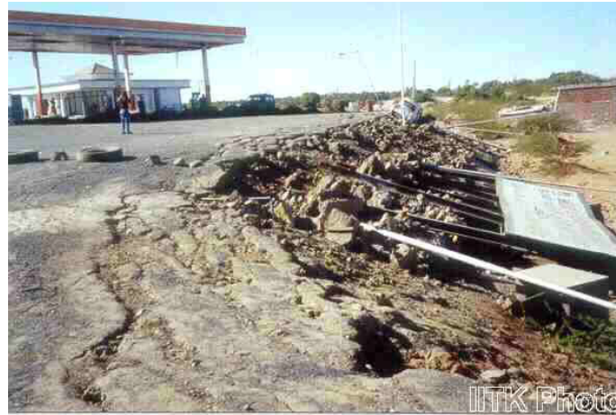
Figure 8 Lateral spreading resulting in damage to a filling station
