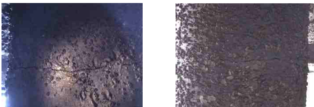
Figure 23 Cracks developed in some of the piles supporting the old jetties [courtesy of EERI]
