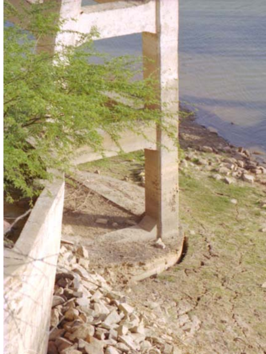
Figure 4 Rudramata (Khari) Bridge - settlement and lateral spreading of the soil, but caisson unaffected
