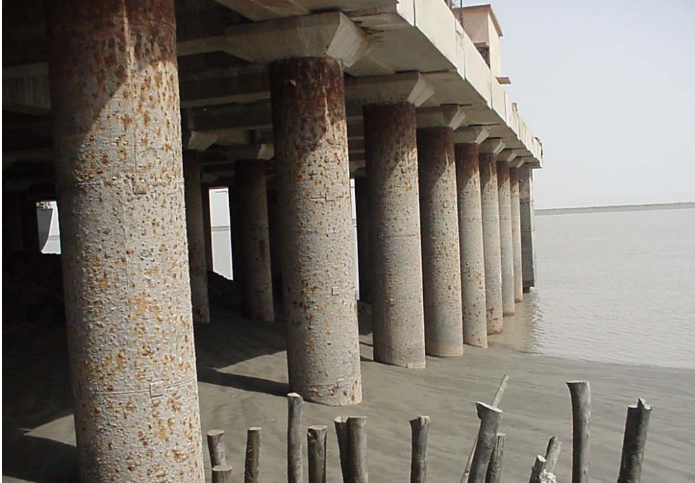
Figure 36 Kandla Port: new berth completed 4 - 5 years ago - 1000mm diameter reinforced concrete piles cast inside permanent steel casings. Structure appeared to have performed well with virtually no damage or displacement.
