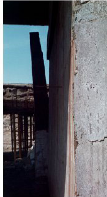
Figure 19 Failure of the abutment walls of the new highway bridge
