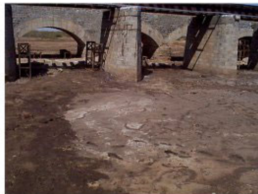
Figure 13 Extensive liquefaction at the pier bases
