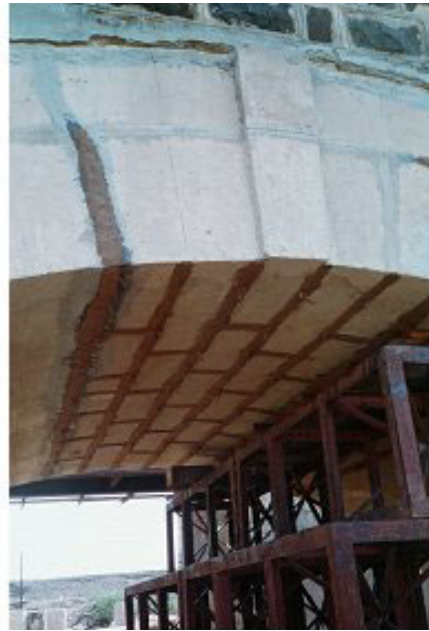
Figure 15 Damage to the crown blocks of the arch
