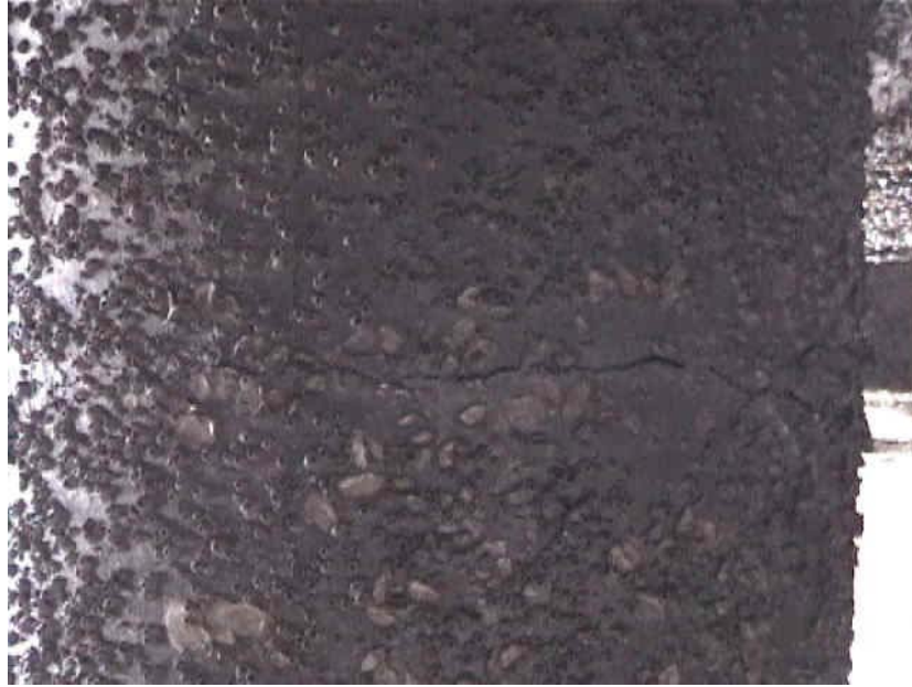
Figure 42 Kandla Port: a close-up of crack in 600mm diameter cylinder pile. [Photo courtesy of EERI].
