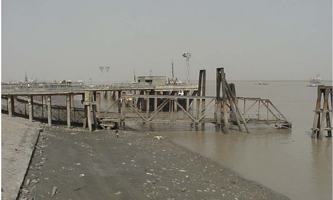
Figure 43 Kandla Port, launch jetty: steel truss dropped off its support ledge during a devastating cyclone which hit Kandla on 9 June 1998.
