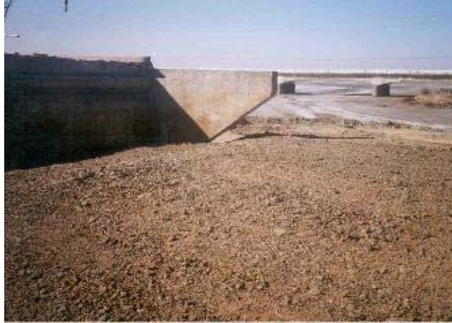
Figure 32 Surajbari New Bridge: liquefaction caused settlement of 1.3m behind the abutment at the Gandhidam end of the bridge. [Photo courtesy of Gammon India Ltd].
