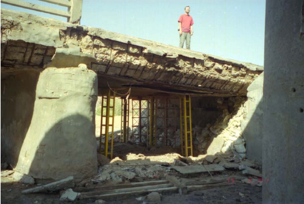
Figure 11 Four-Bridges Site on NH8A just to east of Bhachau – old road bridge showing badly deteriorated concrete, damage to east abutment, loss of sprayed concrete and parapet on ground. This bridge was carrying all the road traffic on the NH8A
