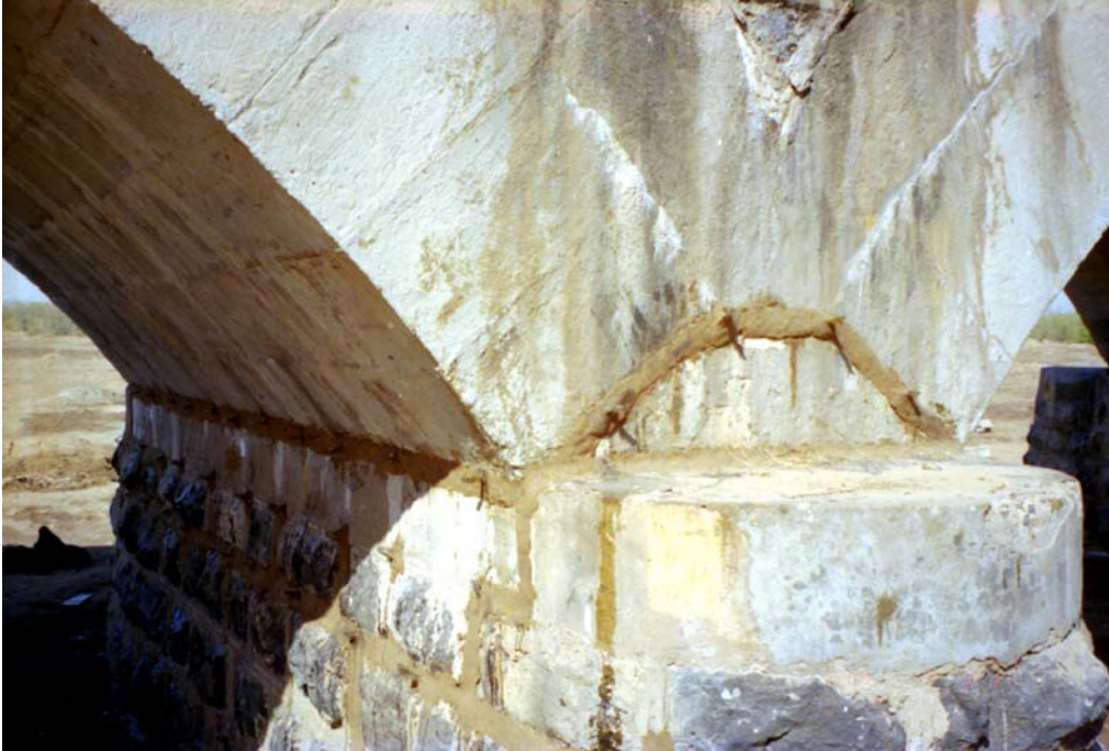
Figure 20 Four-Bridges Site on NH8A, metre gauge rail bridge: cracks between arch blocks had been injected with epoxy resin – note the surface sealing mortar and injection nipples
