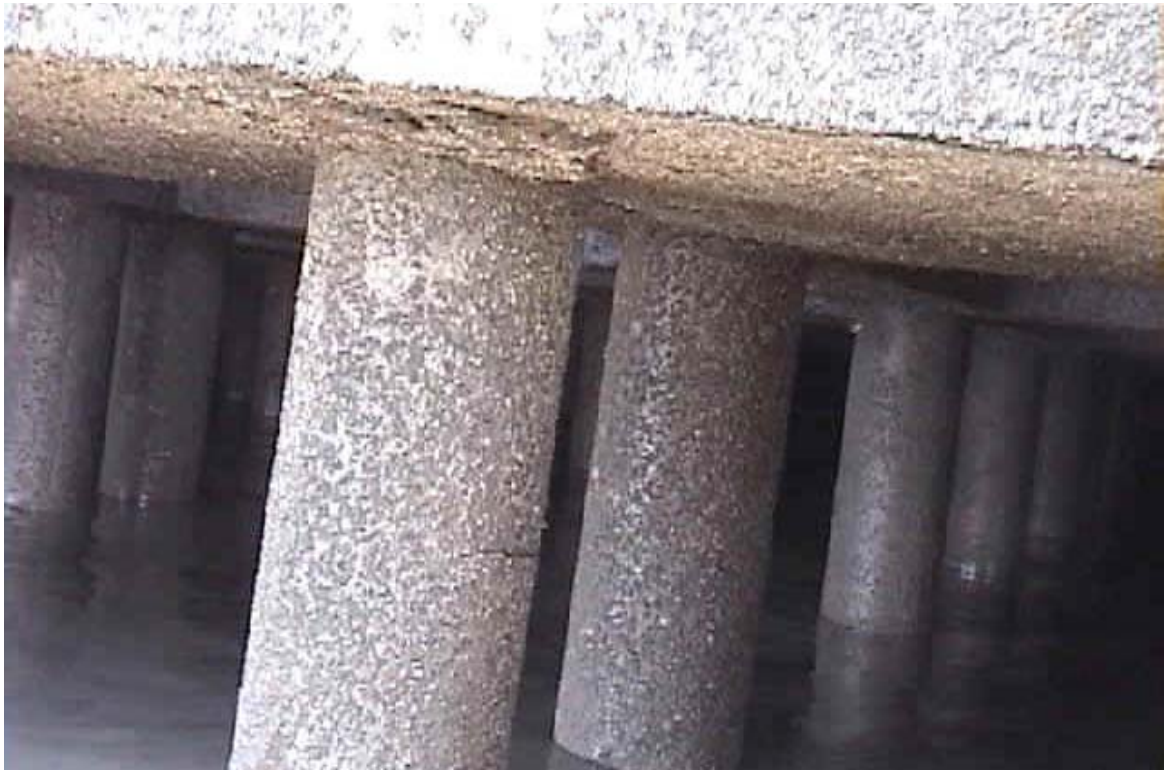
Figure 41 Kandla Port: 600mm diameter cylinder piles had cracked circumferentially about 300mm below their connection with the r.c. framing members. [Photo courtesy of EERI].
