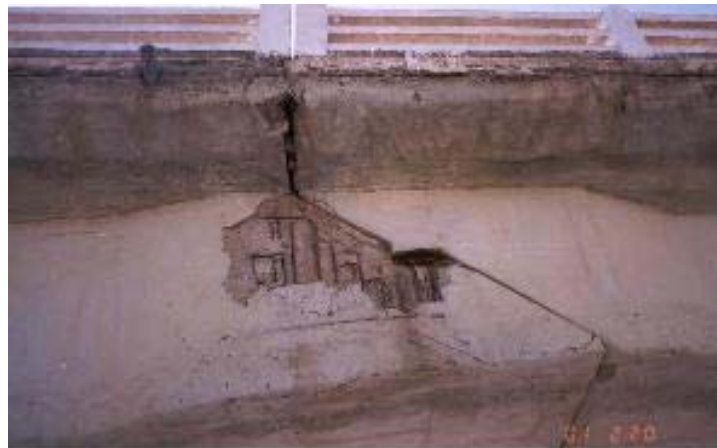
Figure 24 Surajbari Old Bridge: pounding at joint caused spalling of concrete coating and cover. Note severely corroded reinforcement. [Photo courtesy of Mahesh Tandon].
