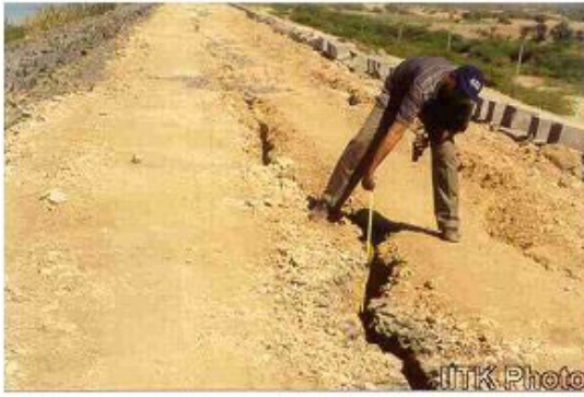
Figure 44 Longitudinal cracks extending to the core
