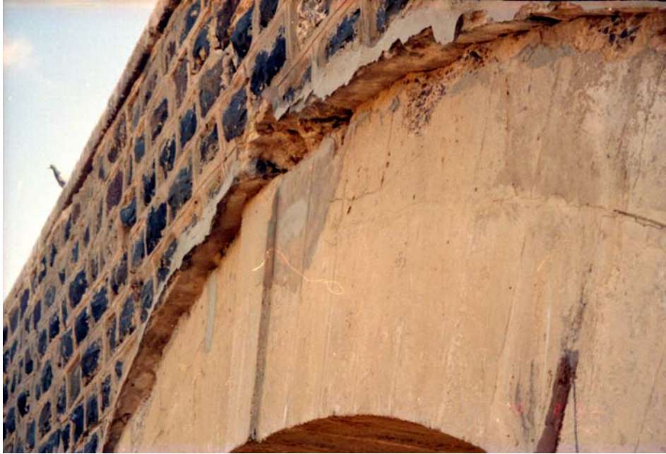
Figure 18 Four-Bridges Site on NH8A, metre gauge rail bridge: bulging of spandrel wall on north side of bridge
