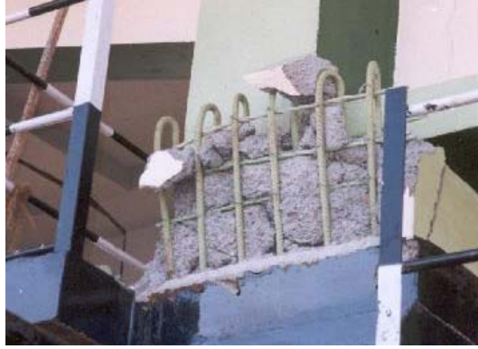
Figure 29 Surajbari New Bridge: damage to shear stopper block. [Photo courtesy of Mahesh Tandon].
