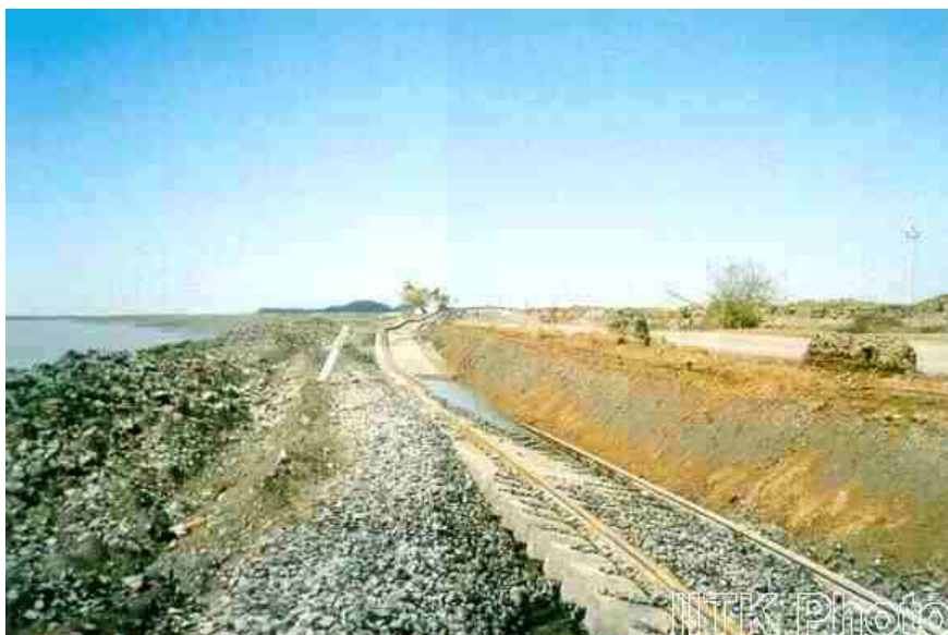
Figure 35 Damage to the railway line feeding Navalakhi port [courtesy of IIT Kanpur]
