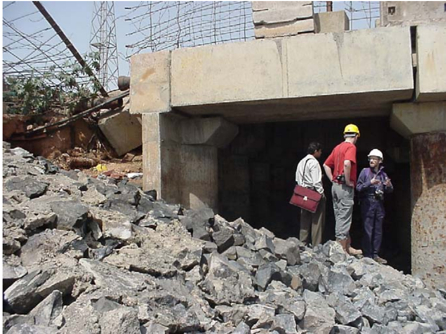
Figure 37 Kandla Port new berth: retaining wall cast integral with landward edge row of piles. Material had been lost at this free corner due to settlement and lateral spreading. See also Figure 39.
