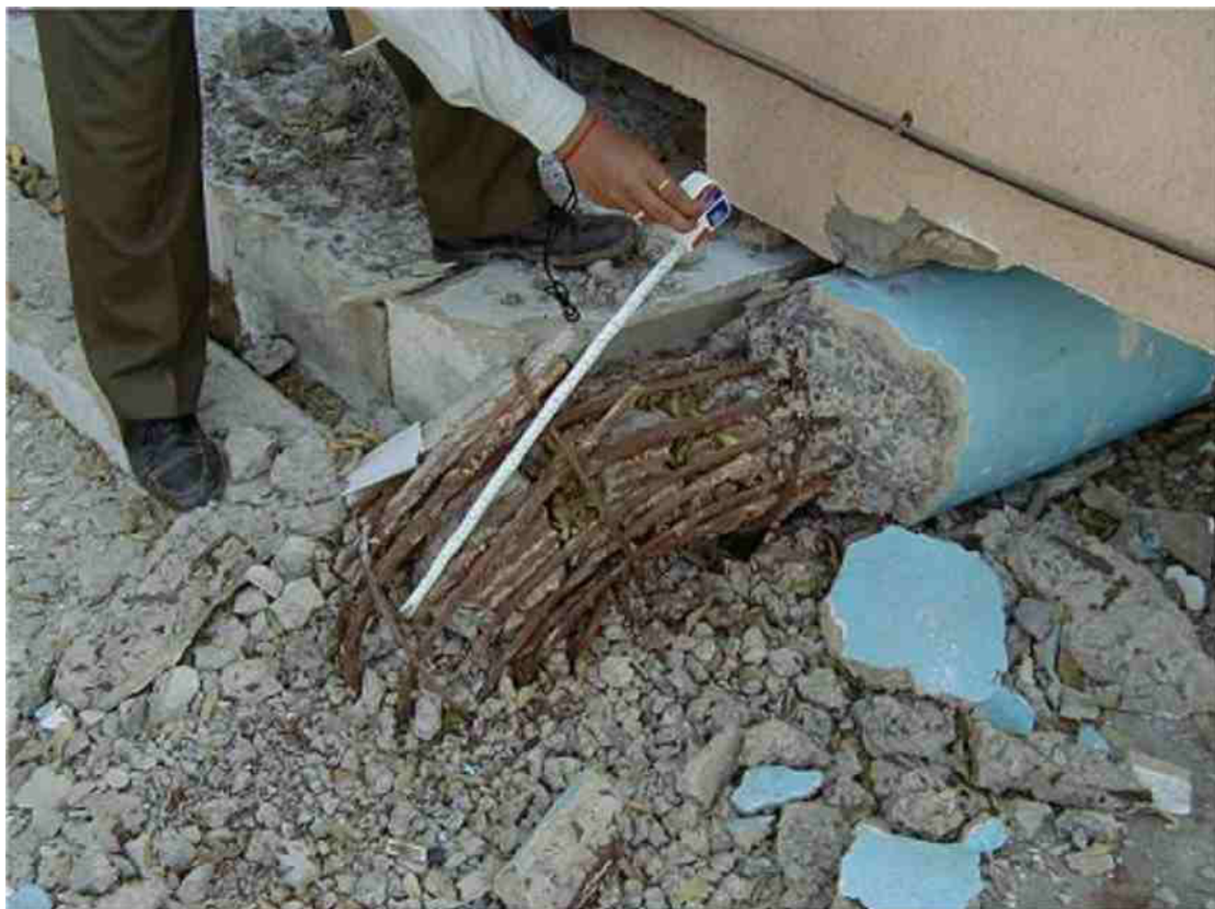
Figure 13 Poor detailing at Kandla Port
