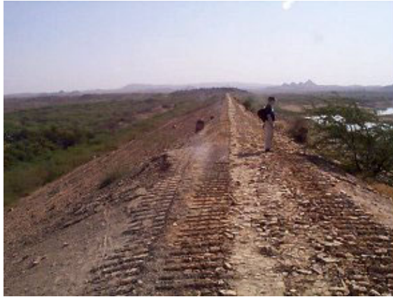
Figure 41 Settlement of the crest
