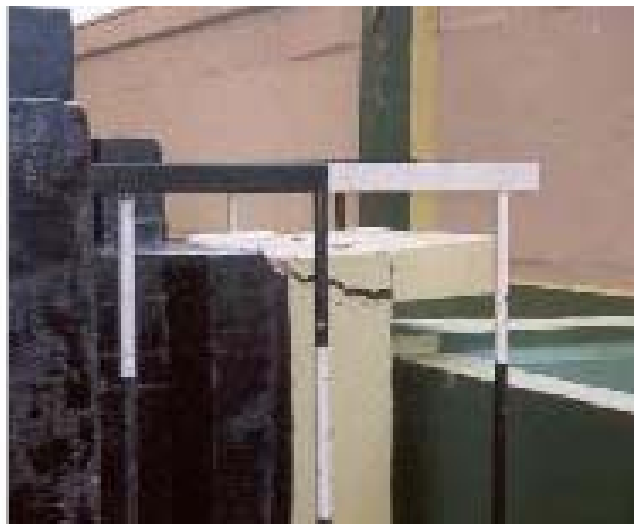
Figure 28 Surajbari New Bridge: many shear stopper blocks were badly damaged. [Photo courtesy of Mahesh Tandon].
