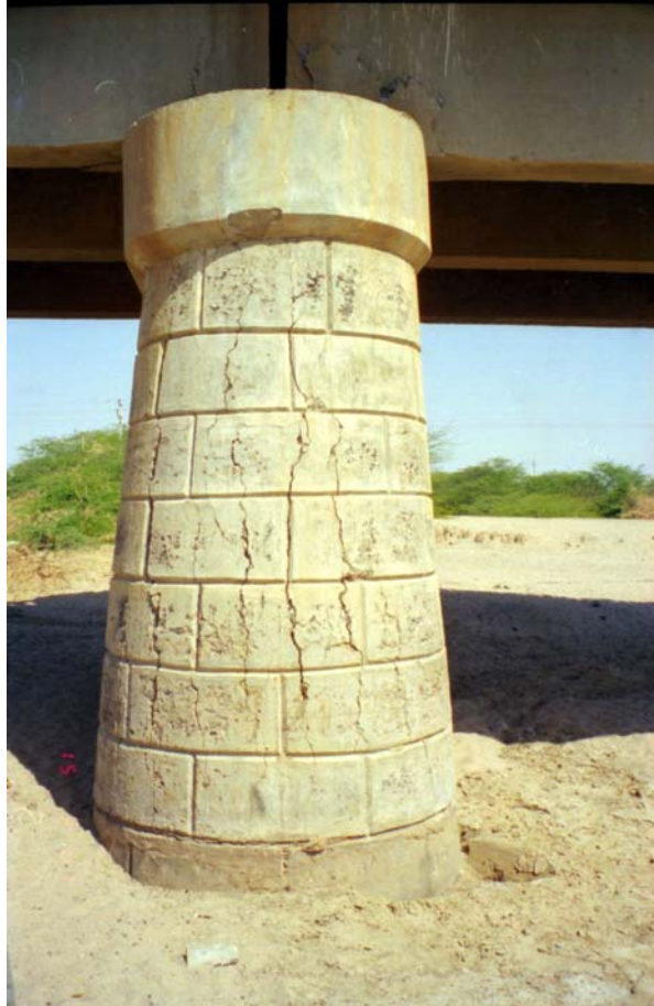
Figure 9 Six Span Bridge near Dudhai – vertical cracks in ends of piers probably due to reinforcement corrosion possibly made worse by splitting forces from corroded and locked up bearings
