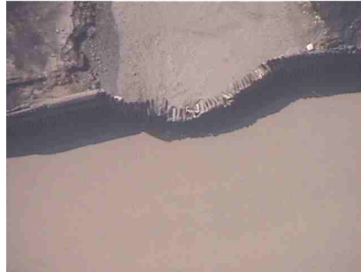
Figure 31 Failure of a sheet pile wall
