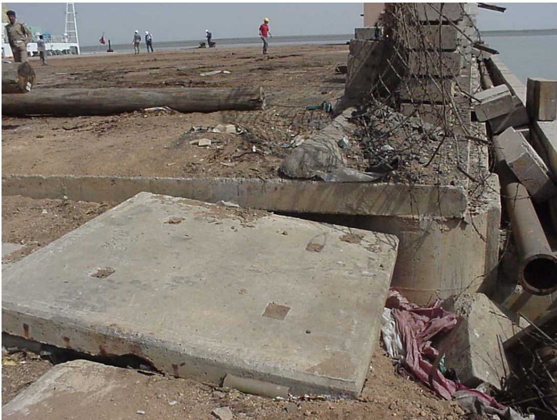
Figure 39 Kandla Port new berth: loss of material at end of new berth
