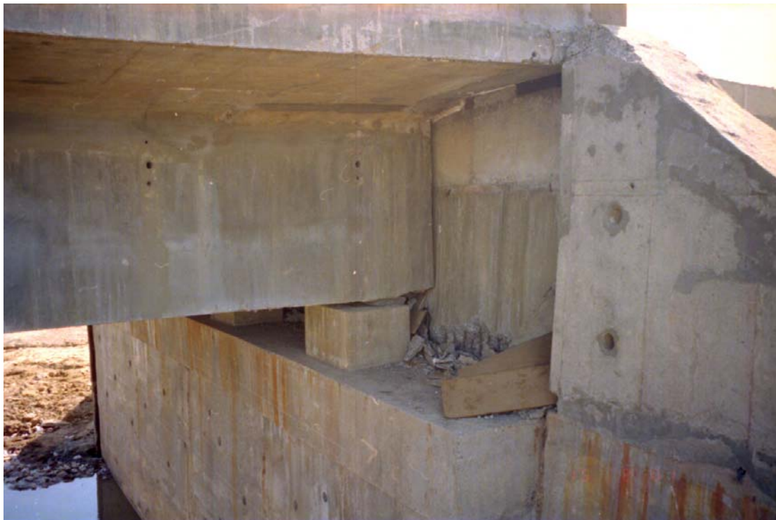
Figure 16 Four-Bridges Site on NH8A, new road bridge: the west abutment had moved forward by about 200mm and ballast wall had also been damaged, but not as severely as at the east end abutment
