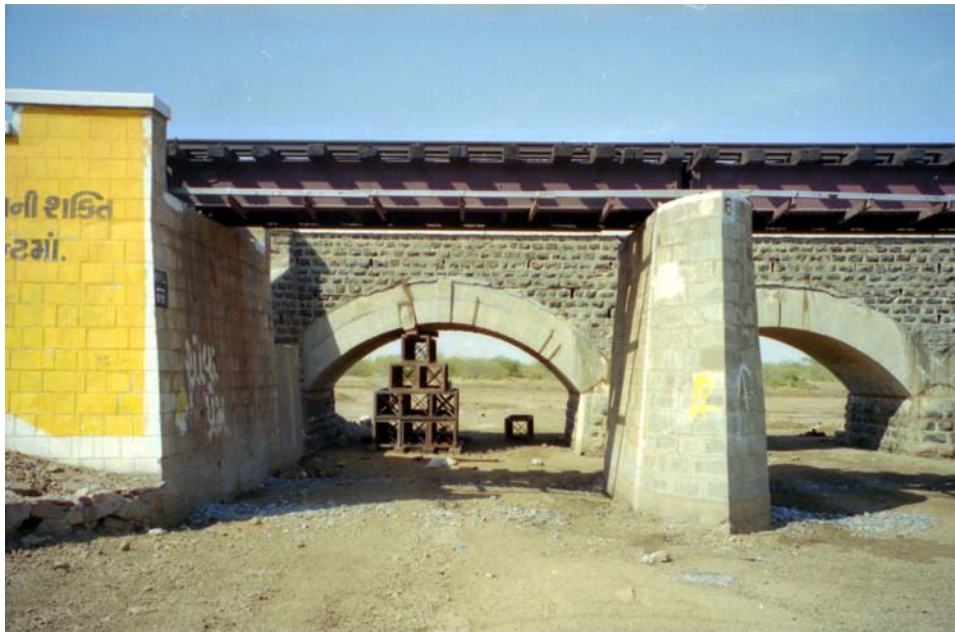
Figure 19 Four-Bridges Site on NH8A, metre gauge and broad gauge rail bridges: joints between loosened arch blocks had been epoxy injected in west end span. Note it had not been possible to jack blocks back into original position
