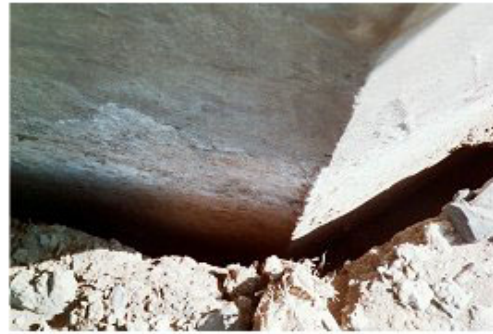
Figure 21 Large gap opened between the pier and soil
