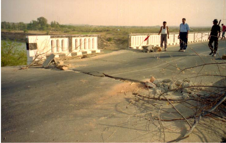
Figure 2 Rudramata (Khari) Bridge – settlement behind north abutment and missing section of parapet
