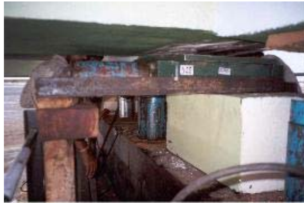
Figure 33 Surajbari New Bridge: decks had been displaced up to a maximum of 250mm. After jacking a Hillman roller assembly was used to move the deck back to its correct position. [Photo courtesy of Mahesh Tandon].
