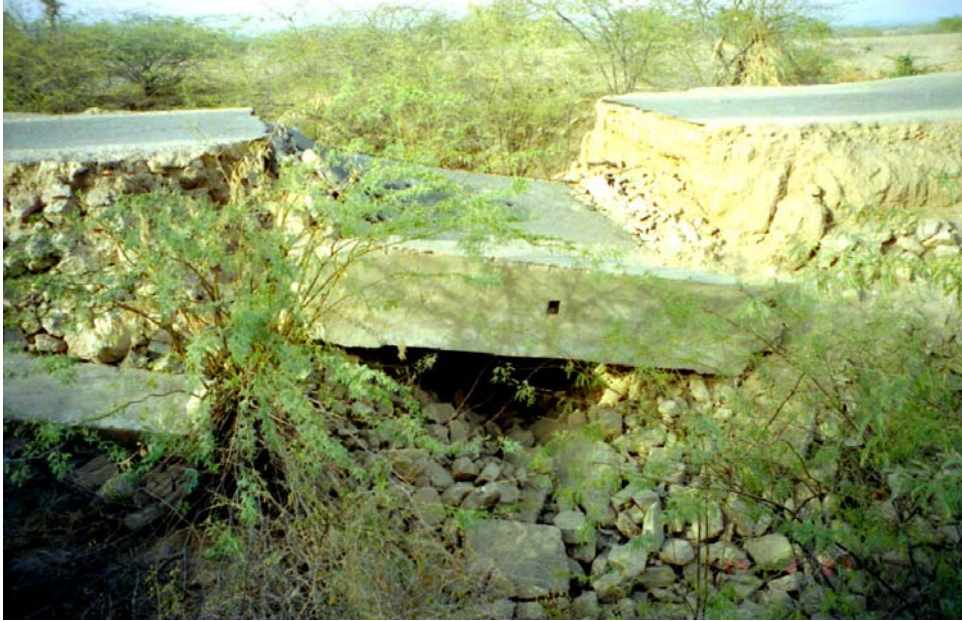
Figure 34 Small reinforced concrete slab bridge on road from Bhuj to Lodai: masonry abutments were destroyed by violence of shaking
