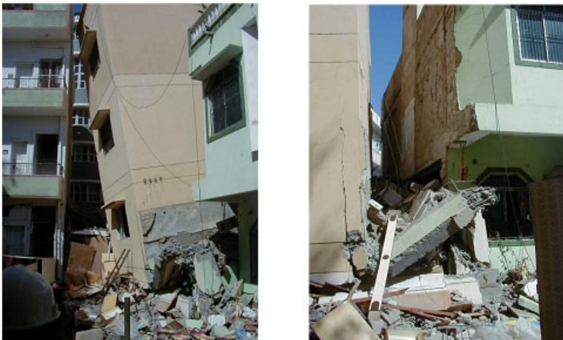
Figure 7 Soft/weak storey collapse in Bhuj
