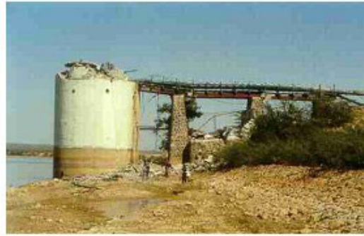
Figure 45 Severe damage to the intake tower
