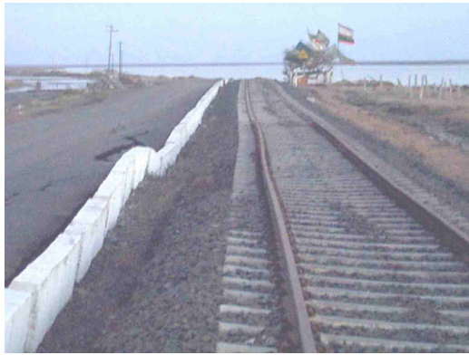
Figure 36 Sudden change in ground elevation along the track
