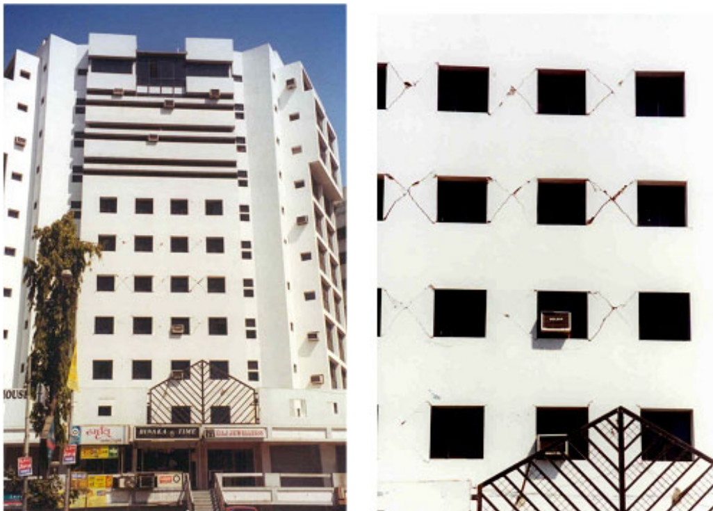
Figure 16 Diagonal cracking in Ahmedabad
