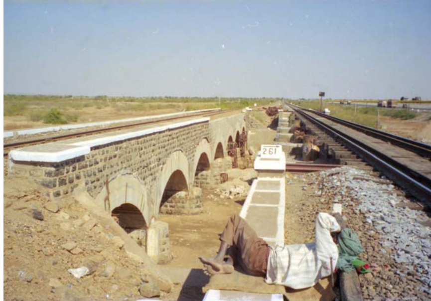
Figure 17 Four-Bridges Site on NH8A, metre gauge and broad gauge rail bridges: masonry arches support metre gauge, and steel girders support broad gauge. Spandrel wall had collapsed and been reconstructed where white coping stones are missing. Note bulges at crown of arches on this south face.
