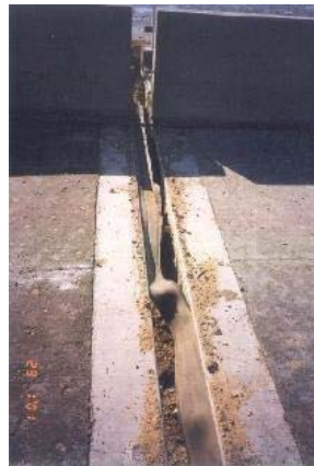
Figure 30 Surajbari New Bridge: deck joints were moved beyond their capacity and some rubber seals were torn out. [Photo courtesy of Mahesh Tandon].
