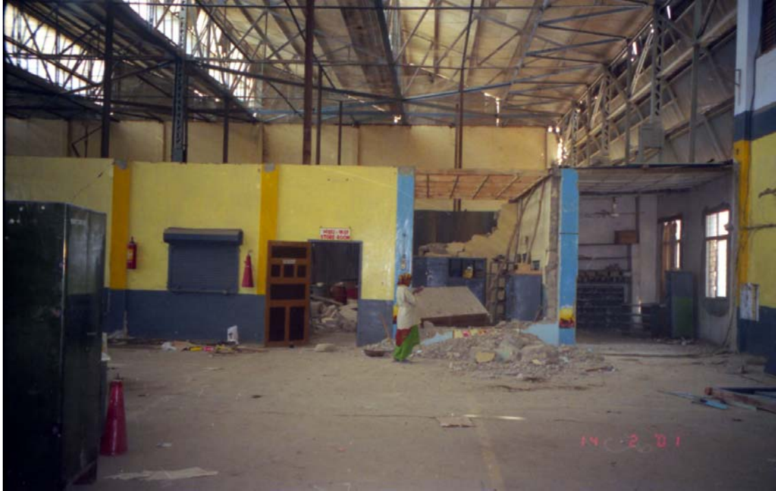
Figure 54 Kandla Port: some masonry partition walls had collapsed in the workshops
