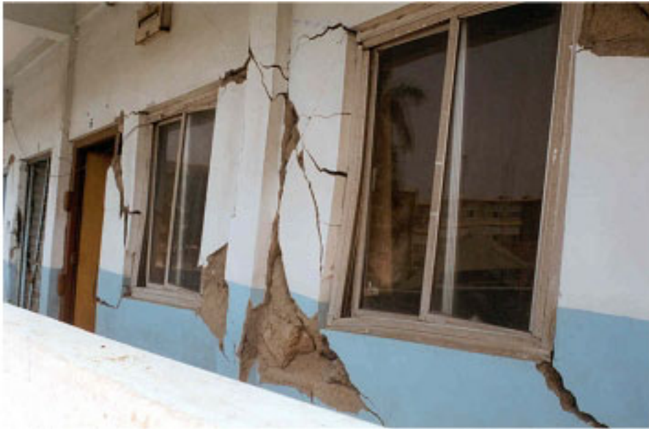
Figure 17 Heavily cracked building at Kandla Port
