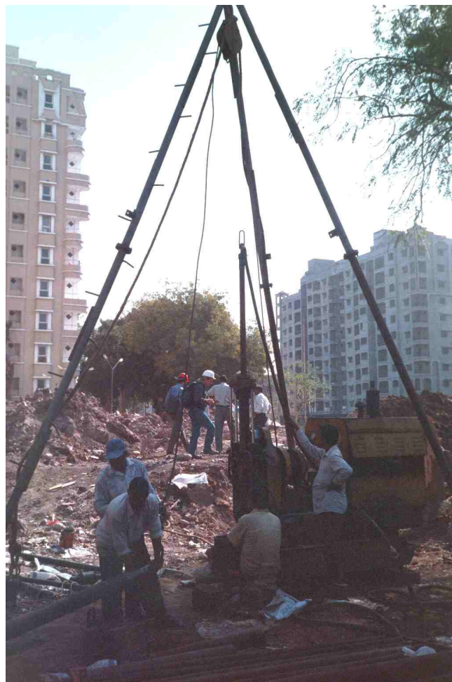
Figure 2 Soil testing at the site of a collapsed building
