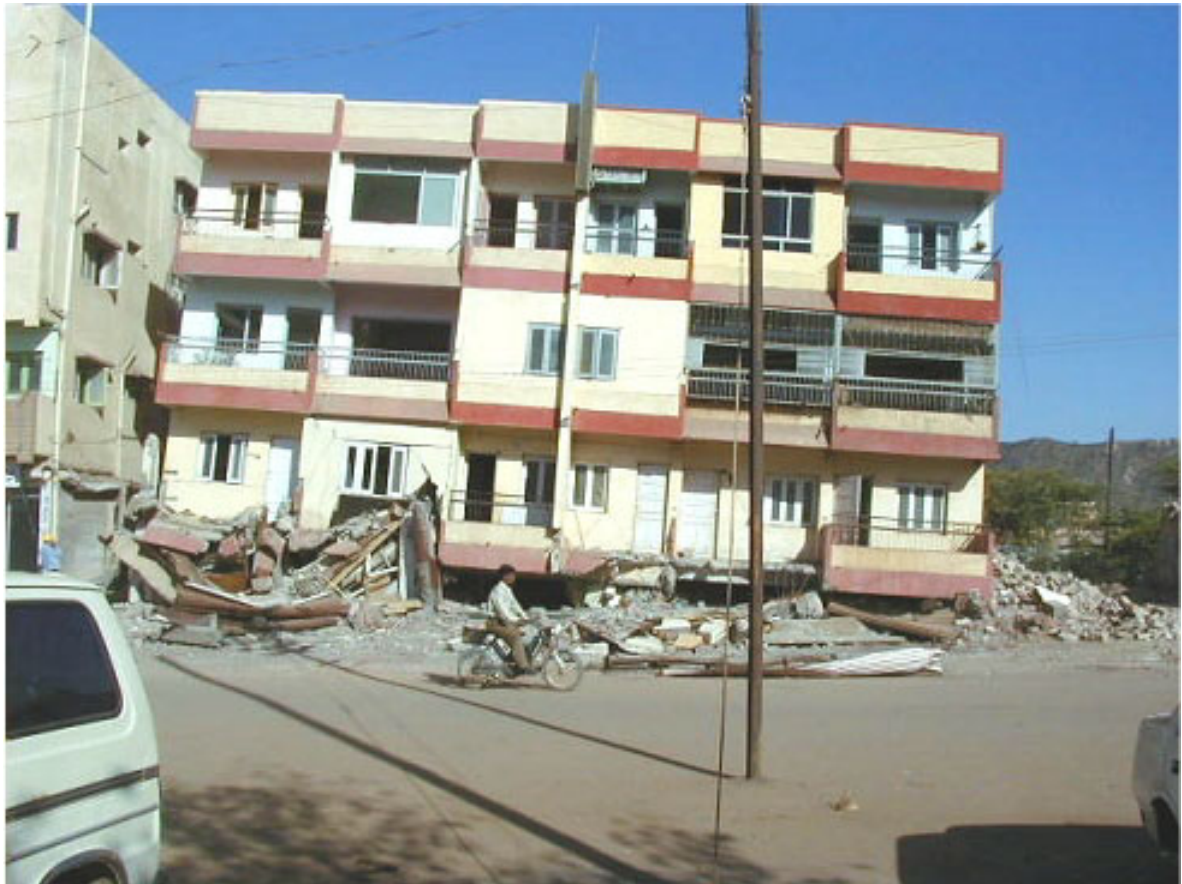
Figure 1 Typical soft storey collapse in Bhuj
