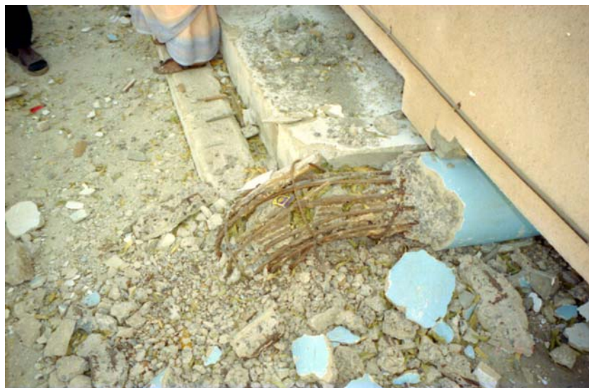
Figure 49 Kandla Port, 2-storey building: laps in maximum moment zone and virtually no confining reinforcement – a fatal combination
