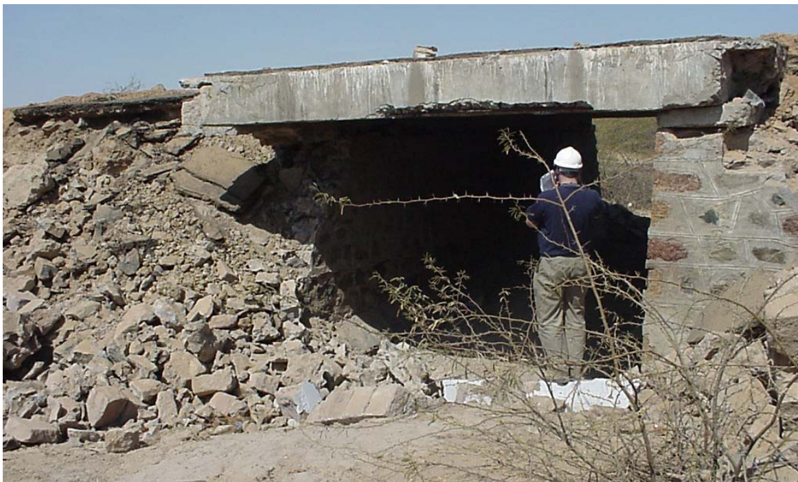
Figure 35 Small reinforced concrete slab bridge structure 10km west of Bhachau at Sikara. East-west orientation and earthquake had shifted the deck southwards
