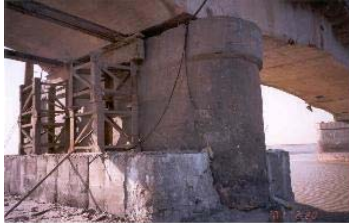
Figure 23 Surajbari Old Bridge: Pier 12 tilted longitudinally and had to be strengthened before re-opening to traffic
