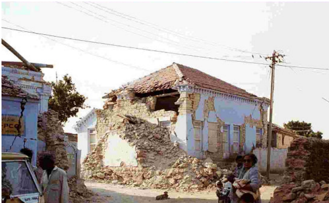
Figure 2 Typical coursed stone with timber floor Type B dwelling where poor tying in of roof has caused upper wall overturning.
