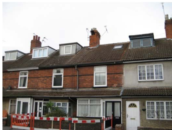
Figure 3: Detail of damage observed to Chimneys at Gainsborough (top). Please note that damage was not widespread (bottom) but localized on individual houses.
