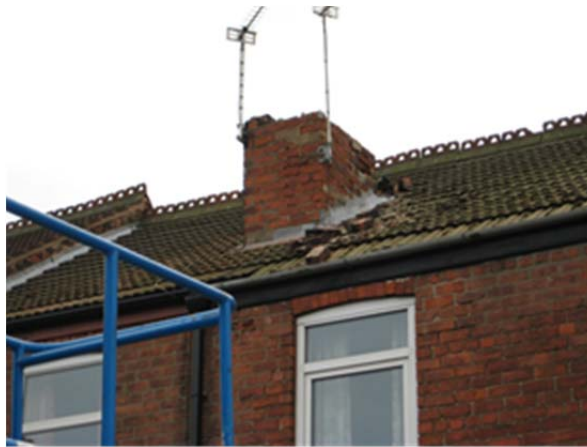
Figure 2: Typical damage observed to Chimneys. Photo taken at Gainsborough
