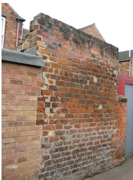
Figure 4: Damage on party wall at Gainsborough
