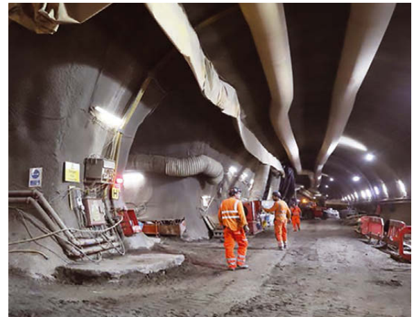
↑ FIGURE 4: Trust of affected companies was key when tunnelling beneath Grade 1 and Grade 2 listed buildings for Bank station upgrade project in London
