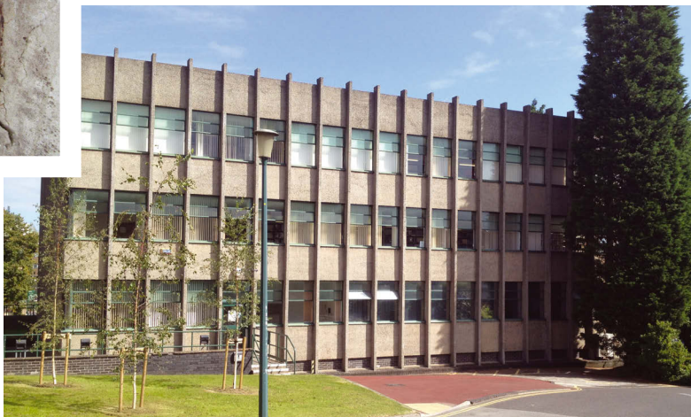
FIGURE 6: Major structural defects were uncovered at George Green Library, University of Nottingham
