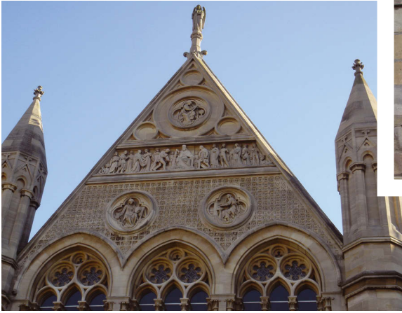
FIGURE 5: Grade II* listed Arkwright Building at Nottingham Trent University, with significant historical movement due to settlement
