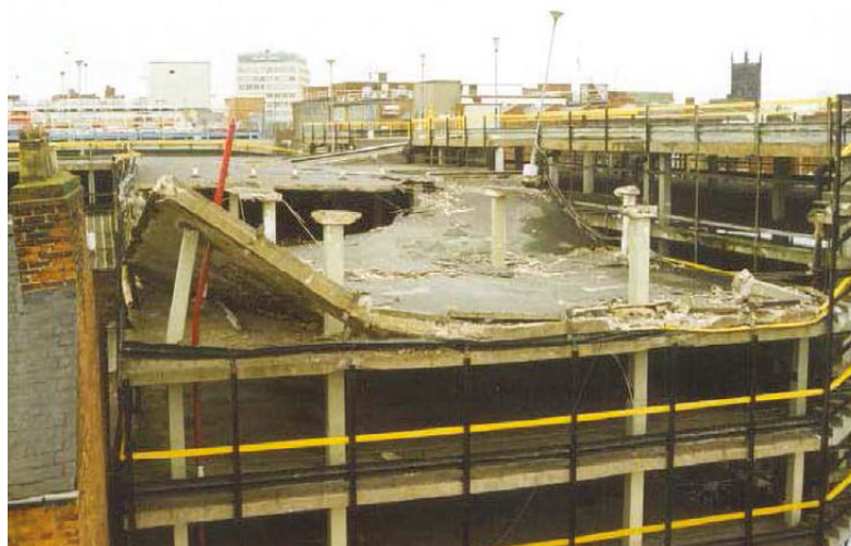
FIGURE 1: It is preferable to avoid sudden failure, such as that of the Pipers Row car park in Wolverhampton in 1997
