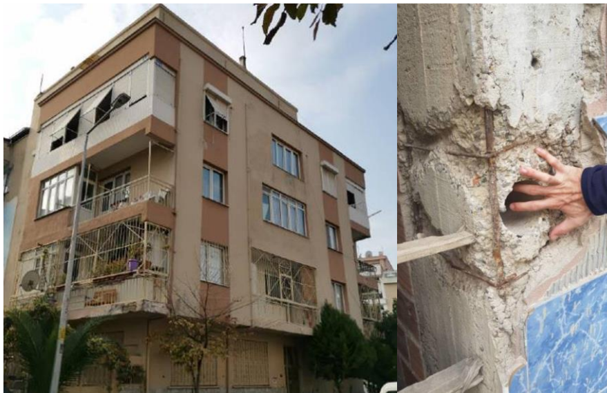
Figure 81: Degradation in structural material and poor detailing in an RC element
