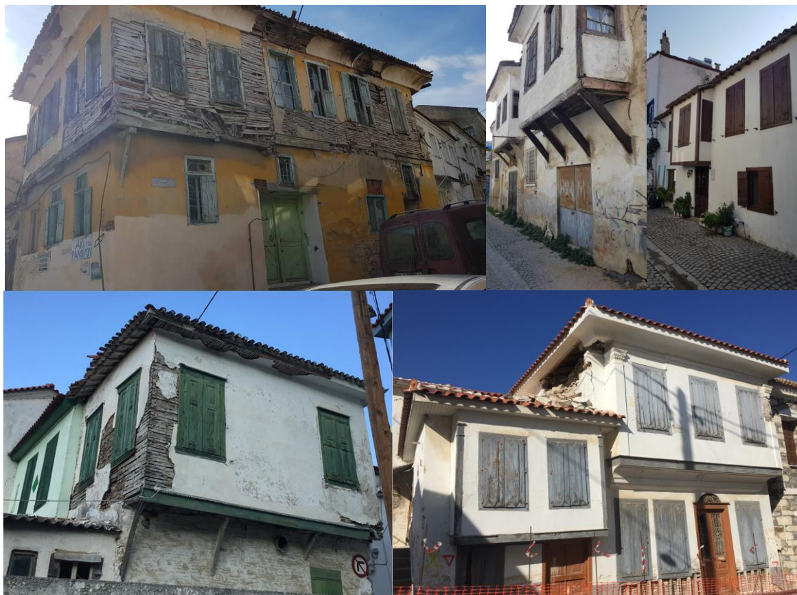
Figure 93: Some examples of hımiş structures in the affected areas (top row) in Turkey and (bottom row) in Samos
