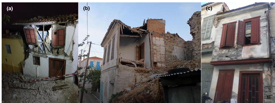
Figure 94: Examples to damage in hımiş structures
