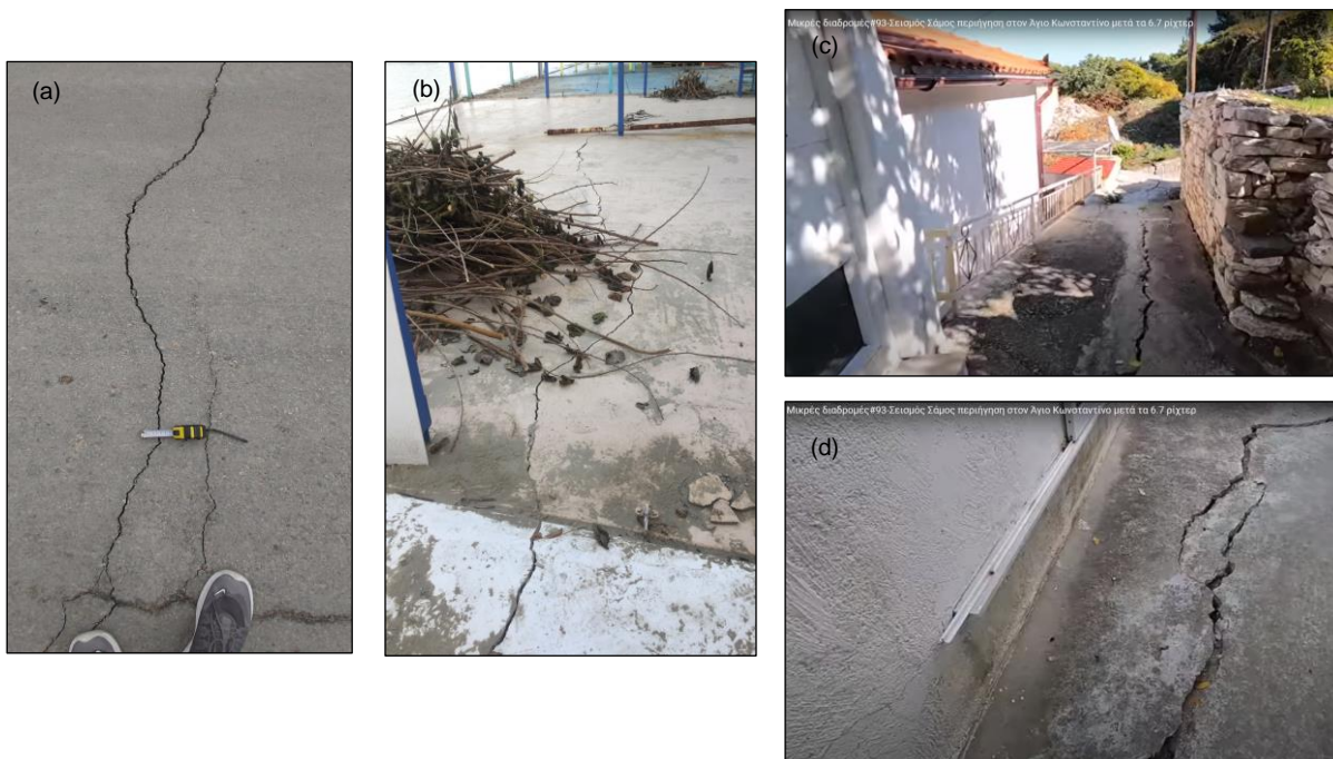
Figure 34: The observed ground cracks in a) Karlovasi, b) Kokkari and c) and d) at the village of Agios Konstantinos (source: https://www.youtube.com/watch?v=E5lv20MwagI&t=1s )
