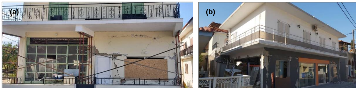
Figure 60: Damage to infill walls in two RC buildings in Samos: (a) in plane and (b) out of plane failure
