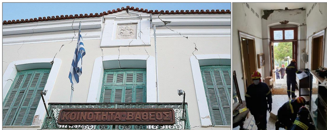
Figure 73: Severely damaged historical building of the town hall of Vathy (photo credit: Facebook page - Kathimerini)
