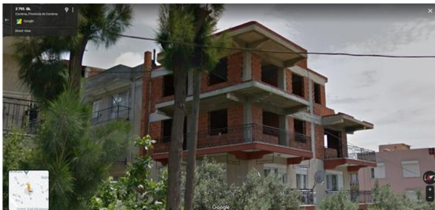
Figure 76: Street view from Izmir – reinforced concrete first and second extension under construction
