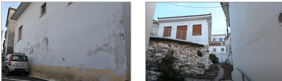
Figure 64: Damage in masonry buildings in Samos with horizontal cracks at floor level due to sliding (Photo credits to "Mikres diadromes" youtube channel)
