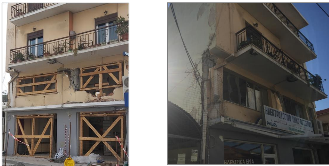
Figure 62: Four-storey building with short column failure in Samos
