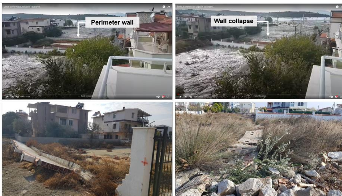
Figure 106: Perimeter wall overturning due to tsunami hydrodynamic effects in Sığacık (coordinates: 38.1982930, 26.7902697). Video frames (on top) from YouTube video: https://youtu.be/n93puRYKhs0
