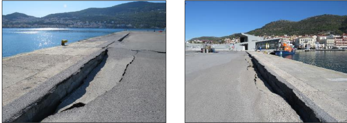
Figure 44: Significant damage was observed on Vathy ports of Samos (Lekkas et al., 2020)
