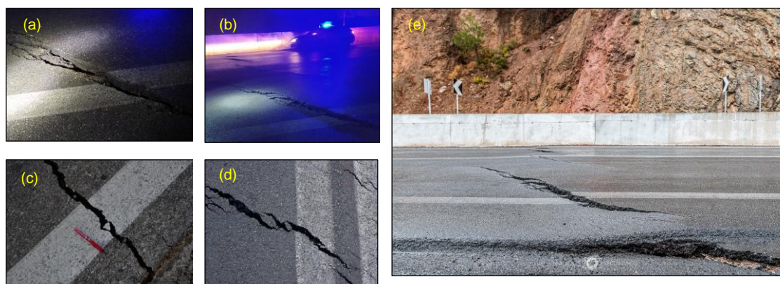
Figure 35: Road cracks observed in the area of (a) Vathy-Karlovasi road (Vadaloukas et al., 2020), (b, c) Agios Nikolaos (Lekkas et al. 2020), and (d) the main road Vathy-Karlovasi close to Karlovasi (photo taken by Manolis Thravalos)
