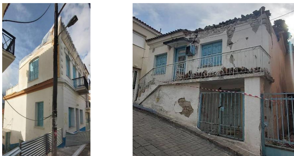
Figure 65: Roof damage to masonry buildings in Samos.
