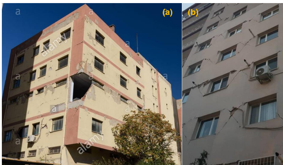
Figure 82: Infill walls damage in RC frames: (a) out of plane (Arda Savaşcioğulları / Alamy Stock Photo) and (b) in-plane failure
