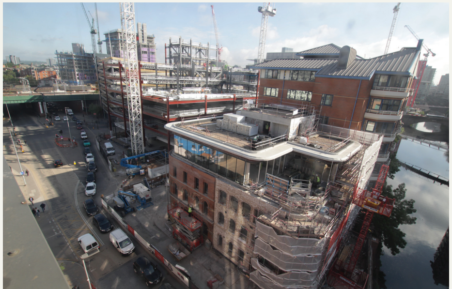
FIGURE 5: One and Two New Bailey, London – Farrat thermal breaks used to achieve BREEAM Excellent rating
