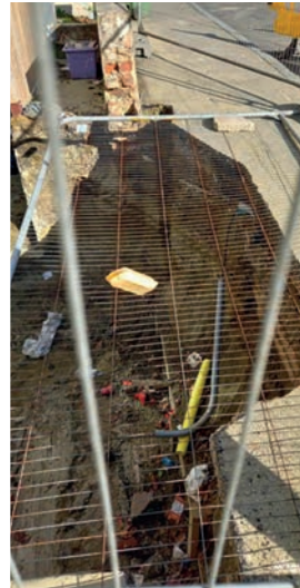
FIGURE 2: Footpath collapse due to unsupported excavation
