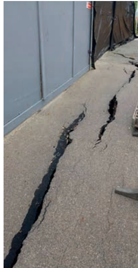
FIGURE 1: Cracking to top surface of footpath adjacent to excavation
