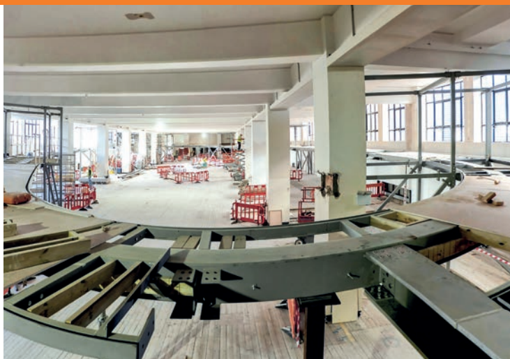
FIGURE 1: An early highlight was designing a steel-and-timber walkway for London's Science Museum
