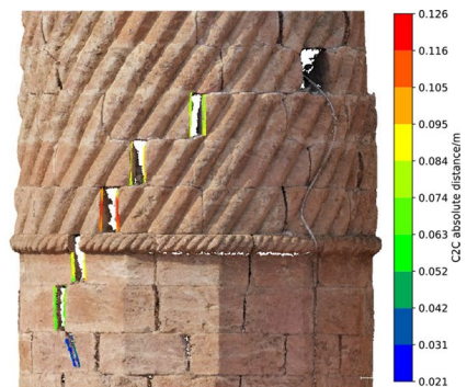
(b) Crack measurements.
