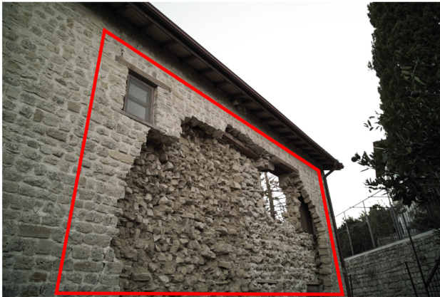
(d) Later photograph showing collapse of the bulging area in N wall
