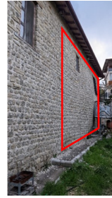
(b) Photograph of bulging in N wall.
