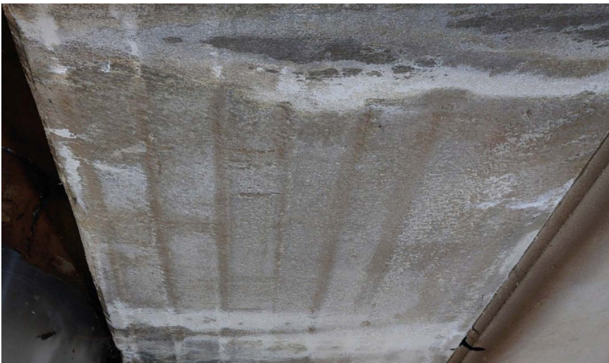
Appendix 1 – 13 Water ingress: Rebar ghosting/shadowing evidencing water ingress
