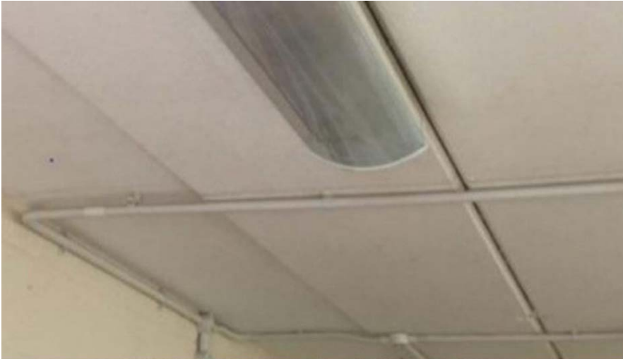
Appendix 1 – 14 Panels stepped down below adjacent panels
