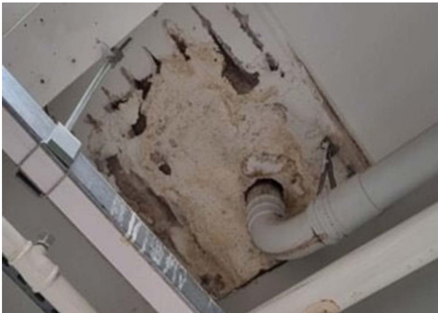
Appendix 1 – 3 Builderswork panel holed for downpipe – spalling, corroded longitudinal and transverse cut bars
