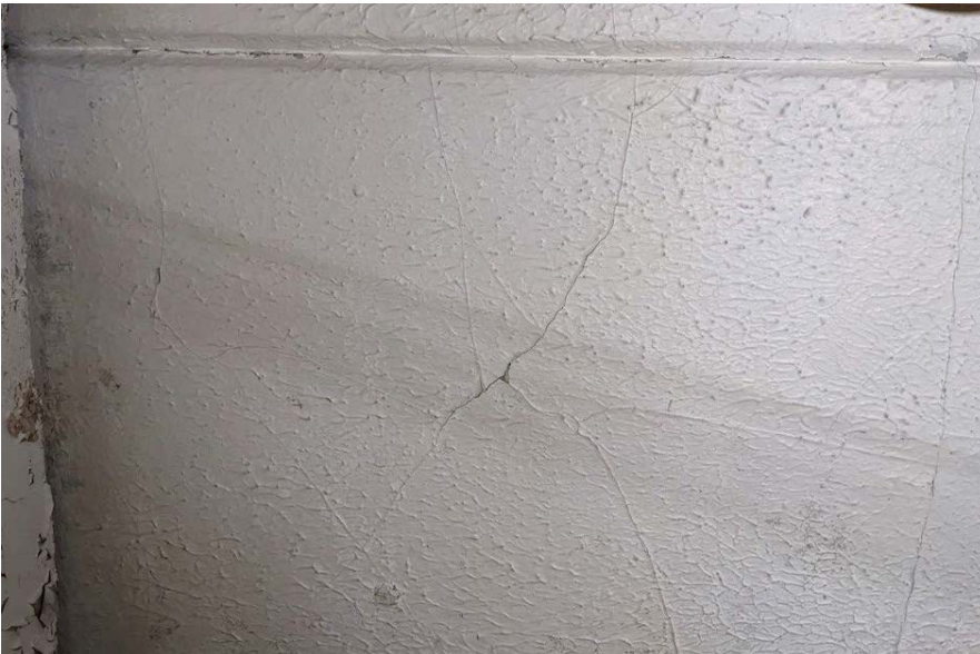
Appendix 1 – 7 Cracking: crazing panel cracks within 500mm of bearing - visible through 'artex' type coating.
