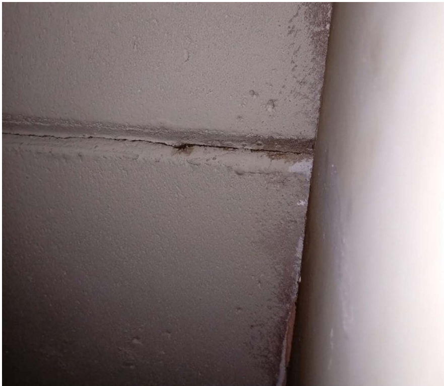
Appendix 1 – 9 Minor longitudinal cracking between panels. By itself not usually a significant concern
