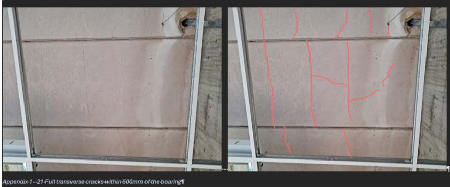
Appendix 1 – 8 Full transverse panel cracks within 500mm of the bearing
