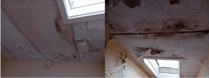
Appendix 1 – 10,11 Severe water ingress: Damage at Skylight location
