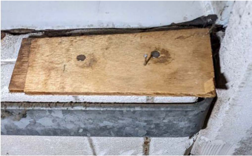
Appendix 1 – 6 Exposed steel trimming strap supporting cut panel
