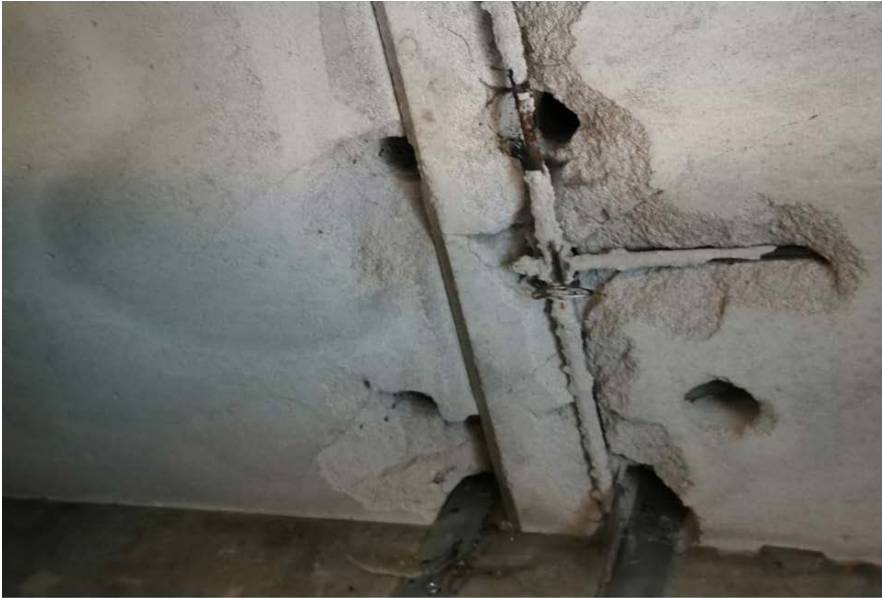
Appendix 1 – 4 Builderswork has caused spalling of panel face exposing rebar
