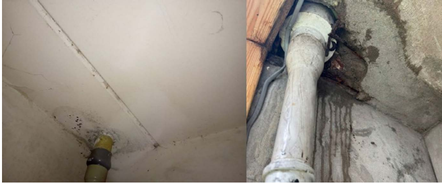
Appendix 1 – 1,2 Builderswork - panel holed for downpipe, with evidence of water ingress
