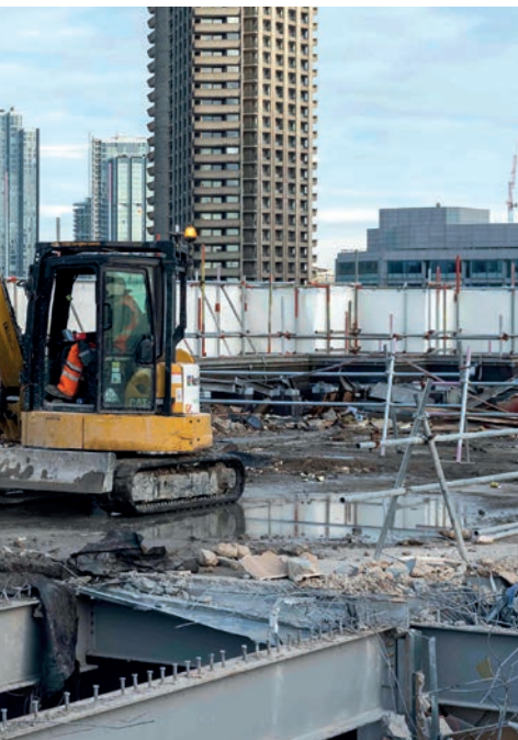
FIGURE 1: At City Place House, Howarth had site role overseeing steel recovery, with large proportion subsequently reused at 30 Duke Street
