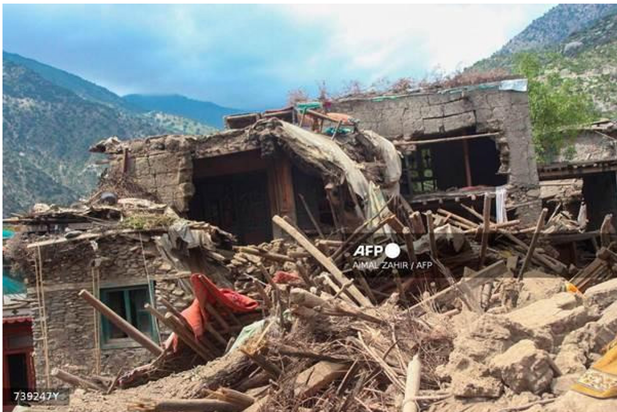
Figure 5.25: A damaged and tilted house situated on sloped terrain in Mazar Dara village, Nurgal district, Kunar province (Zahir, 2025)
