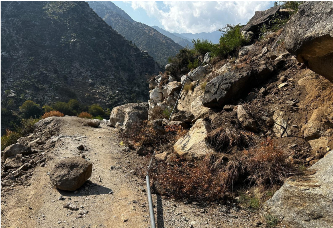
Figure 6.2: Example of damages to a water supply pipe due to rockfalls
