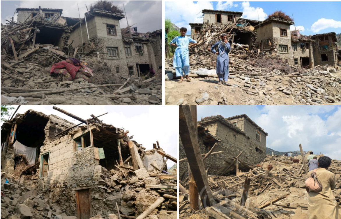
Figure B.4: Earthquake damaged buildings in Kunar with stone and cob walls
