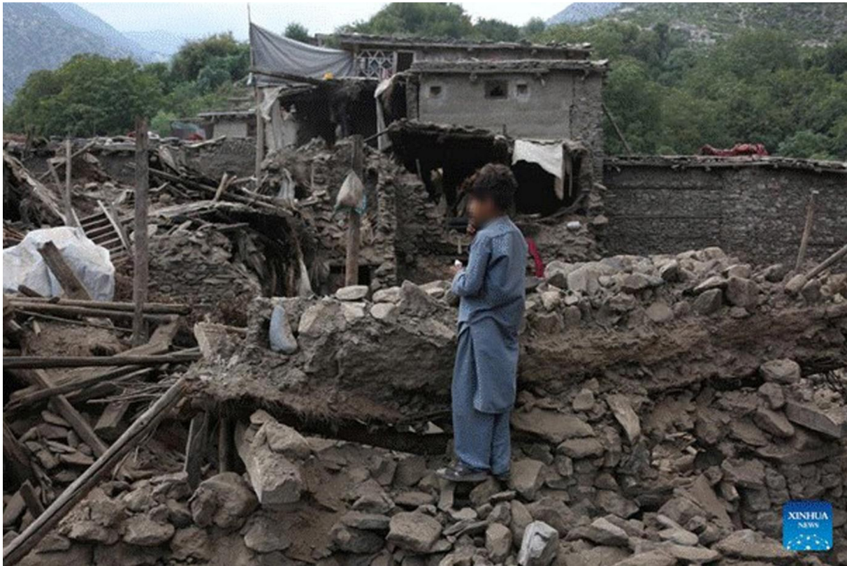
Figure 5.20: Unreinforced strip foundation of collapsed house at Nurgal district of Kunar province (Xinhua, 2025)
