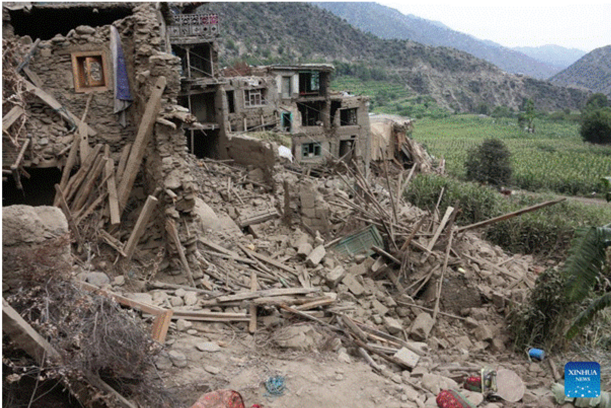
Figure 4.3: Houses built onto slopes damaged by differential movement at Nurgal district of Kunar province (Xinhua, 2025)
