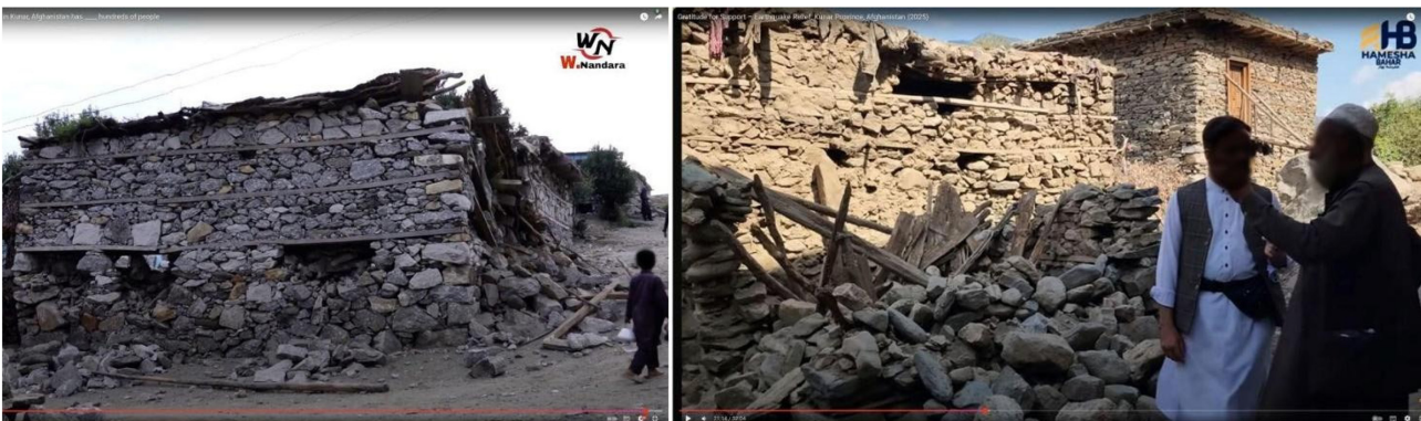
Figure 5.27: Stone/Timber connection. Left: YouTube, Watan Nandara channel https://tinyurl.com/yxnchrsb ; Right: Youtube, Hameshabahar Afghanistan channel https://tinyurl.com/3hwusksw
