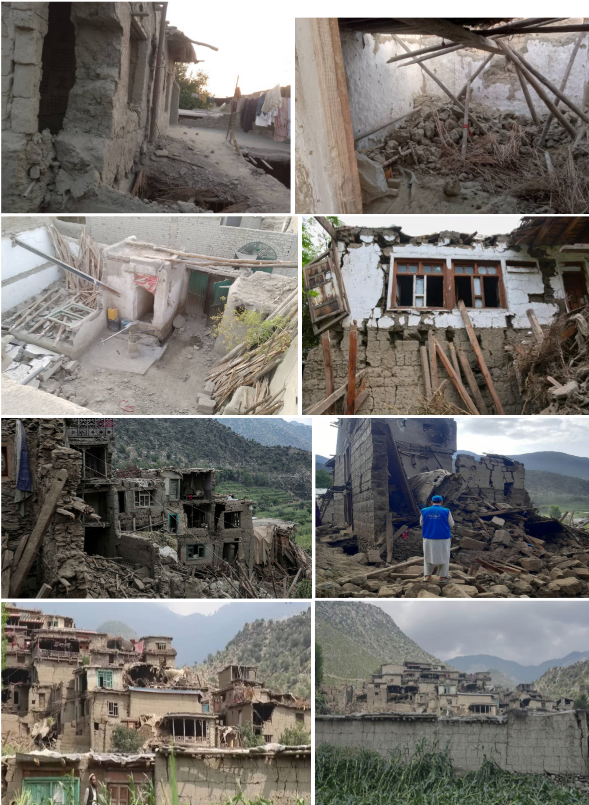
Figure B.5: Earthen structure affected by earthquake
