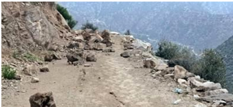
Figure 4.7: Rockfall blocking road access (Miyamoto International, 2025a)
