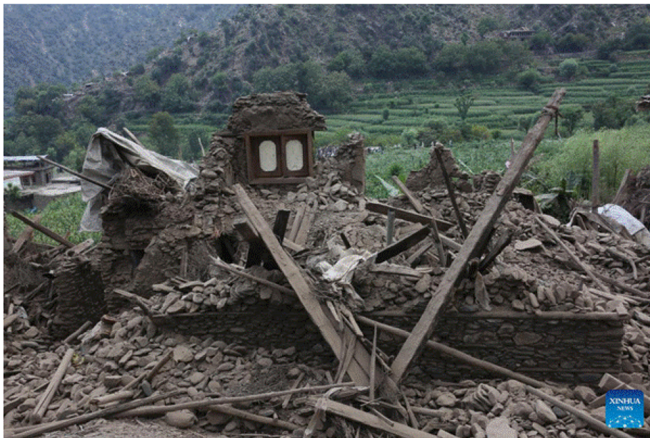
Figure 4.2: Complete collapse of unreinforced house at Nurgal district of Kunar province (Xinhua, 2025)
