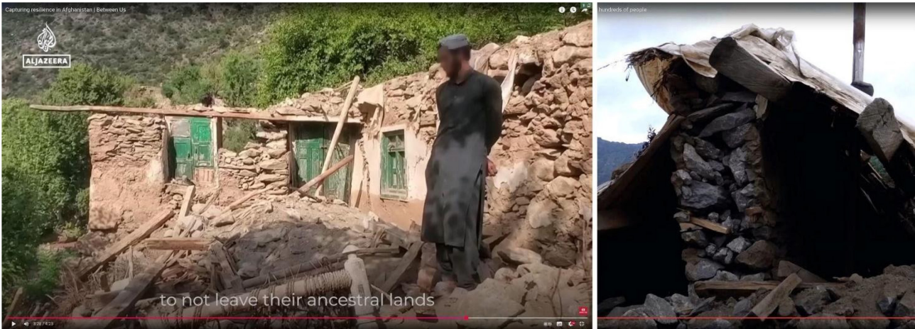
Figure 5.13: Wall coherence. Left: delamination (Credit: Youtube, Aljazeera English channel https://tinyurl.com/8bhbe5x6 ), Right: absence of through stone (Credit: YouTube, Watan Nandara channel https://tinyurl.com/yxnchrsb )
