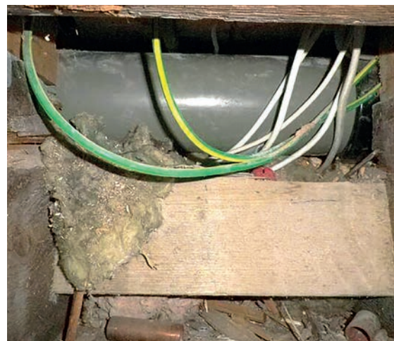
➤ FIGURE 2: Soil pipe passing through notched and unreinforced floor joist
