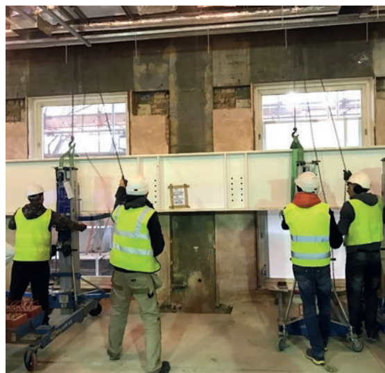
FIGURE 1: Refurbishment of existing structure can extend its use but may involve changes to load paths
